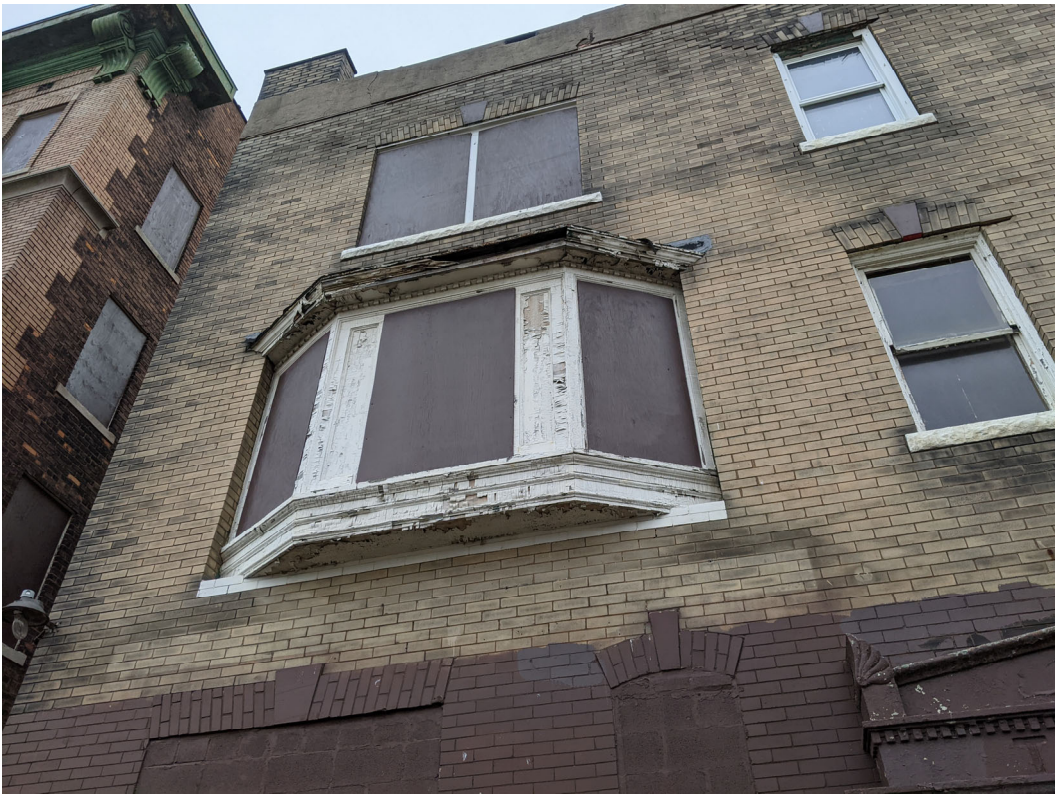
Detail view showing conditions at the Henry (primary) facade. The center (2 nd story) window is original. Staff photo, November 24, 2020.
