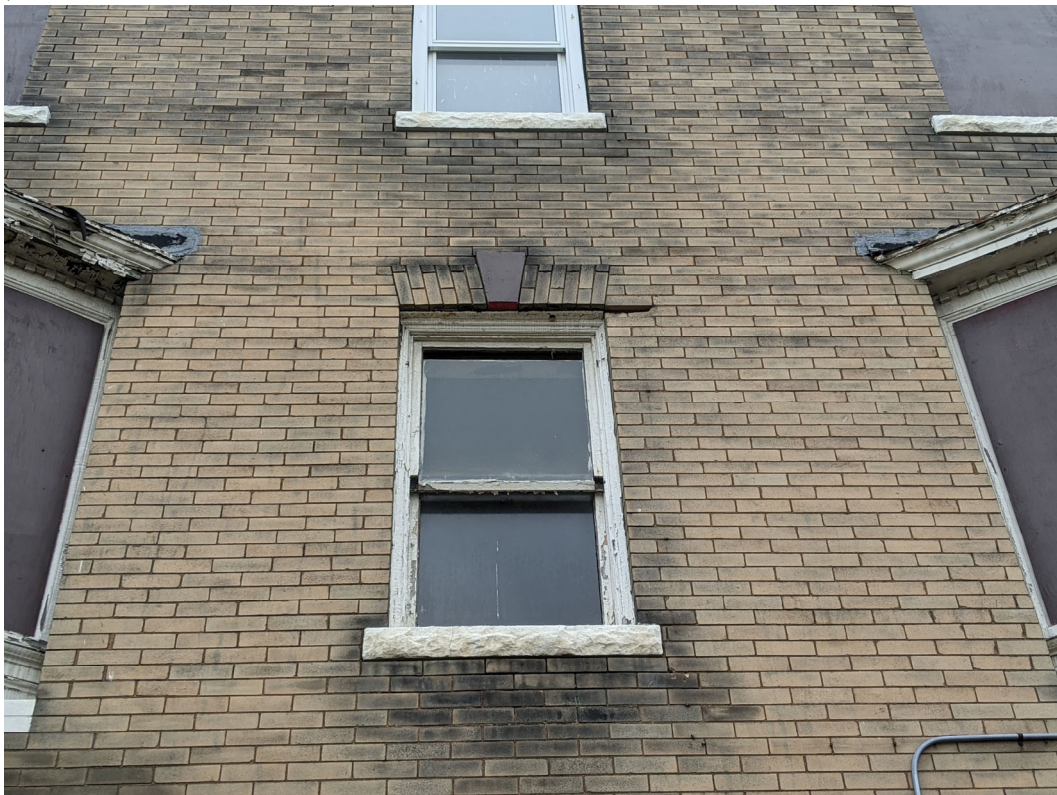
Detail view of an original wood window at the front elevation. Staff photo, December 7, 2020.
