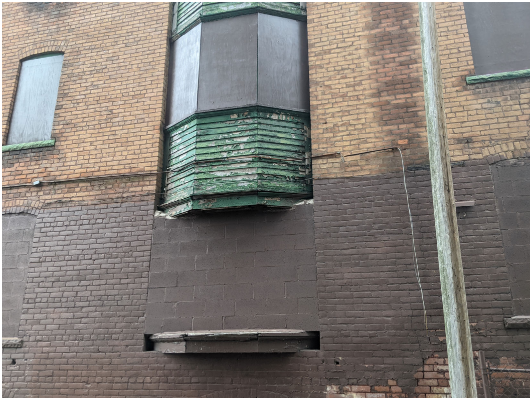
Detail view of west-facing bay at alley elevation. Note unusual clapboard detailing, and missing first story windows. Staff photo, December 7, 2020
