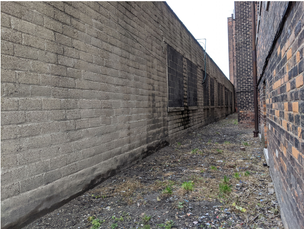
View of the concrete block east elevation, immediately adjacent to Bretton Hall. Note the large, blocked-in window openings. Staff photo, November 24, 2020.
