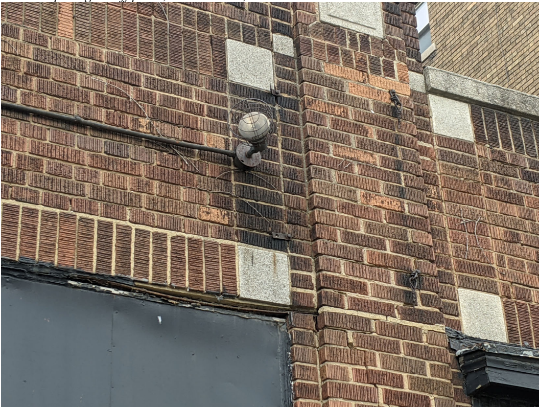
Detail view of brick/stonework and existing light fixtures at front facade. Staff photo, November 24, 2020.
