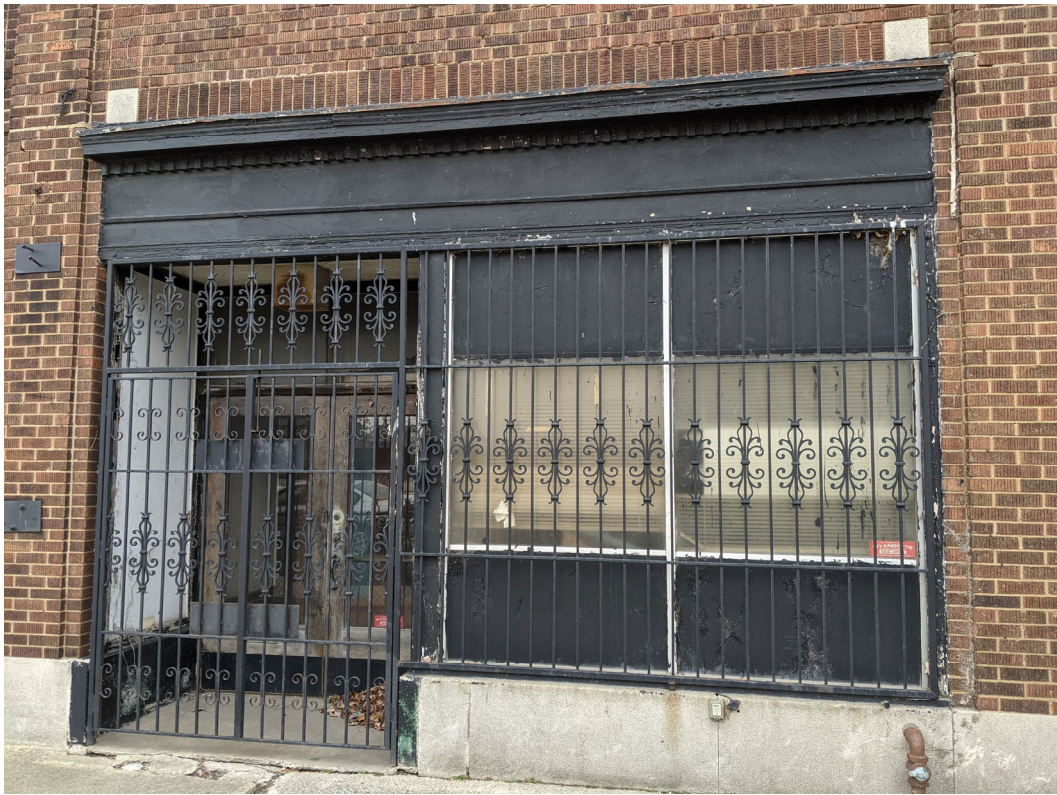
Detail view showing conditions at the westernmost storefront. Staff photo, November 24, 2020.
