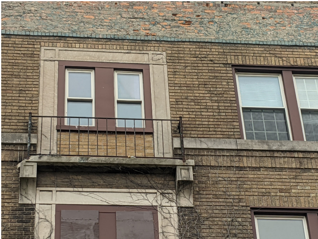
Detail view of altered balconette openings and cornice area above. Staff photo, December 7, 2020.
