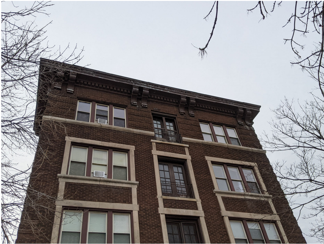
Detail view showing conditions at the Henry (primary) facade. Staff photo, November 24, 2020.
