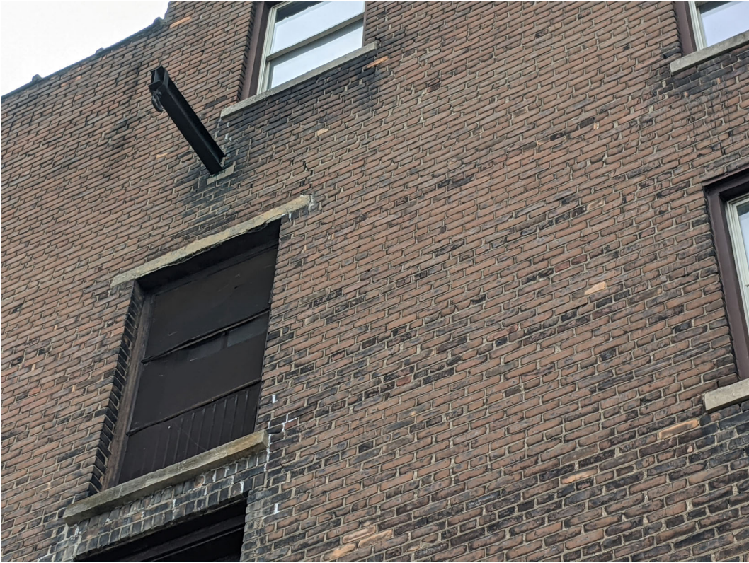
Detail view of brick and furniture hoist beam at top of rear elevation. Staff photo, December 7, 2020.
