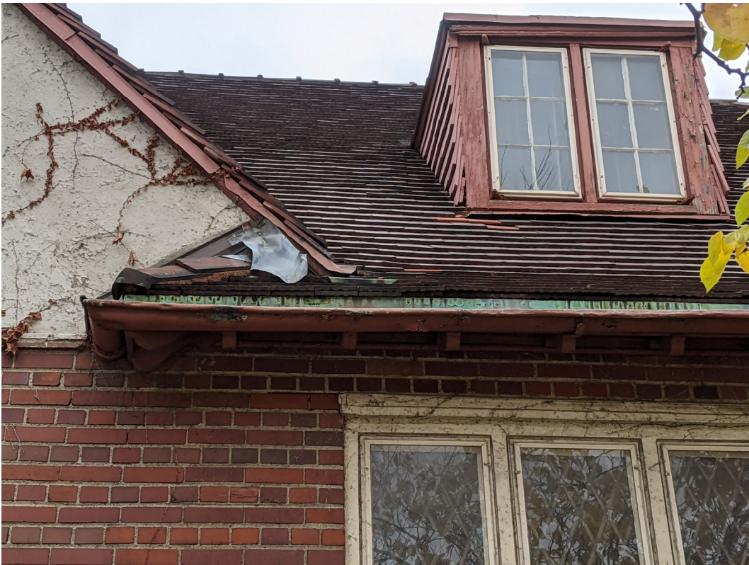
Detail view of roof along John R elevation. Note visible copper and indentations at edge of gutter. Staff photo, October 30, 2020.
