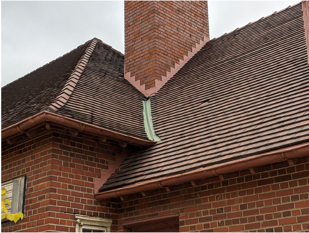
Detail view of roof as seen from John R. Note copper flashing and wear/tear on gutters consistent with a soft metal. Staff photo, October 30, 2020.
