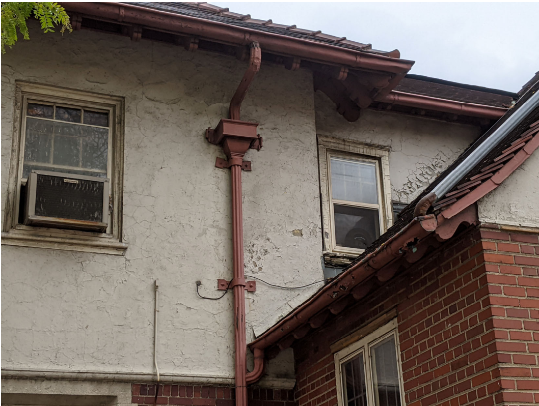
Detail view of roof and ornamental downspout system. Note also the radiused elbow bend at bottom. Staff photo, October 30, 2020.
