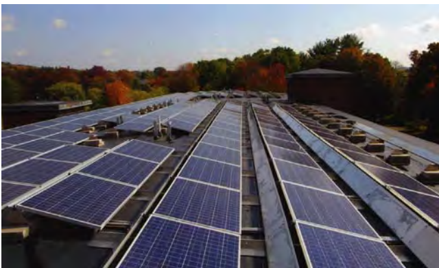
Solar panels installed on the flat roof.
