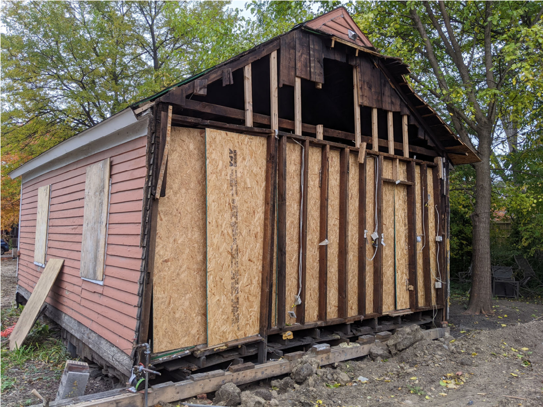
Rear view of 2221 Wabash, showing partial demolition already undertaken per the Commission’s previous approval. Staff photo, October 30, 2020.
