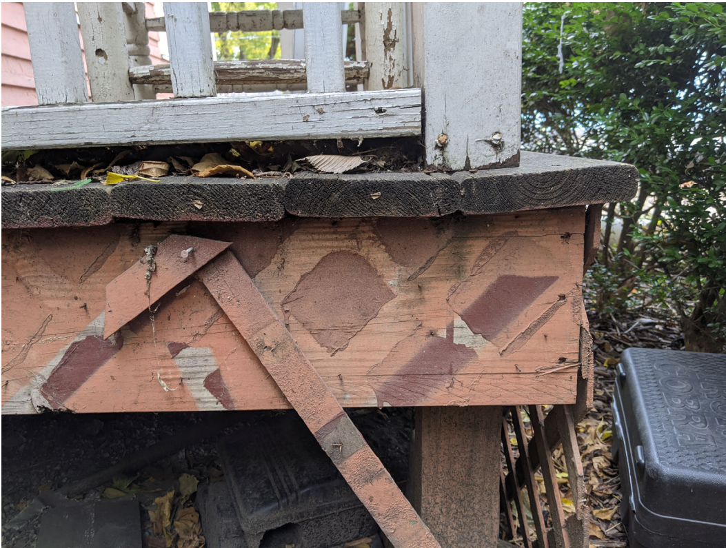
Detail view of front porch. Modern pressure-treated products and a single coat of paint confirm not historic age. Staff photo, October 30, 2020.
