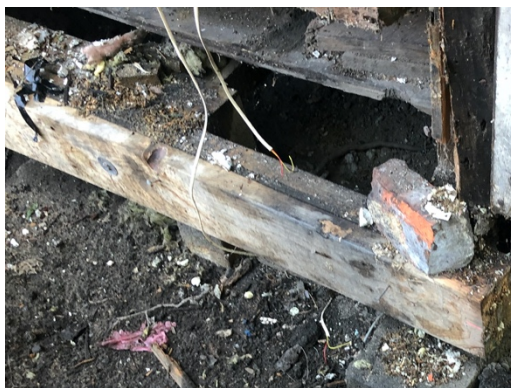
P7: Floor Structure Deterioration
