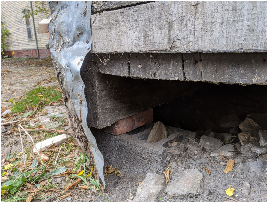
Detail view of "foundation" under front facade. While the heavy timber appears of historic-age, clearly the brick and concrete block were later alterations, probably to a deteriorated wood foundation pile. Staff photo, October 30, 2020.
