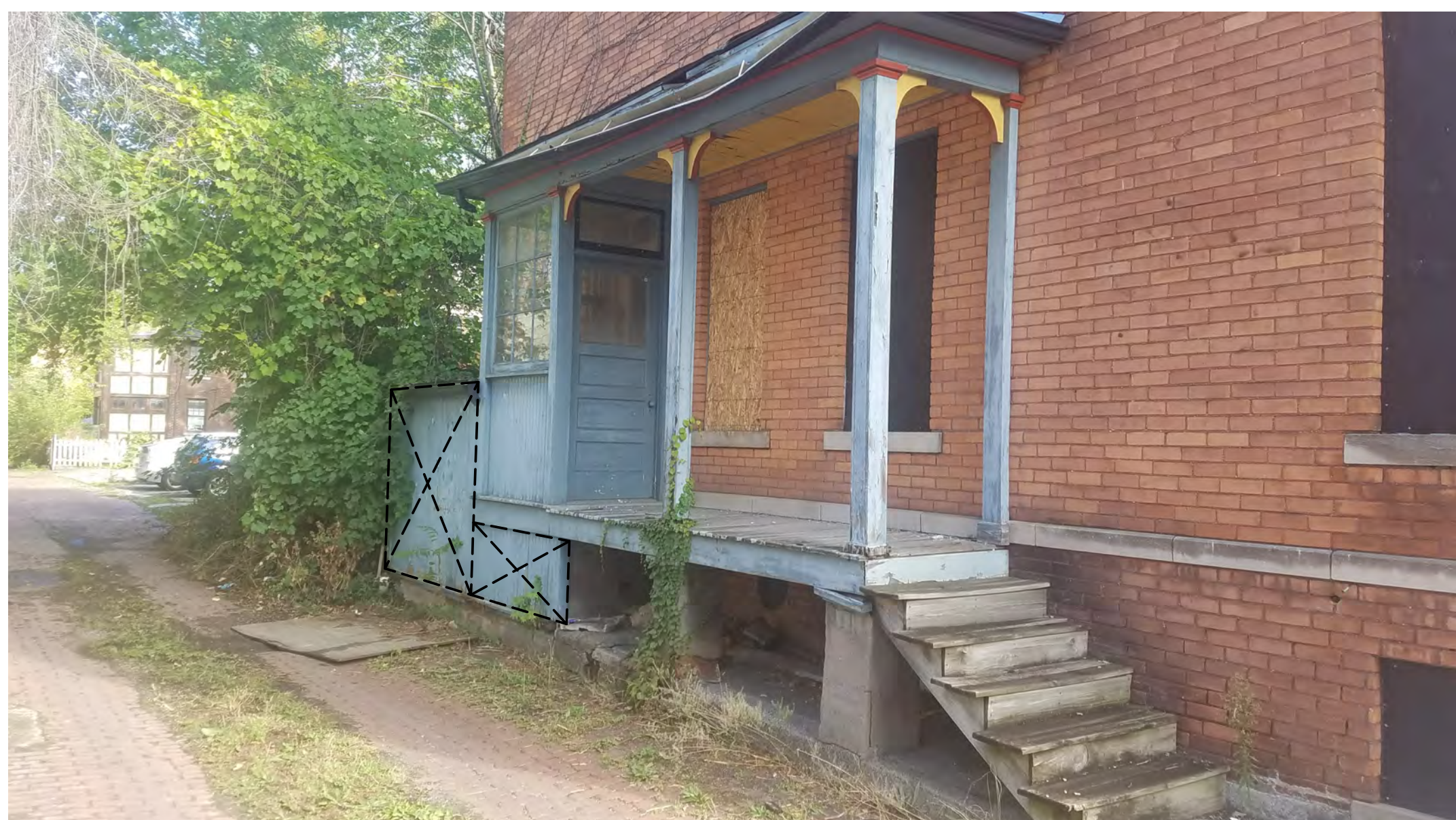
EXISTING PORCH AND BASEMENT STAIR ENCLOSURE (IDENTICAL ON BOTH SIDES OF THE BUILDING)
