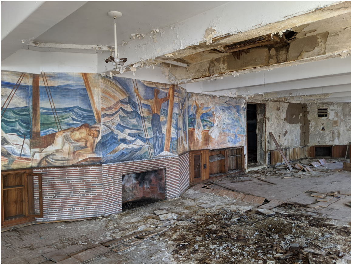
General view of the wardroom and portions of the Fredenthal mural, with water damage towards rear (east). Staff photo, 2/14/2020.
