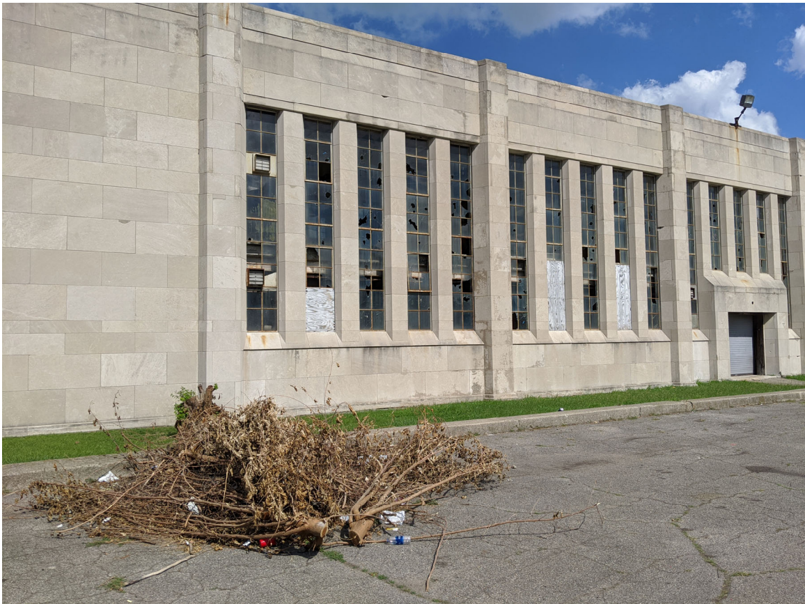
View of East Elevation (north block), showing broken windows and apparent dumping on site. Staff photo, 8/7/2020.
