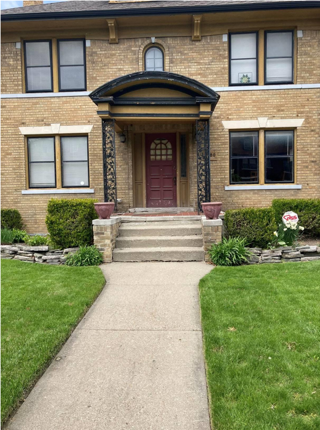
Applicant Photo – Shows porch before columns were removed and temporary supports put in place
