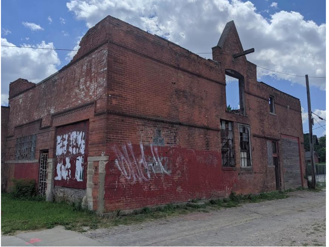
Carriage house. Note. East elevation gable has collapsed
