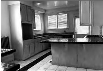
BEFORE: The kitchen of the house Jeff Cowin bought, renovated, and lives in had buckled counters and uneven floors.
