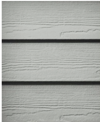
SIDING James Hardie Cement Board COLOR B:14 Dark Grayish, Olive MS: 10Y 2/2, Color System E, to match house.
