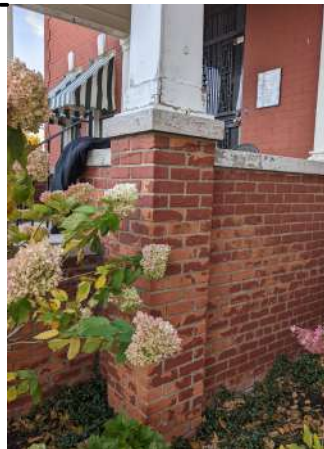
EXISTING COLUMN BASE SPALLING MASONRY PAINT
