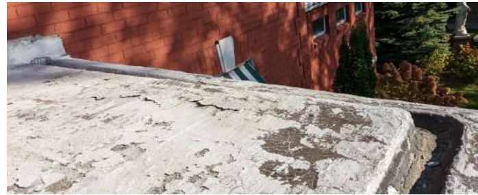
MULTIPLE LAYERS OF DECAYED ROOFING, LEAKING INTEGRAL GUTTER, INADEQUATE GUTTER DEPTH, DECAYED WALL COUNTERFLASH
