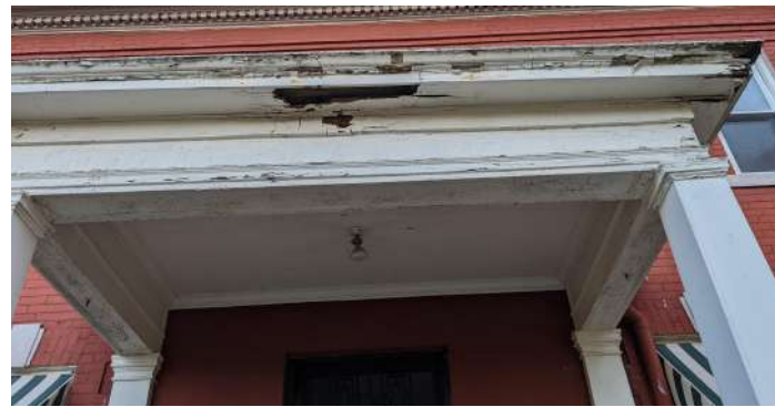
MODIFIED OVERHANGS WITH DECAYED SOFFITS AND FASCIA, EXISTING PORCH CEILING AND LIGHT
