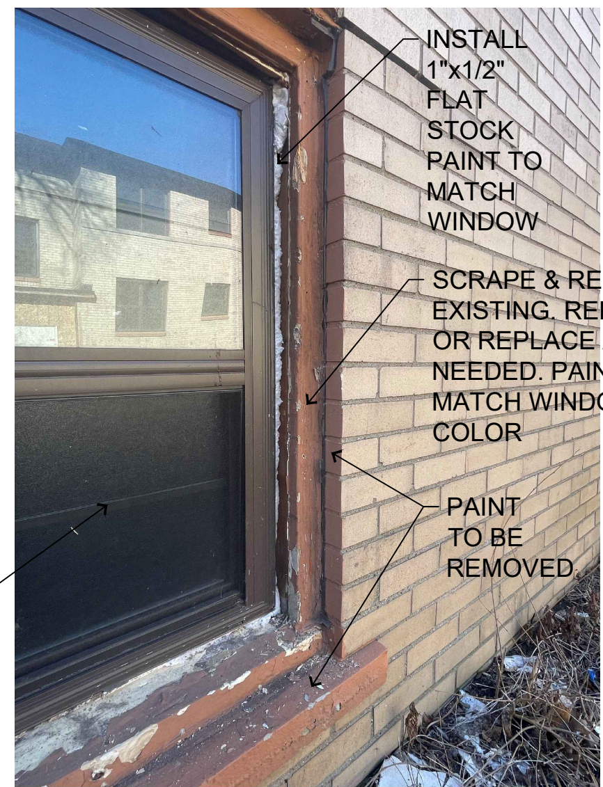
window with metal removed (bottom right view)
