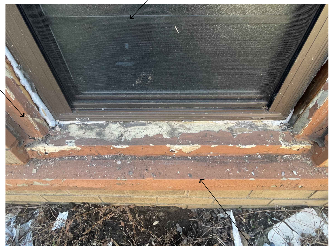
window with metal removed (bottom stool view)
