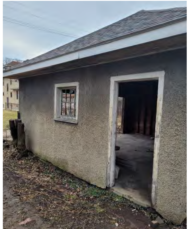
Site photo 3, by Applicant showing garage at the rear of the property with new asphalt roof (work completed without approval).
