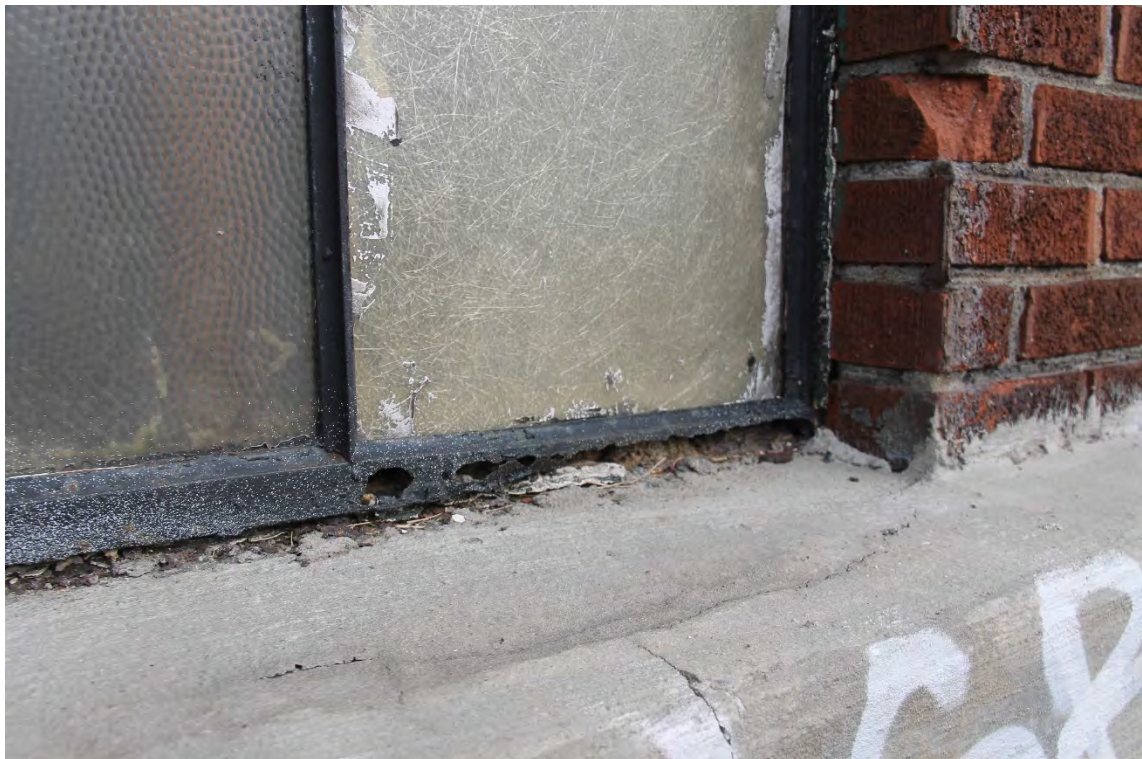
Typical Bottom Rail Condition, Exterior View
