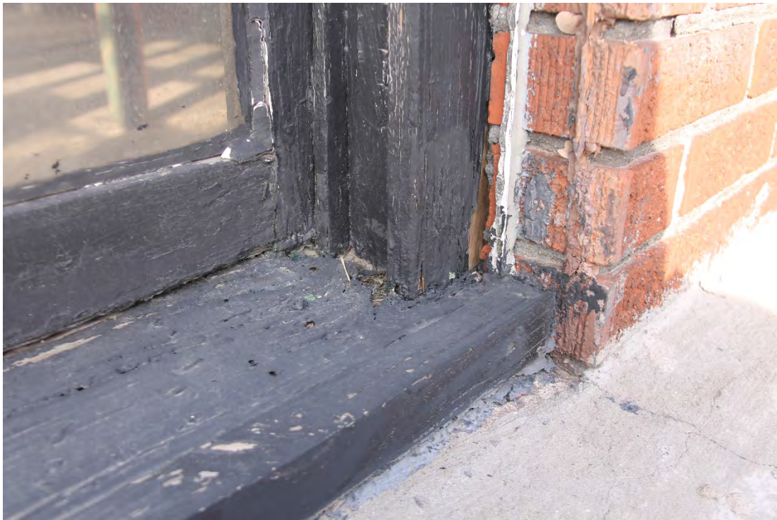
Exterior View of Failed Sill; Completely Rotted Through with Paint Covering. Example of 2x2 Added to All Windows Covering Rotten Sill, As Well As Missing Brick Mould.
