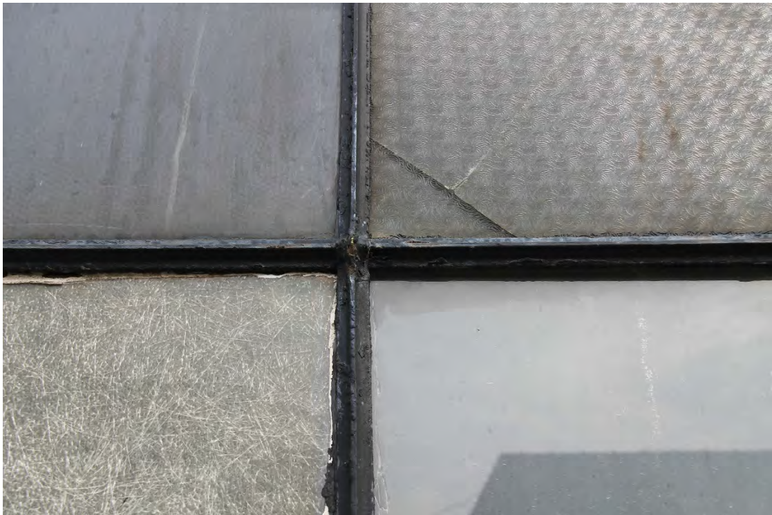
Typical Muntin Original Steel Window and Example of Four Types of Glazing Existing
