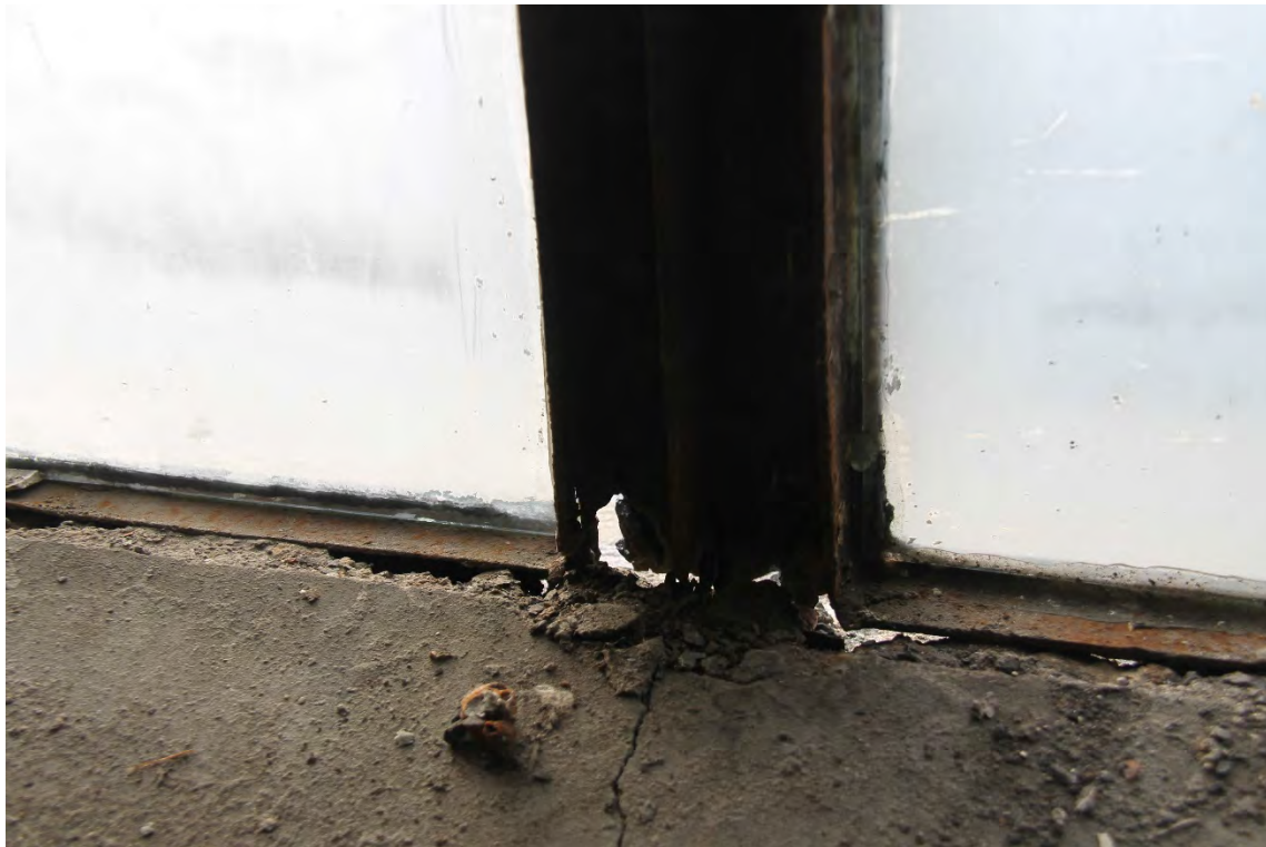
Mullion Condition of Existing Steel Window, Interior View
