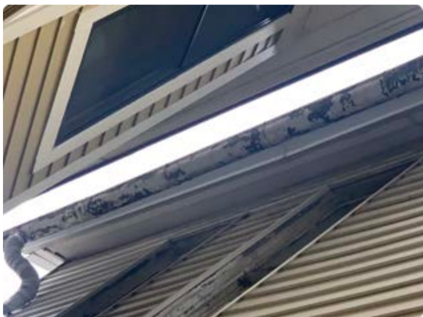
Rotted gutter on the side of home side view from front left.
