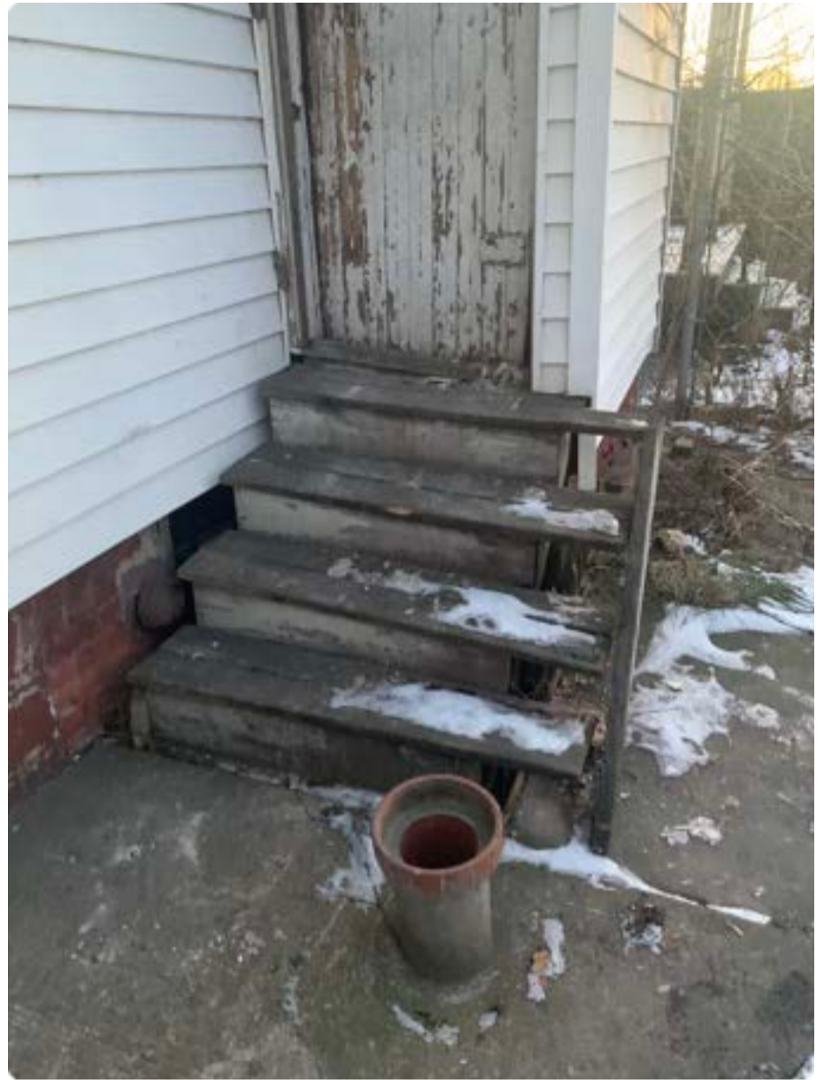
Exterior rotted back steps & old clean out vent
