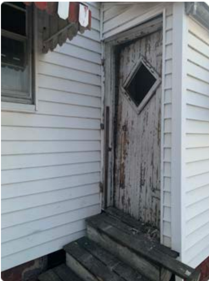
Exterior rotted back porch door
