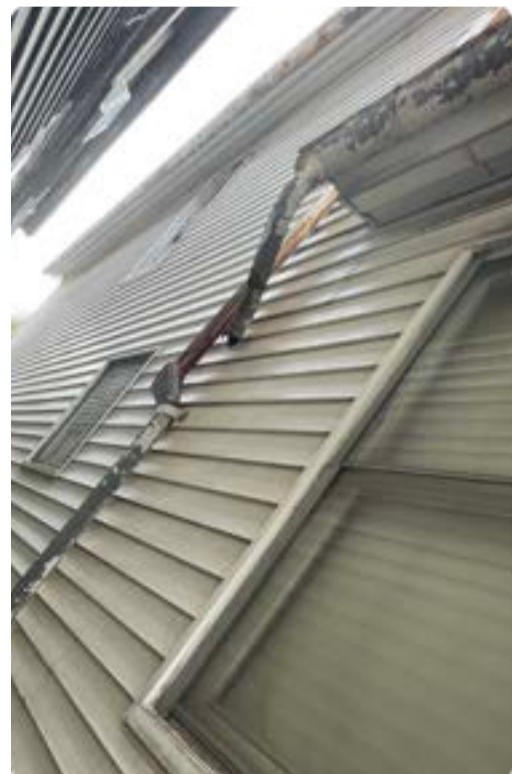
Rotted and broken gutter
