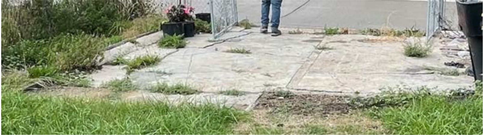
Broken cement garage pad
