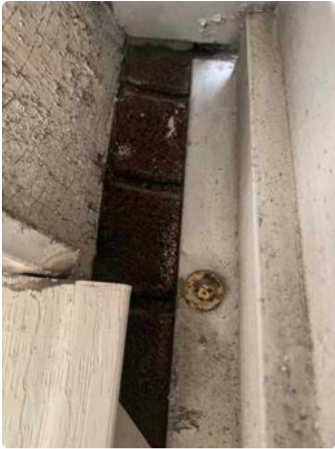
Exposed portion of Red Asbestos Overlay
