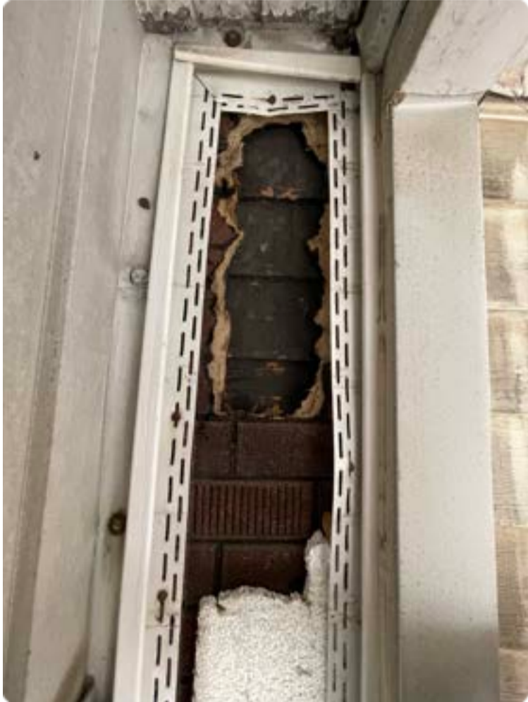
Current layers of exterior cladding: ( Vinyl siding, Styrofoam, Insulbrick, Original wood front left corner)
