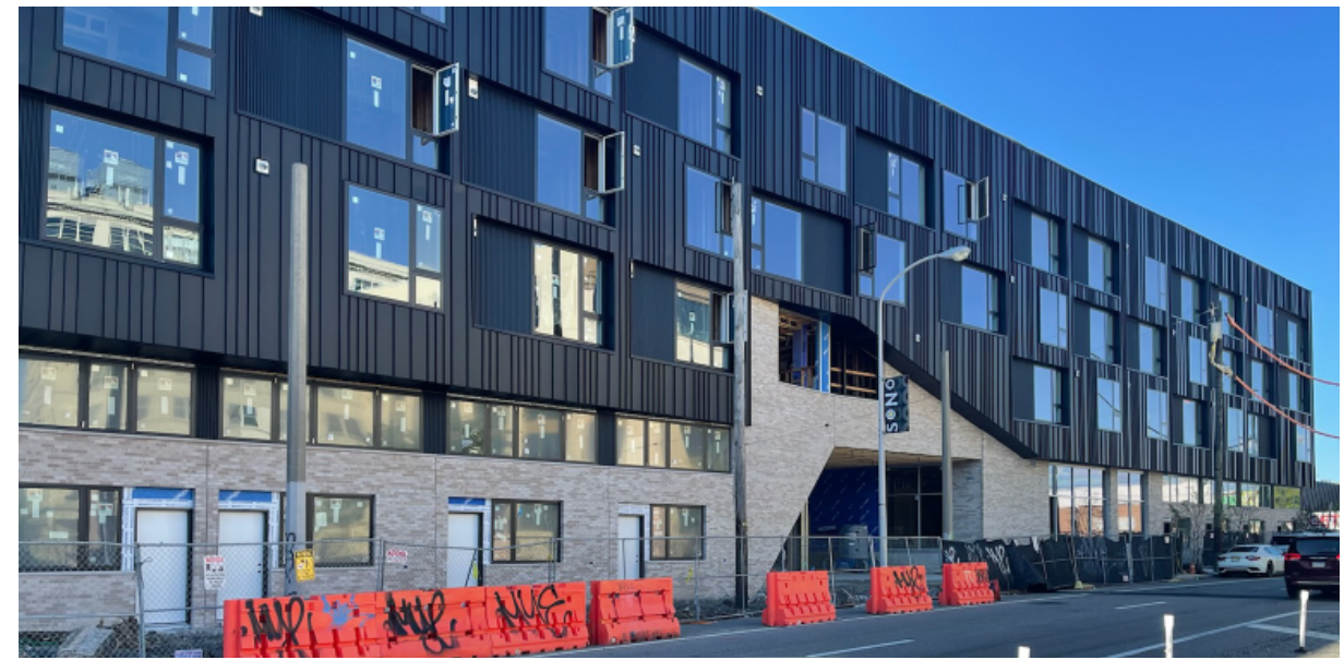
STANDING SEAM PROFILE IDENTICAL TO CMG PRODUCT VARIABLE WIDTHS (16" TO 8") - NO STIFFENING RIBS SONO, PHILADELPHIA (IN PROGRESS)
