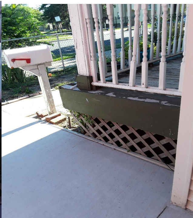
Porch is falling into the ground.
