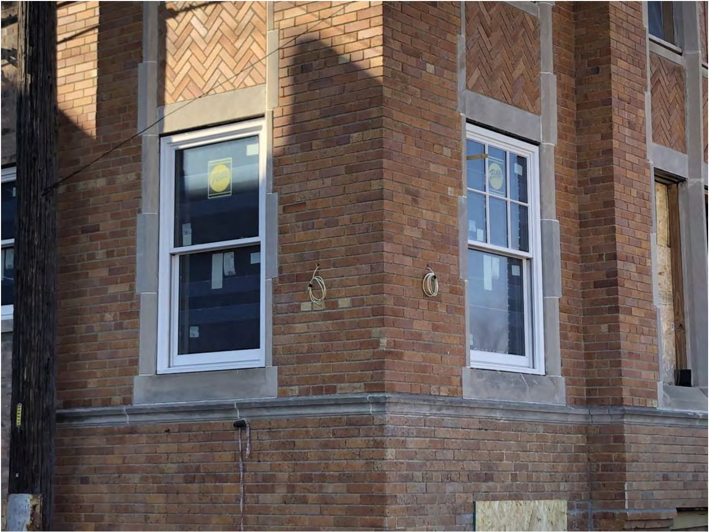
The window on the left, staff believes, should have a six-over-one pattern.
