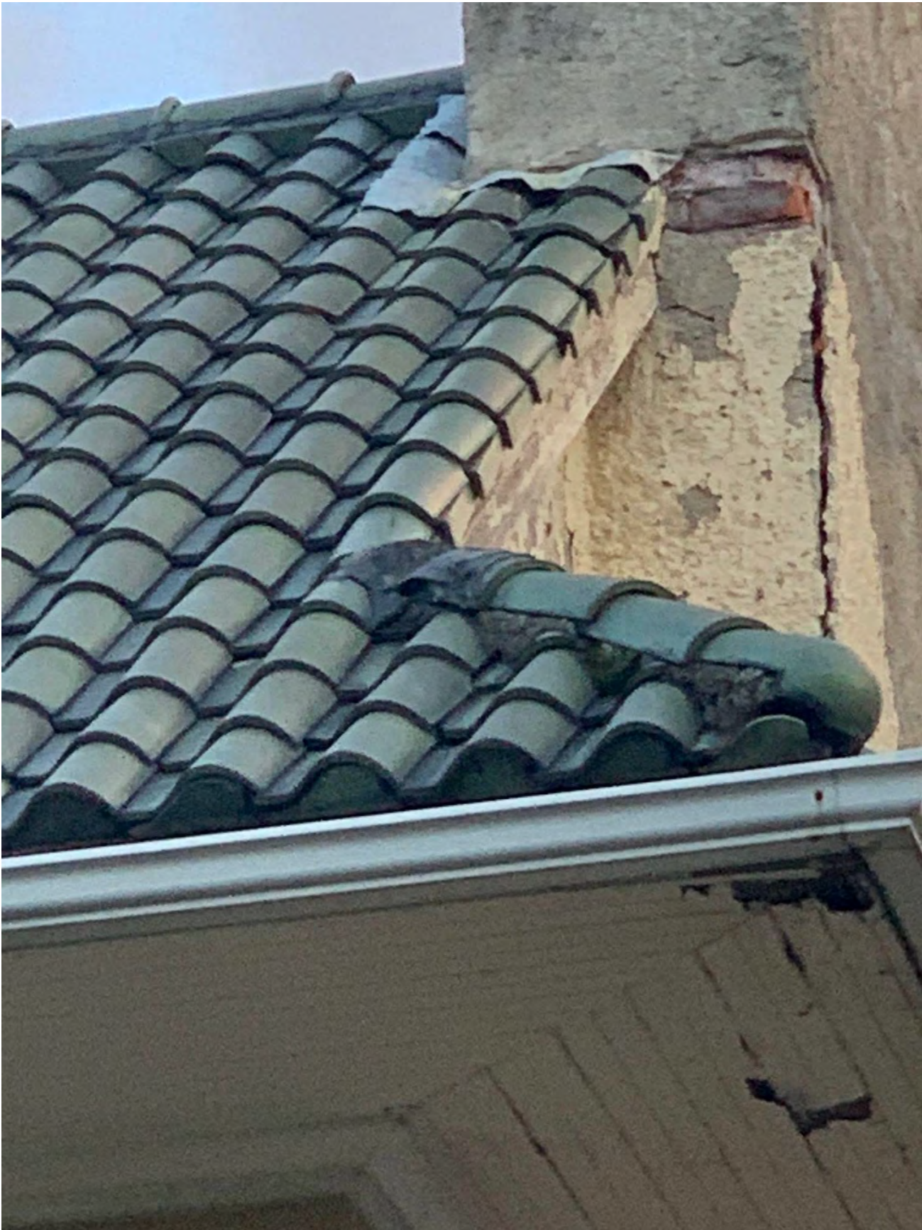
Missing Tile Detail 3 9-10
