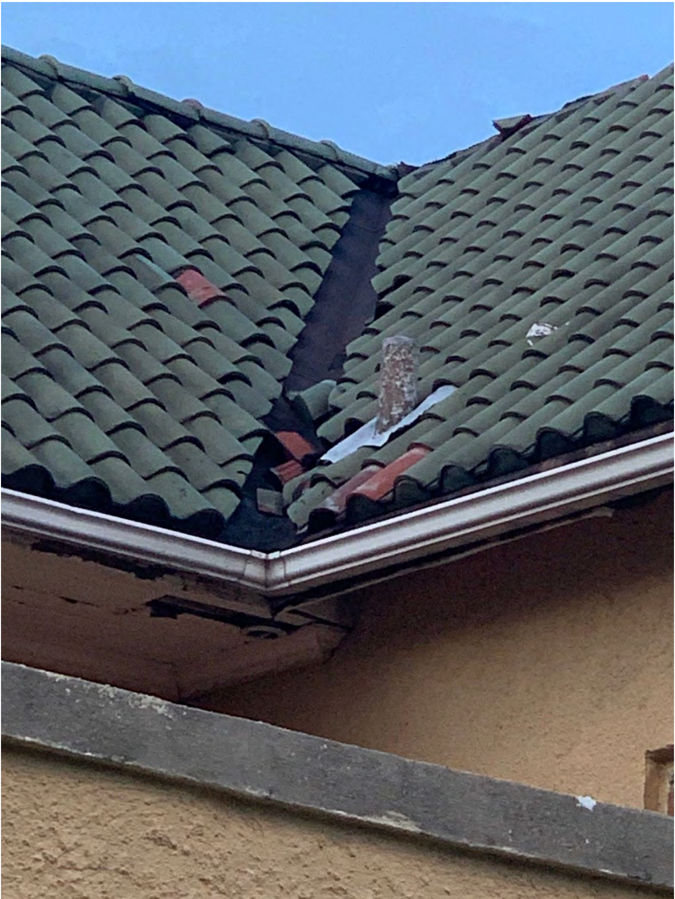
Missing Tile Detail2 9-10
