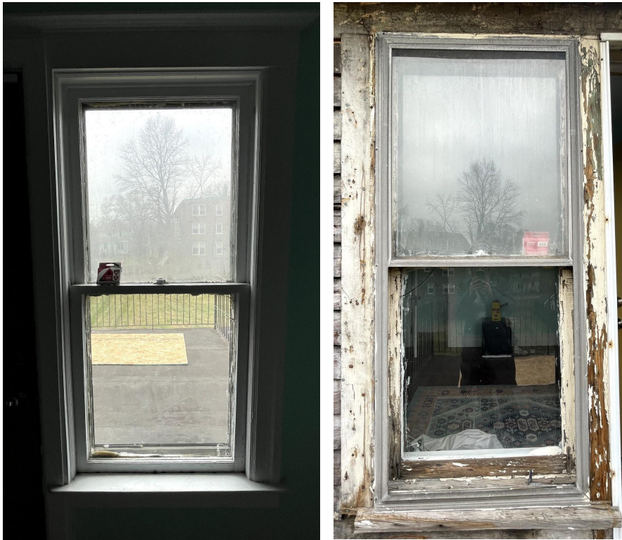
Window U, 55" x 28.5" Wood, inoperable, rotted sash and sill. These two windows sit on the West side of the house and have no protection (trees, buildings, etc.) from weather elements. Additional photos on next page
