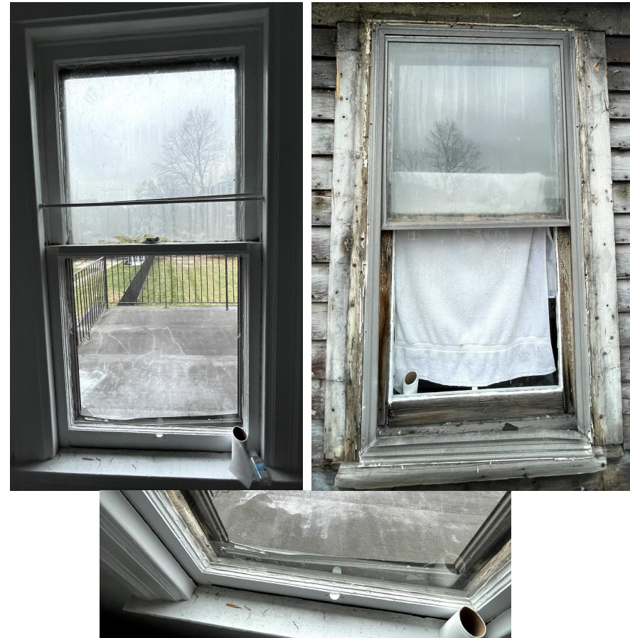
Window V, 61.5" x 29" Wood, inoperable, warped storm window, rotted sash and sill.
