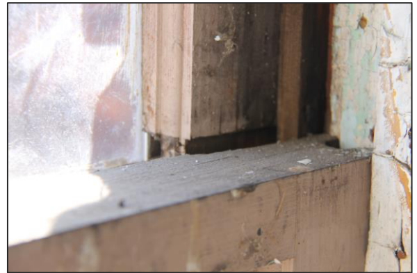
Failed Sash Joinery
