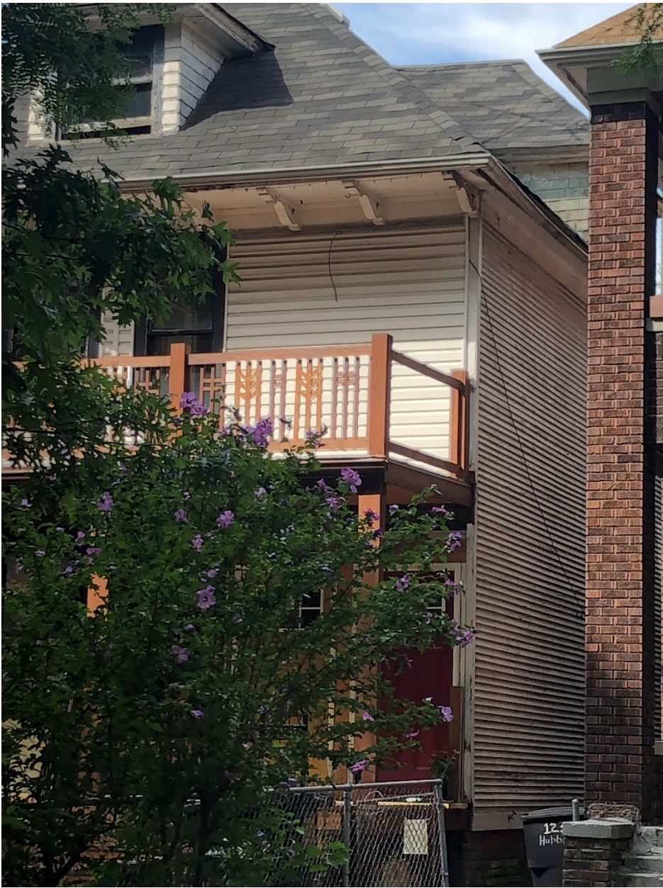
Here you see the transition from the vinyl siding to the historic narrow clapboard siding.
