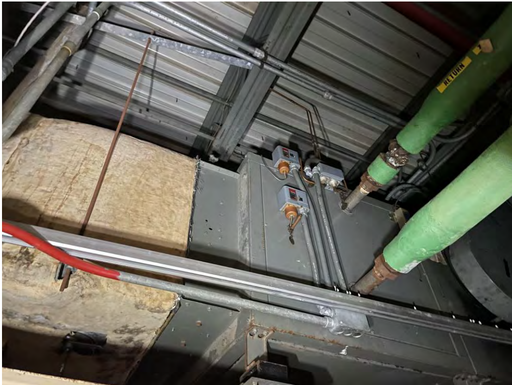
Old HVAC unit
