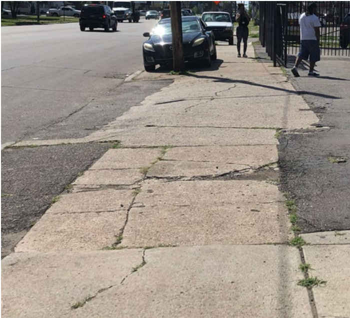
BROKEN, OBSTRUCTED SIDEWALKS
