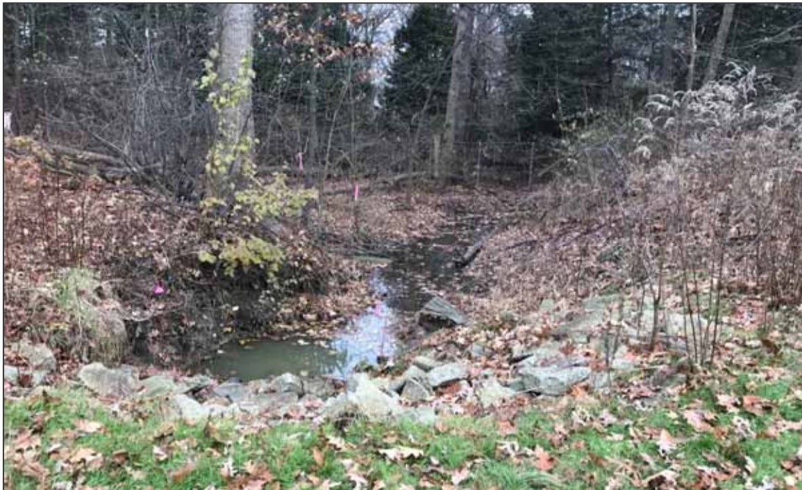
PHOTO NO. 20: View of the drain outflow located on the southern portion of the eastern parcel.
