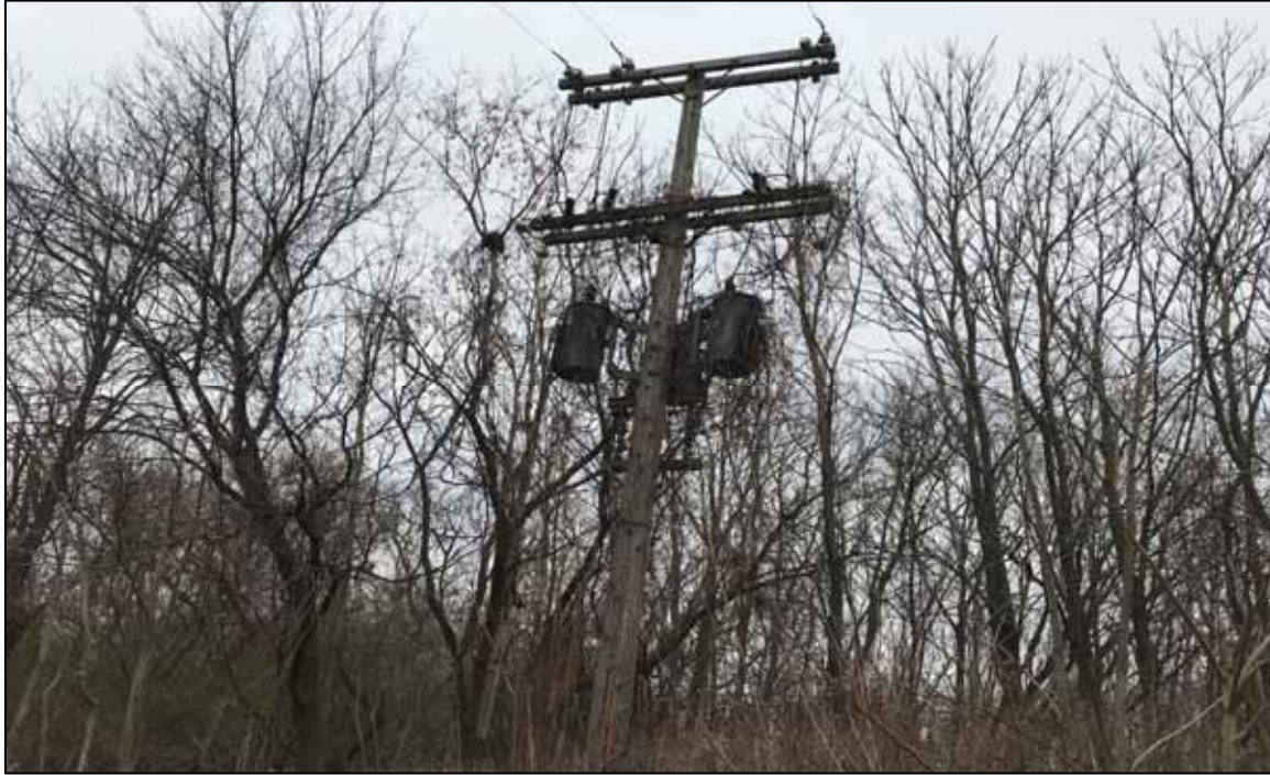
PHOTO NO. 13: View of three pole-mounted transformers located northwest of the irrigation well pump house.
