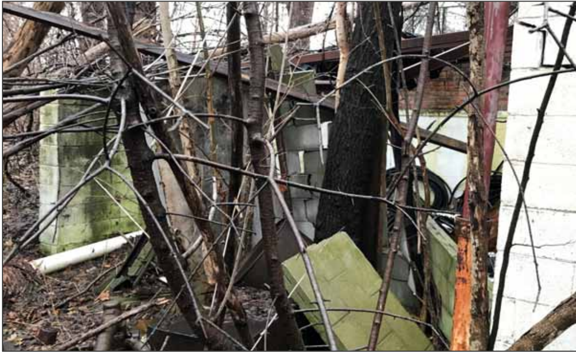
PHOTO NO. 35: View of the northern portion of the refrigeration house, with roof collapse and debris.
