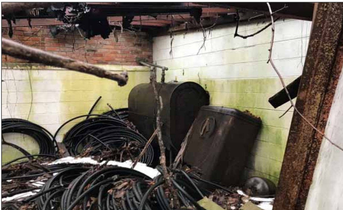
PHOTO NO. 36: View of the abandoned heating oil AST observed in the northern portion of the refrigeration house.
