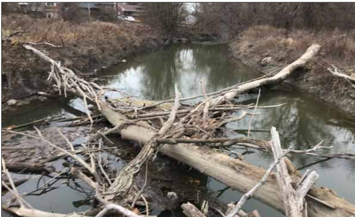
PHOTO NO. 28: View of the log jam observed at the bridge over the Rouge River, south of the clubhouse.
