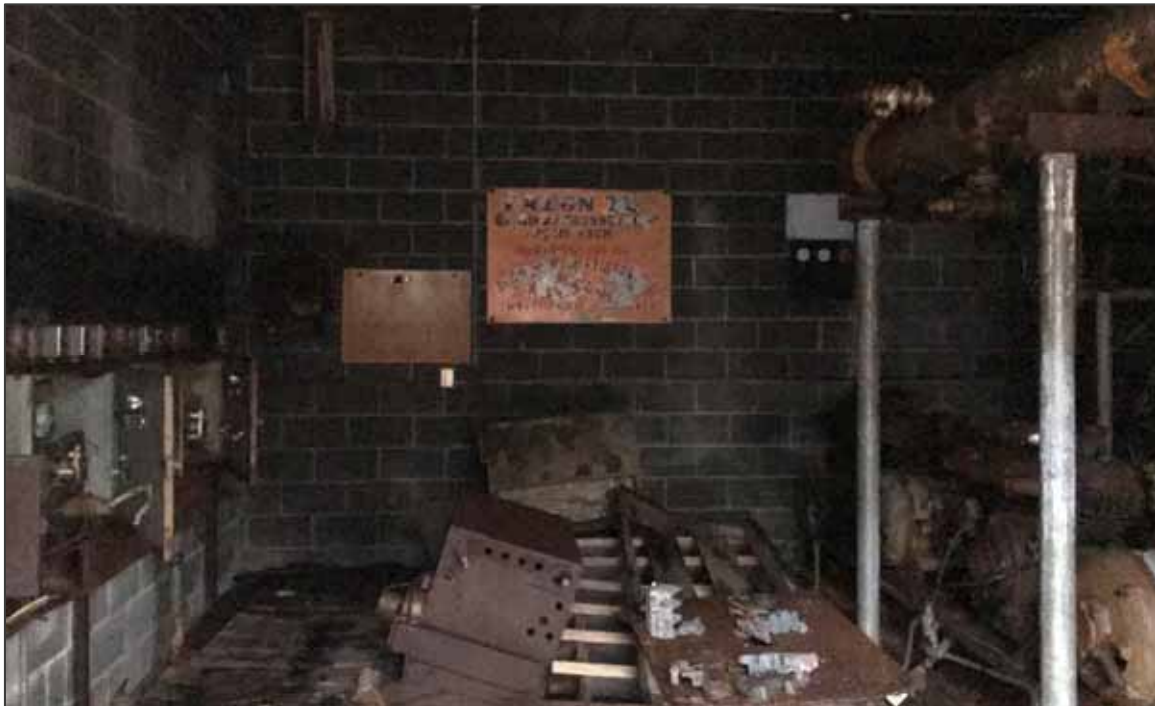
PHOTO NO. 34: View of the sign identifying Freon 22 as refrigerant in the refrigeration system.
