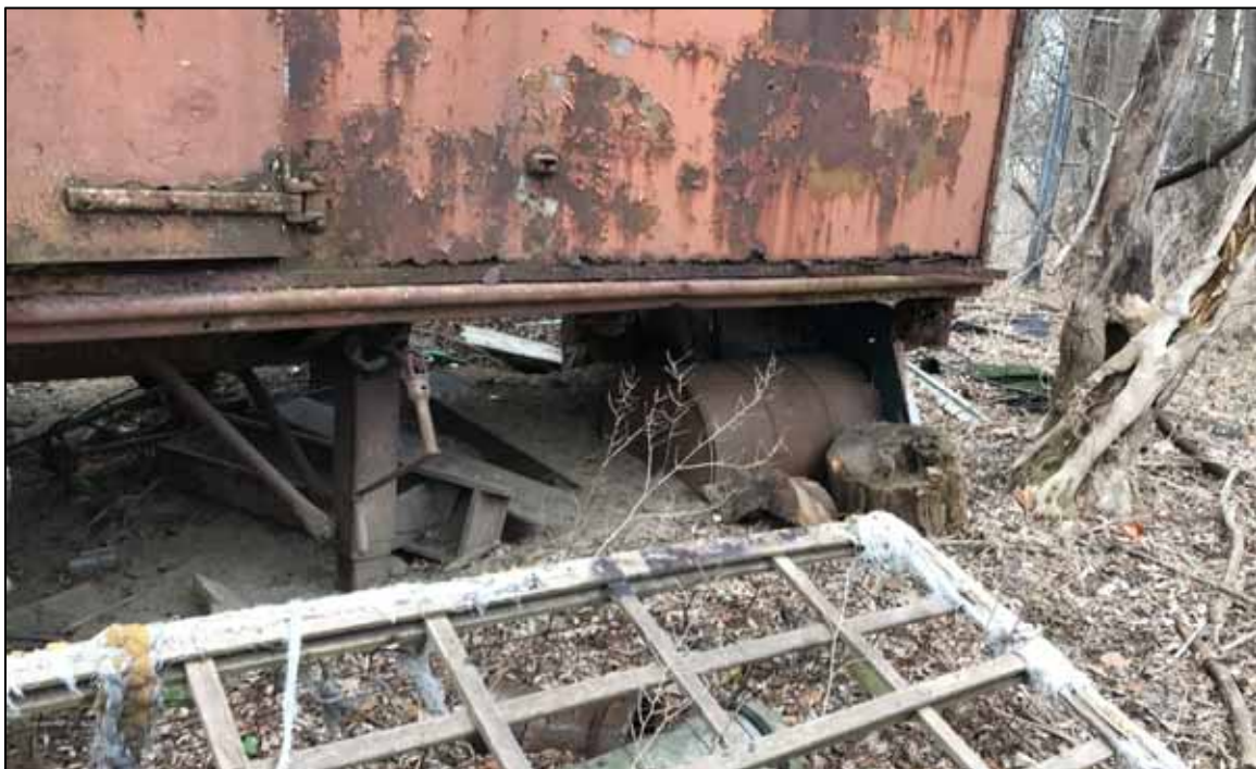
PHOTO NO. 8: View of a partially buried drum with no label beneath the semi-trailer.
