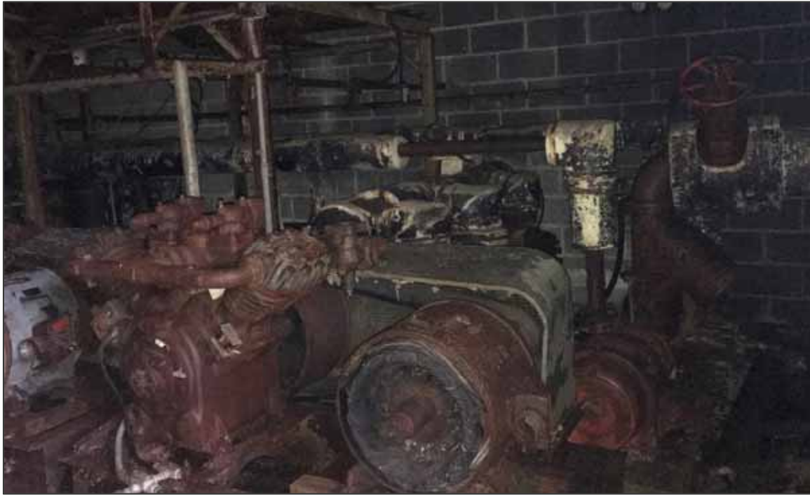
PHOTO NO. 33: View of the refrigeration system in the refrigeration house.
