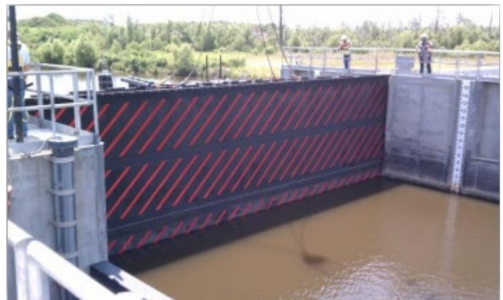
Figure 16: Stop log closure across Hero Canal, New Orleans, LA
