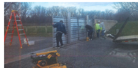
Example of stop logs being placed (Lawton Park, Fort Wayne, Indiana)
