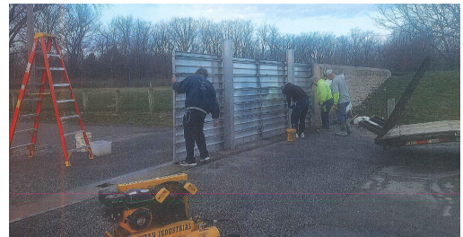
Example of stop logs being placed (Lawton Park, Fort Wayne, Indiana)
