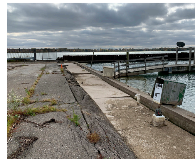
Uneven and broken pavement at the marina’s eastern parking area
