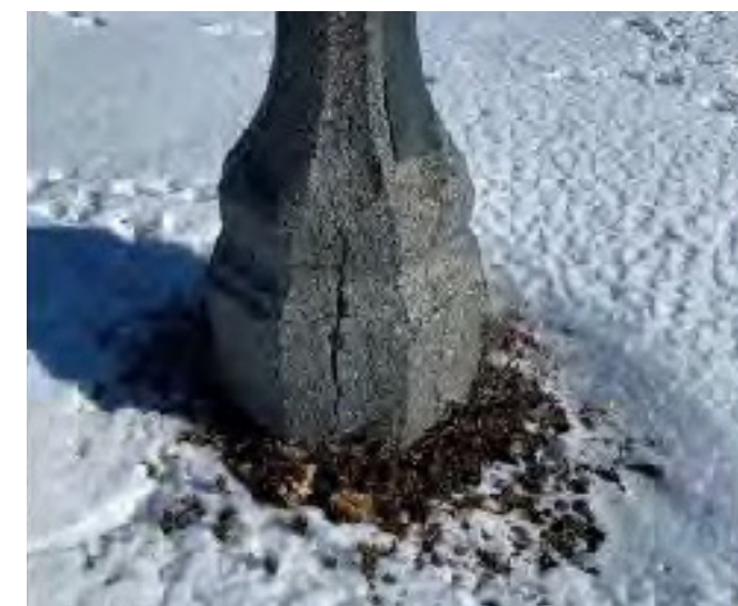
Precast concrete lighting fixtures with vertical cracking
