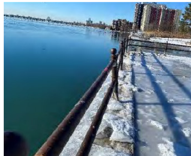
Existing concrete and steel sheet pile wall, leaning railing sections and flooding noted
