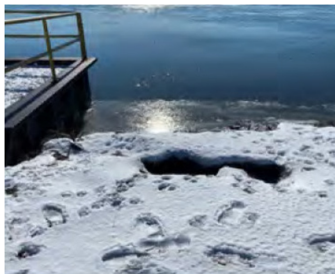
Unformed concrete poured along portions of shoreline is undermined
