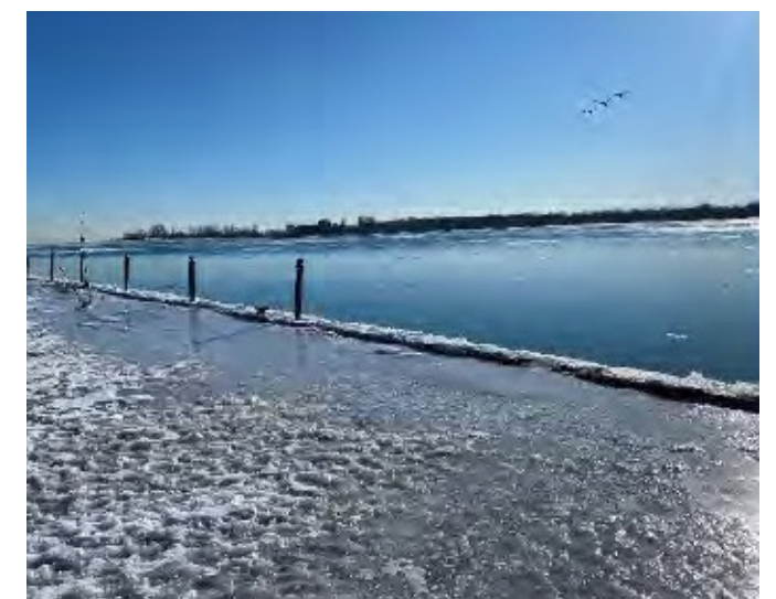
Approximately 70’ of missing railing and damaged posts
