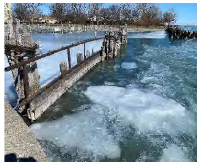
Timber pile and steel components noted to be in poor condition for breakwall at riverside entrance
