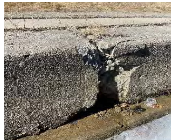
Concrete seawall shows deterioration to top of wall section requiring maintenance
