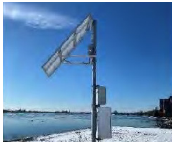
Solar panel system
