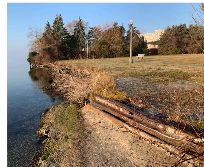
Unprotected shoreline with notable erosion
