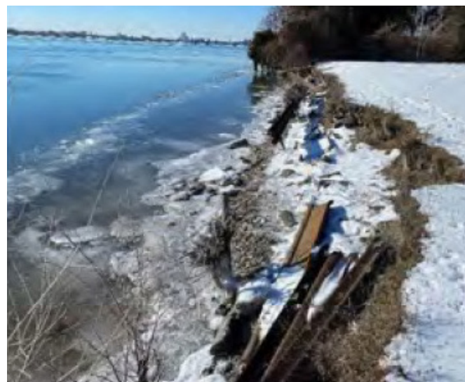
Guardrail section along shoreline is damaged and portions are missing, a potential hazard
