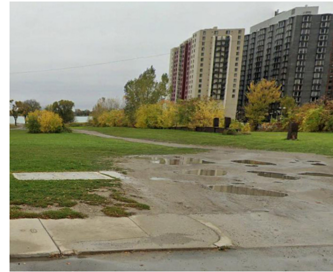
Dirt path in poor condition, used by vehicles to access the waterfront
