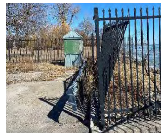
Approximately 40’ of fence is in need of repair
