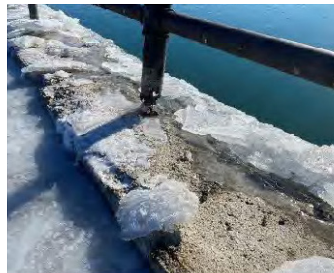
Broken post at railing
