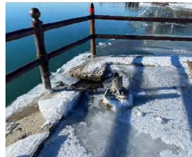
Damaged and missing light pole
