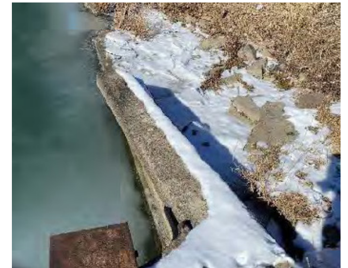
Noted deterioration of concrete seawall
