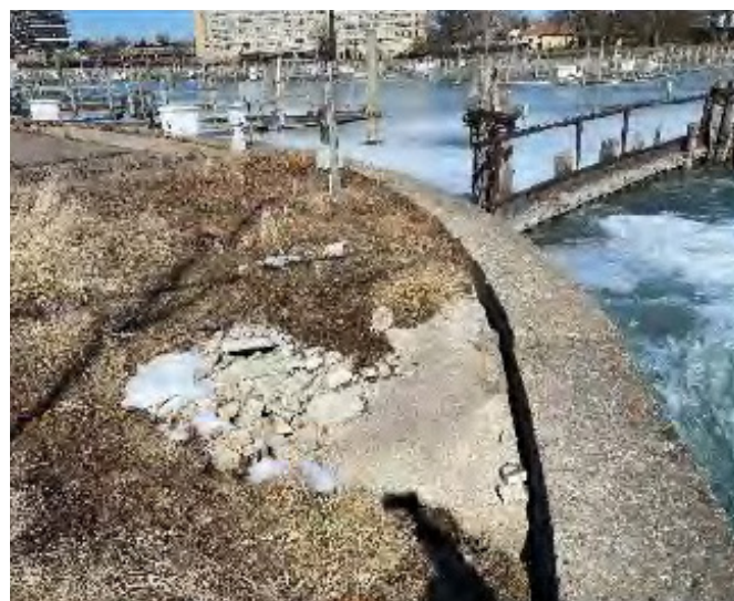
Concrete seawall in fair condition; separation in wall segments causing material loss from behind wall
