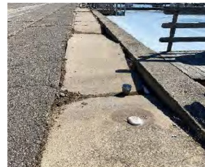
Significant settlement behind wall causing concrete walk to be uneven and potentially hazardous
