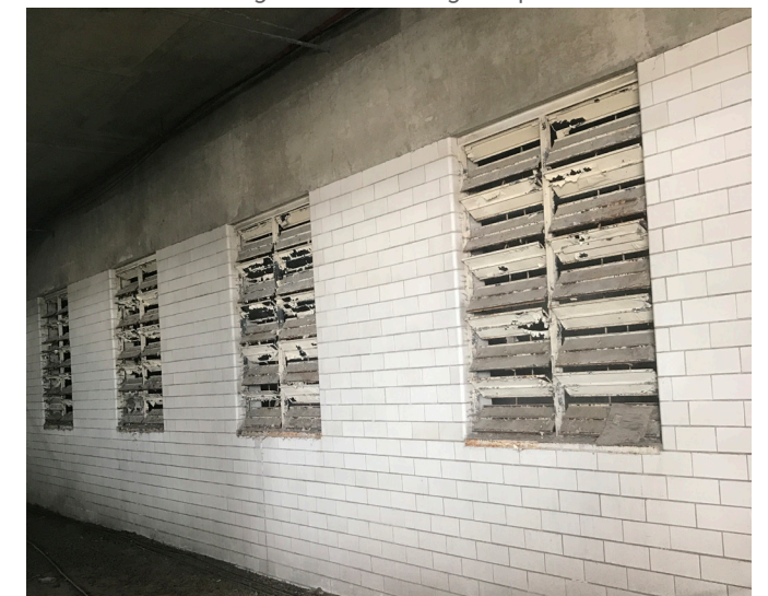
Damaged air vents in the lower level
