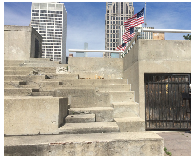
The mass concrete structure (Pyramid) is in poor condition and poses a safety hazard
