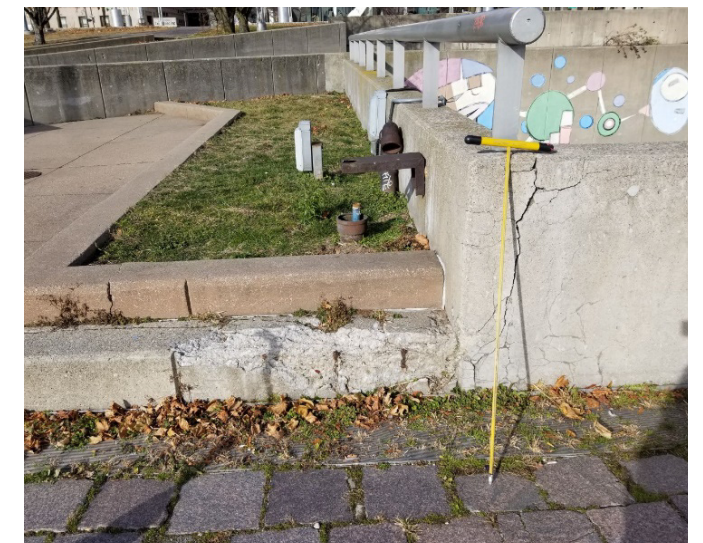
Fire and water damage to outside masonry wall in recessed area. Significant damage to painted surfaces
