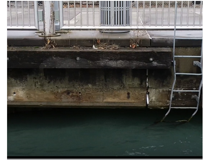
Seawall was found to be in fair condition with noted deficiencies.
