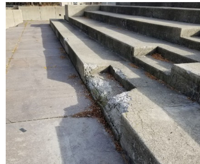
Concrete Step with numerous concrete deficiencies at walkway locations and concrete seating location
