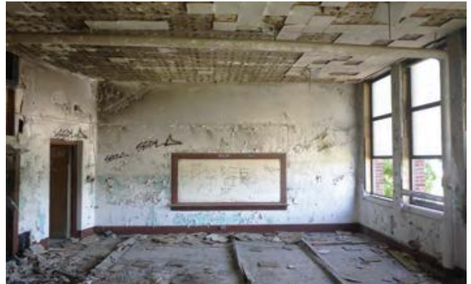
Typical classroom in 1924 unit, with plaster walls and wood floors. Aluminum replacement windows are partly intact.
