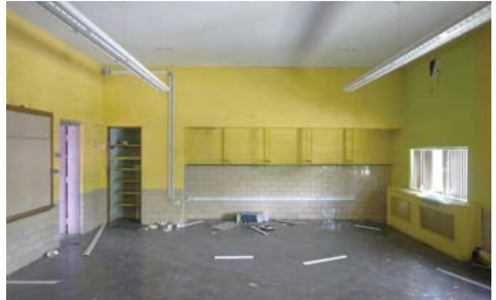
Typical classroom, view of back wall with coat/storage alcove. Note drastically reduced-size window to the right. Green painted area shows the size of the original window opening.
