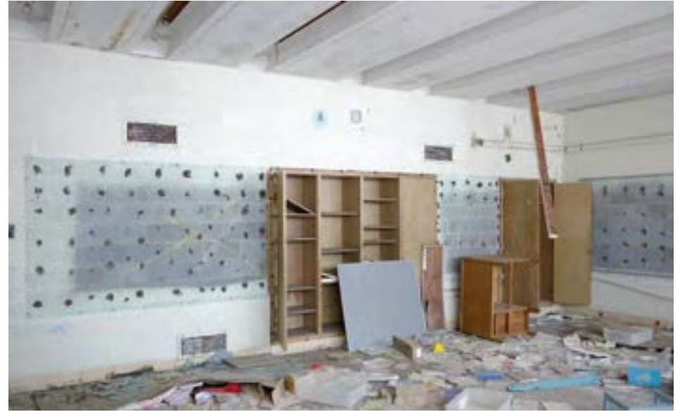
Classroom finishes are simple, including simple wood cabinetry, VCT floors, and an exposed-structure ceiling that incorporates fluorescent tube lights in between the joists.
