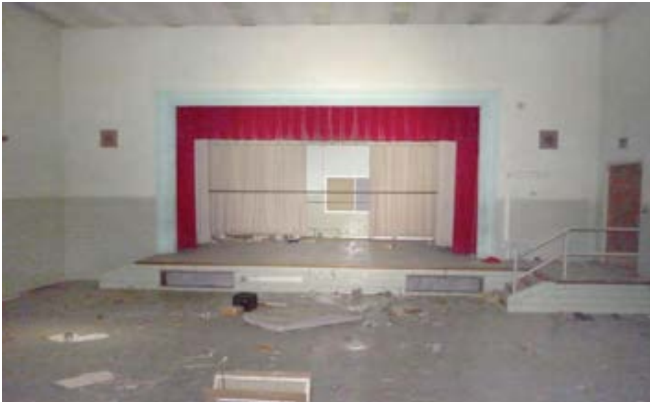
The auditorium is small, with a low stage and a flat sunken floor. The space is a simple box with painted CMU and green glazed tile matching the corridors.
