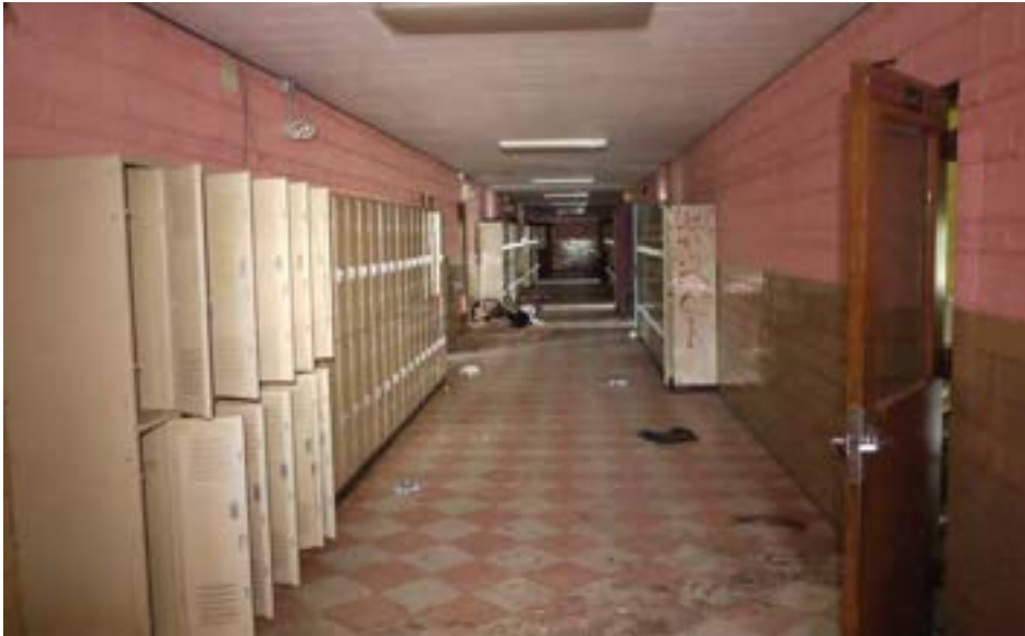
The second floor main corridor is a simple double-loaded hallway with painted CMU and glazed block walls. This hallway did not originally contain lockers; instead, students stored their coats and belongings inside the classrooms.
