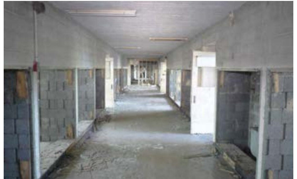
Corridor in the east classroom wing with concrete block structure visible where locker banks have been removed.
