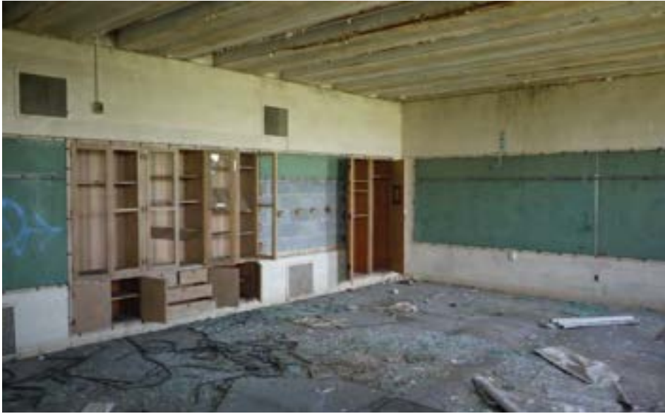
Typical 1955 classroom with concrete block walls, wood floors, and wood built-in cabinets. Note corrosion on steel ceiling system.
