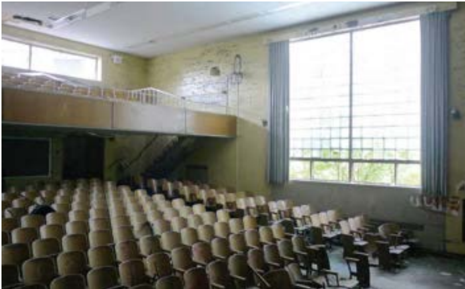
Auditorium main floor and balcony viewed from stage. The space receives most of its light from one large glass block window.
