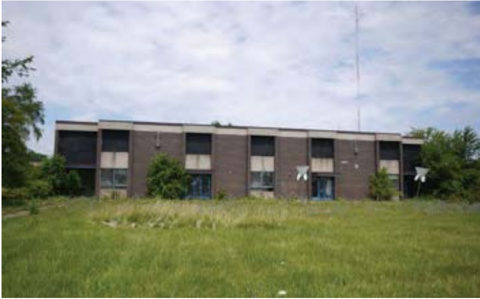
South elevation with small play field in foreground, showing a 2-story classroom wing.
