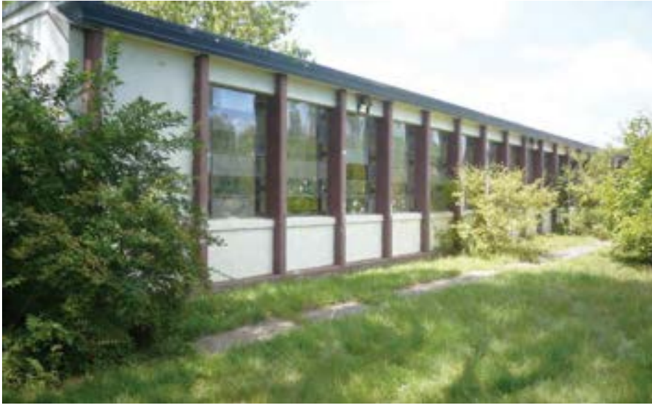
East elevation showing repeating steel-frame grid windows and concrete columns. The school's modern style is quite different from other schools built in Detroit, even others in same era. This school appears to barely predate the shift to International Style architecture circa 1950.
