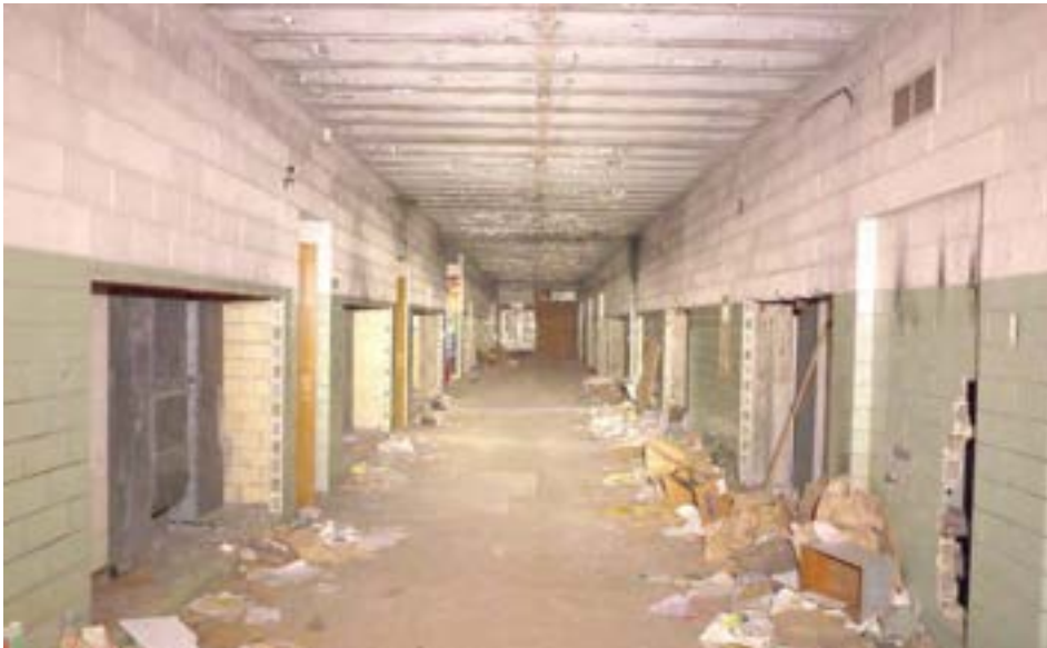
The building has been extensively scrapped, but finishes and structure remain in relatively good condition. The school's corridors feature glazed block finishes with a unique shade of jade green.
