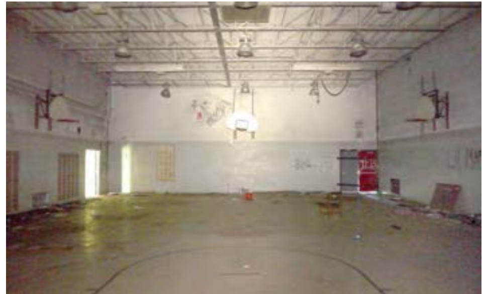
The gym is a windowless space with painted CMU walls and an open-web steel joist ceiling. The space is 45x70' with 20' ceilings.
