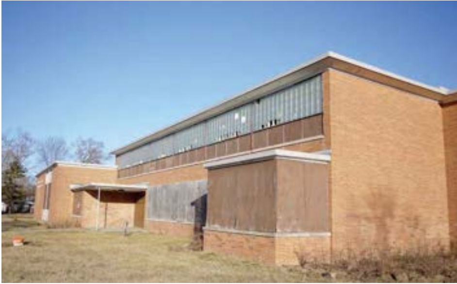
The main (south) facade of the school, showing continuous bands of glass block extending along the entire classroom wing. The windows are largely intact.
