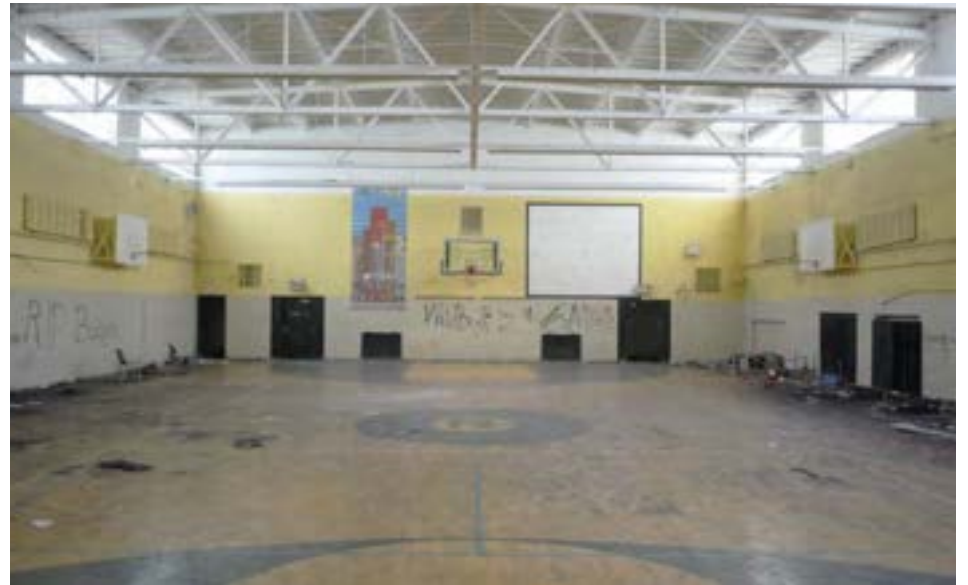
The 60x90' gymnasium is in relatively good condition. It is lit by glass block clerestory windows on the northwest and southeast elevations.
