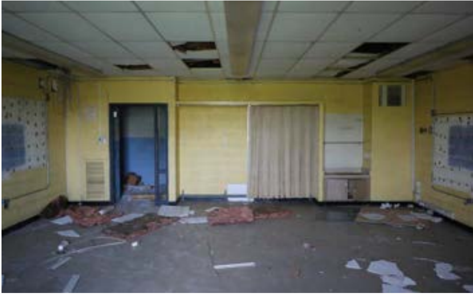
A typical 2nd classroom on the south wing. Instead of the wood built-in storage units found in most other schools, this school has a folding plastic curtain concealing a storage alcove.
