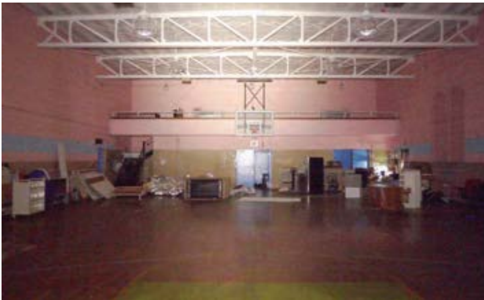
Gymnasium viewed from stage, showing balcony seating area (behind basketball hoop) with kitchen and storage areas below.
