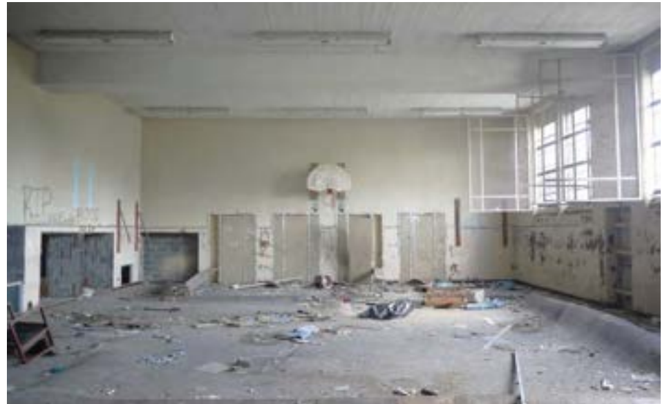
The gym is a simple concrete box with large steel-frame windows. Although there are lunch tables built into the walls, indicating the space's use as a cafeteria, the school does not have a kitchen or food serving area.
