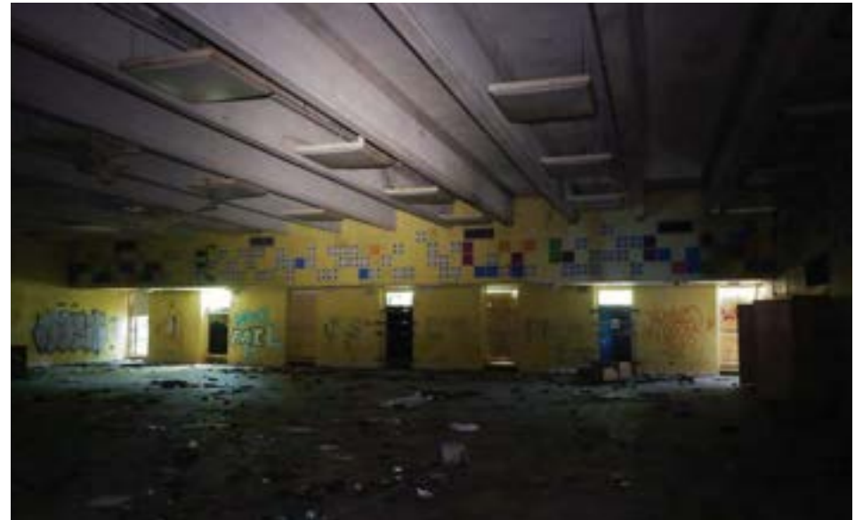
Cafeteria in 1963 unit is a spacious column-free area with long-span concrete roof.
