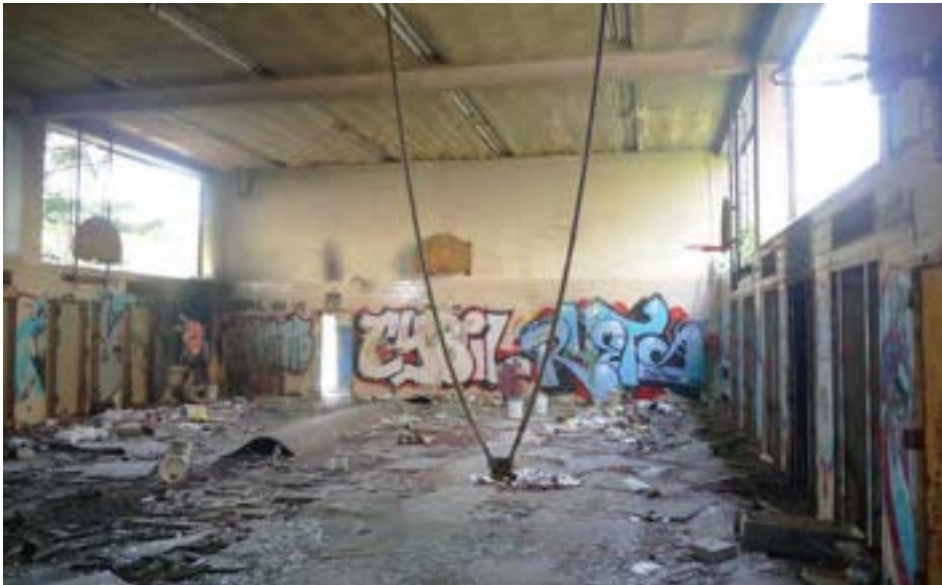
1955 gymnasium features large clerestory windows facing east and west; windows are missing but were likely glass block.
