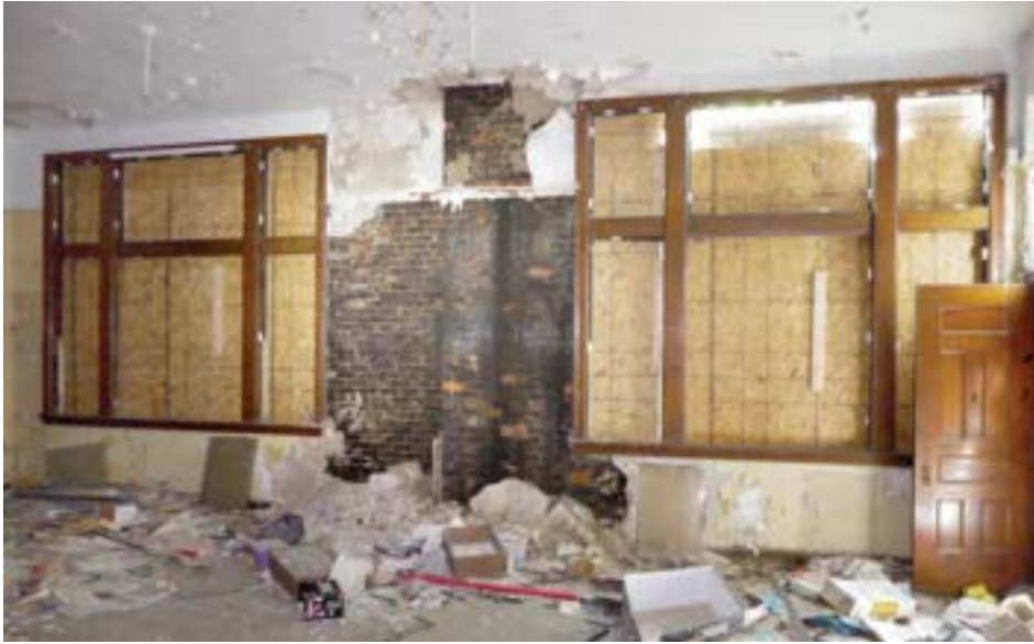
Water damage in an upper-level classroom has caused the plaster walls to disintegrate, revealing the school's load-bearing brick walls. Historic wood window frames are visible, though the original window assemblies and their modern replacements are gone.
