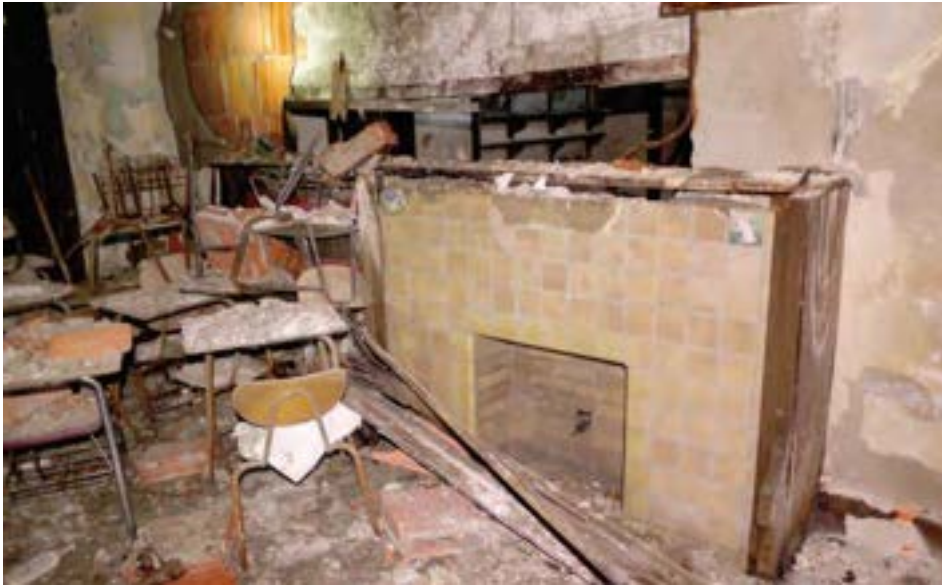
The kindergarten has been heavily damaged by water, fire, and scrapping. Most finishes have been destroyed, but this tile fireplace with prized Pewabic tiles may still be salvaged. Despite the rough appearance, however, the building's structure itself appears to be sound.
