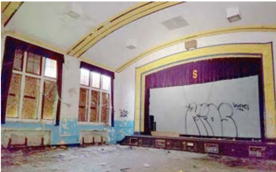
The main auditorium features a 20' high barrel-vaulted ceiling, a wide stage, and a flat floor without fixed seating. There are three large west-facing windows.
