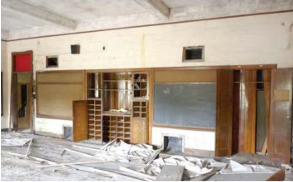
A typical classroom. Interior finishes are simple painted concrete, with built-in wood casework. Classrooms were generally in fine condition.
