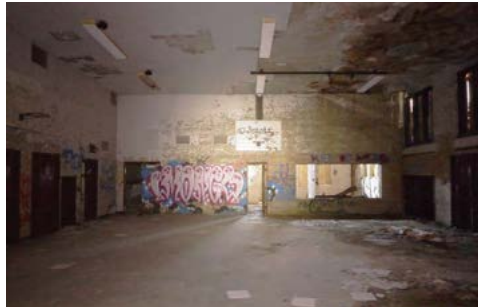
The gym/cafeteria is a simple brick box with high windows. The kitchen and serving window are visible on the back wall.
