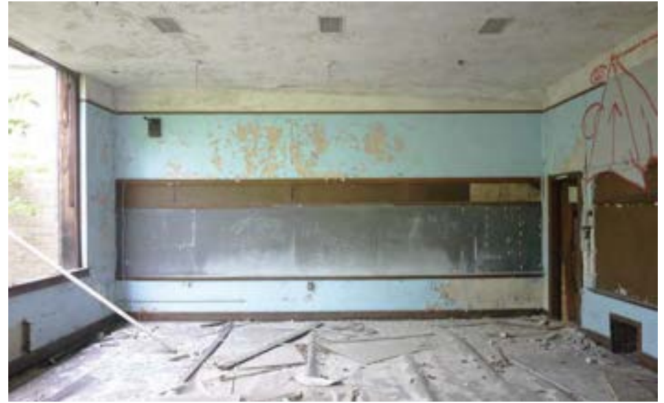
A typical standard classroom with plaster finishes and wood floor in relatively intact condition. Windows have been removed throughout the building. Classrooms at the east end of the building show considerably more distress.
