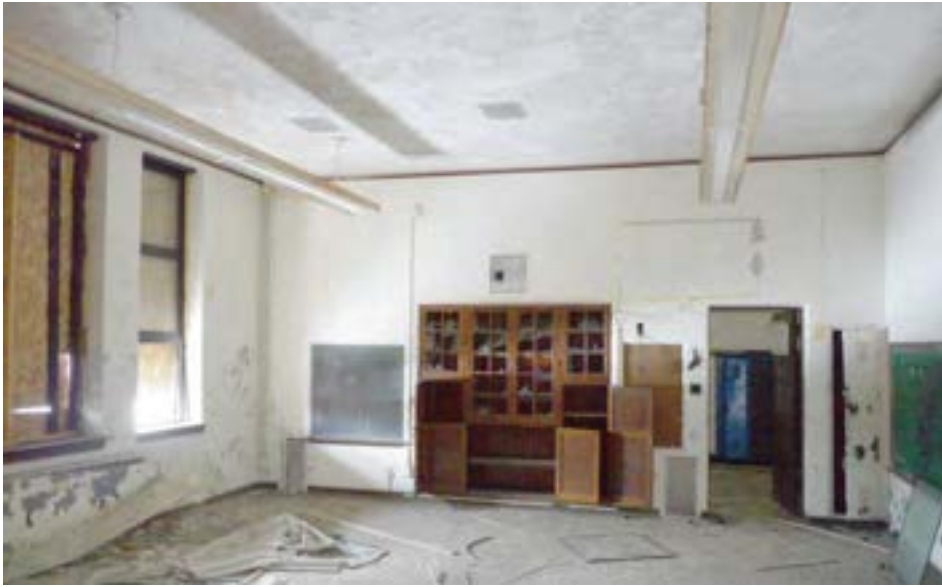
Classrooms in the older north unit feature plaster walls, built-in cabinetry and wood window frames. The original windows were replaced with modern aluminum windows, but many of those have since been scrapped.
