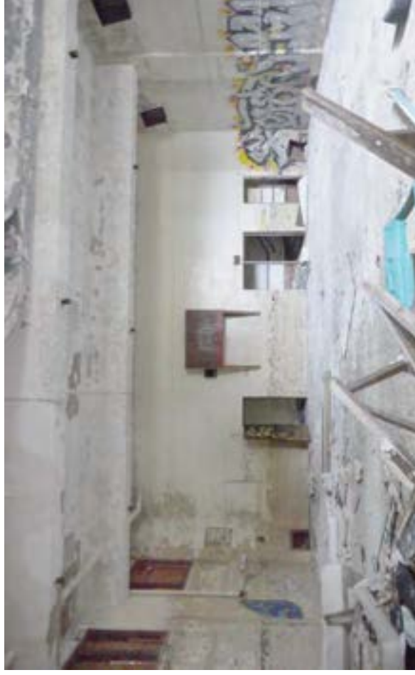
A large gymnasium with 19-foot high ceilings occupies the basement level beneath the auditorium. Large windows just above grade provide the space with ample natural light.
