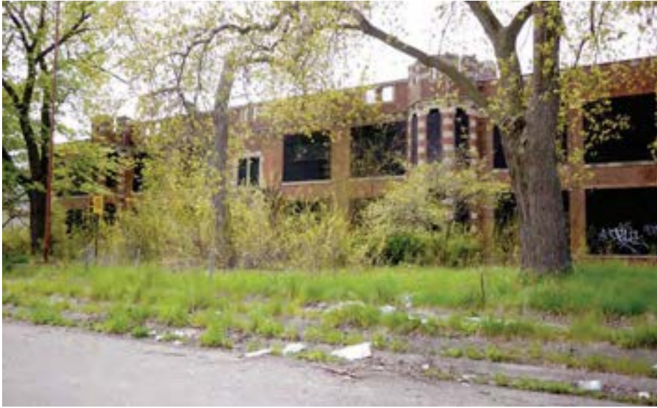
The front (east) elevation of the school is overgrown, somewhat obscuring the symmetrical Tudor Revival-style facade. Two castle-like towers with crenelated parapets flank the main entrance.
