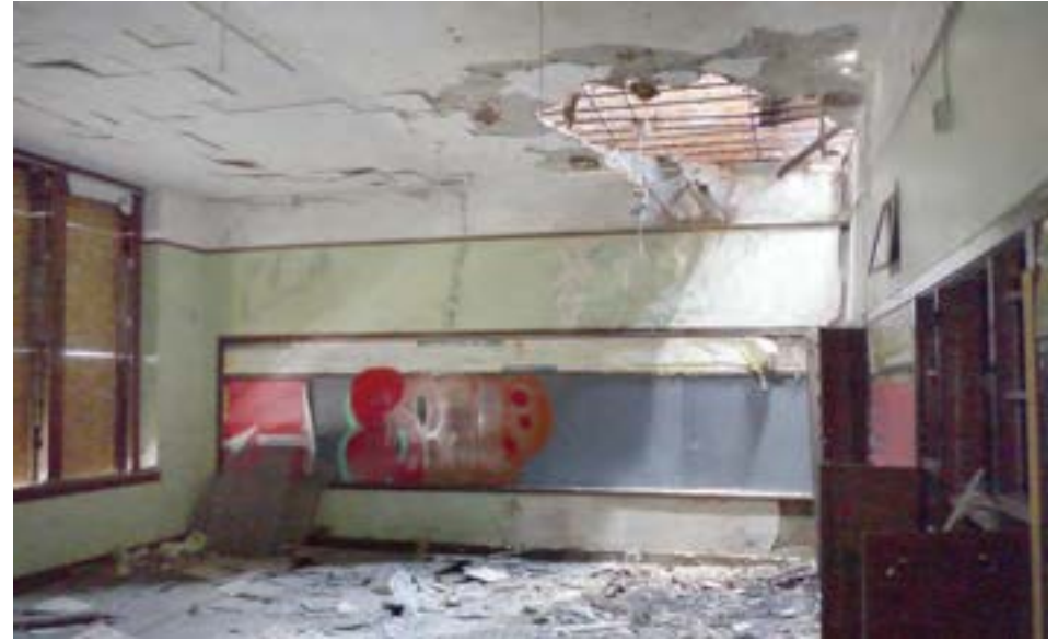
A hole in the ceiling of this second floor classroom reveals a red brick wall and soaring attic space above. The ceiling could be removed to create a loft-like space.
