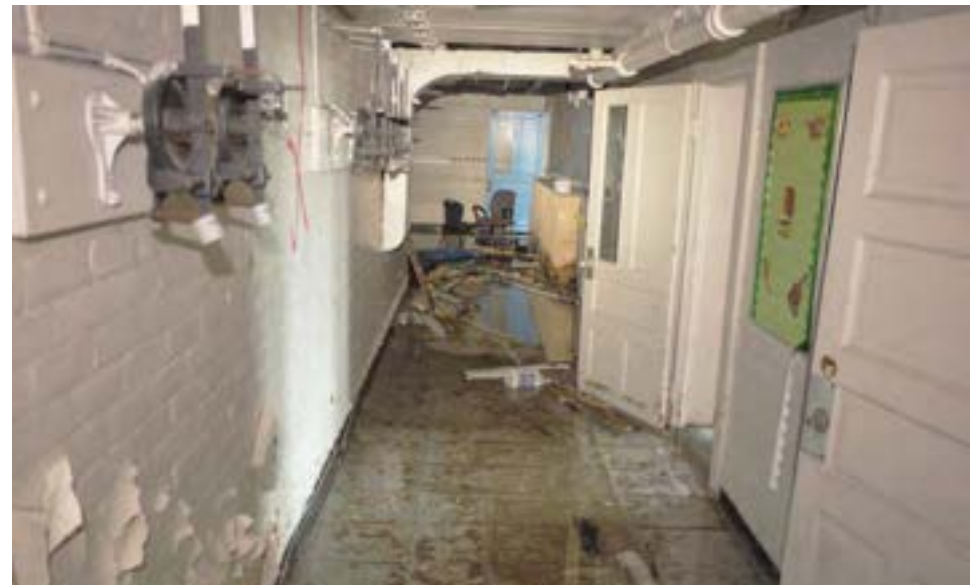
A narrow section of hallway in the basement, here, flooded with water from a broken pipe. The basement holds mechanical spaces in the center and classrooms around the perimeter.
