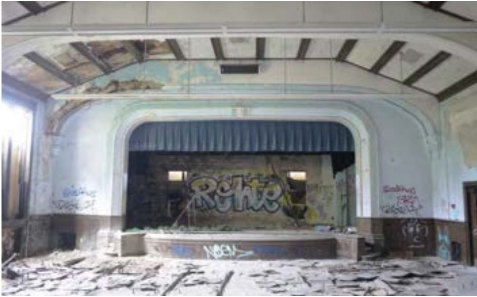
The second-floor auditorium features unique plaster detailing meant to evoke exposed heavy timbers and hammer joists
