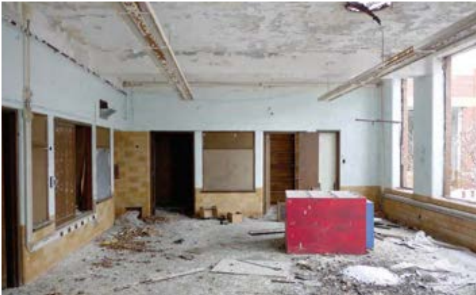
The "sewing & cooking" room is an example of a courtyard-facing classroom. Classrooms facing the interior have tall windows and direct access to the large courtyards. The durable concrete and glazed block finishes are in good condition.
