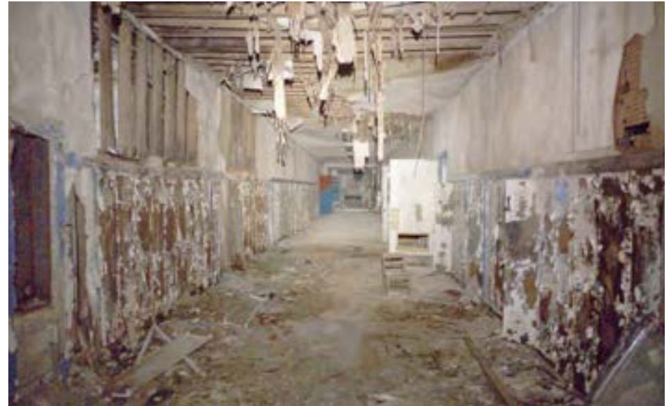
Water infiltration has damaged interior finishes in the second floor main corridor.
