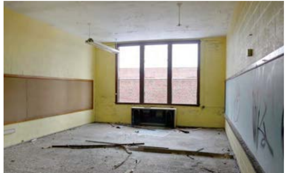
A classroom on the mezzanine level above the gym. This space was likely a second-floor playroom with the same footprint as the gym below, but was later divided into three to create additional classroom space..
