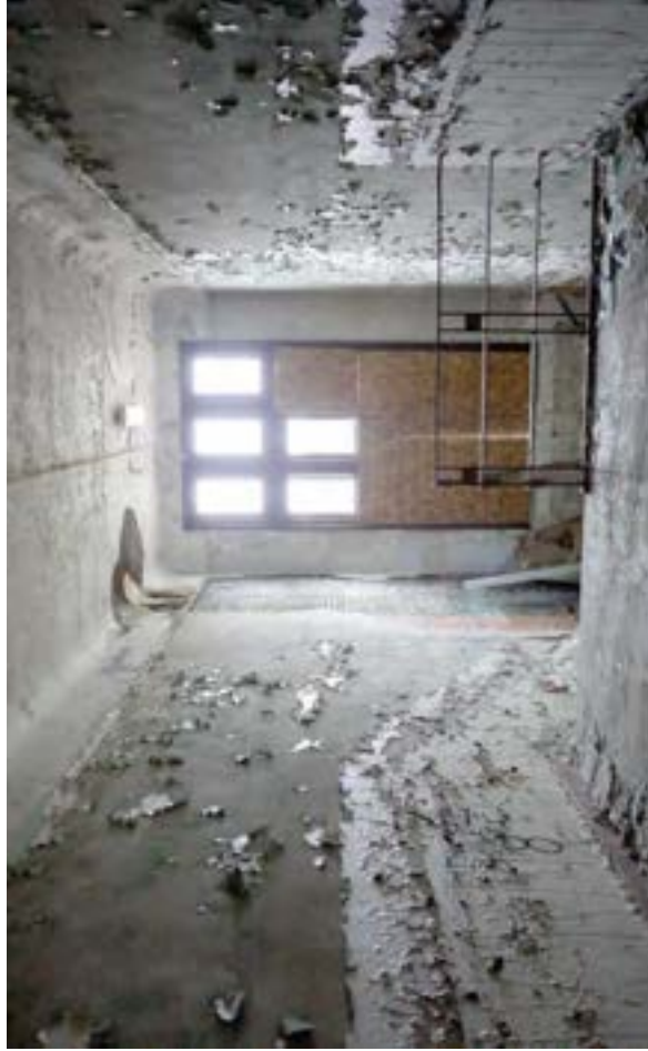
Primary stairwells at either end of the original unit feature 16' high windows that flood the corridor with natural light. Stairwells and corridors feature simple rounded covered ceilings.
