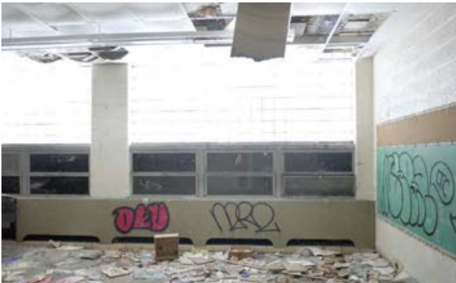
A typical classroom in the 1951 wing, featuring large glass block windows with operable steel frame lites below. The more durable painted CMU finishes in the newer wing are in relatively good shape compared to the moisture-sensitive plaster of the 1920s wing.
