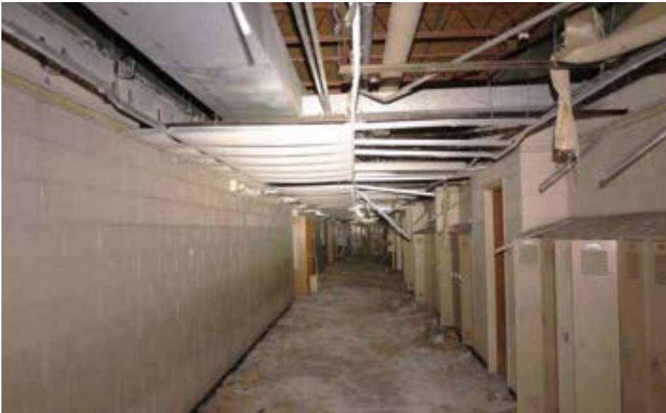
Typical hallways are narrow double-loaded spaces with low drop ceilings and no windows. Open-web steel joist roof structure is visible at top right.
