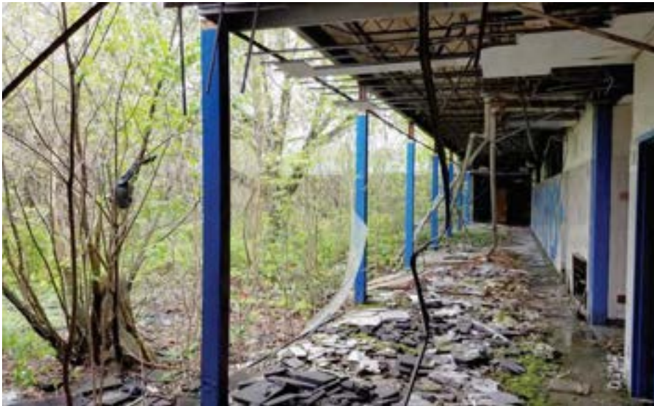
East courtyard viewed from a central connector corridor. This corridor originally featured glazed curtain walls on all four sides, but these have all been scrapped. The courtyard would have been accessible via a door near the camera location.
