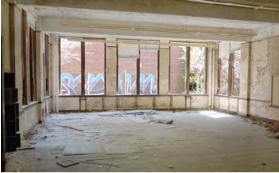
The large main kindergarten room protrudes into the central courtyard. Originally, these windows would have offered a view to the outside, but a two-story corridor connecting the north and south wings blocked off the view.
