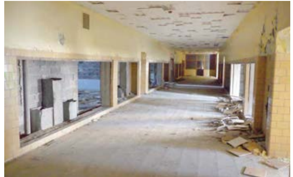
The second-floor corridor in the 1951 unit has been extensively scrapped, but otherwise, finishes are in good condition and there is little evidence of water damage.
