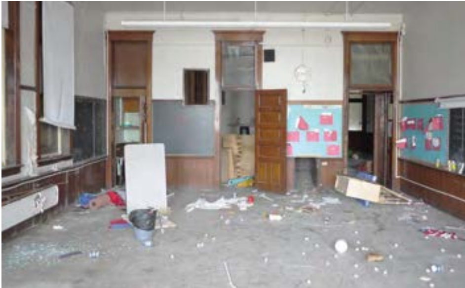
A typical central-wing classroom facing the main corridor. This former art room includes a small closet (left door) and an attached walk-in storage room (middle door).
