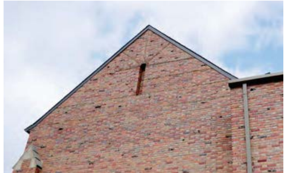
A detail of the unique tudor-revival brick details on the south elevation.
