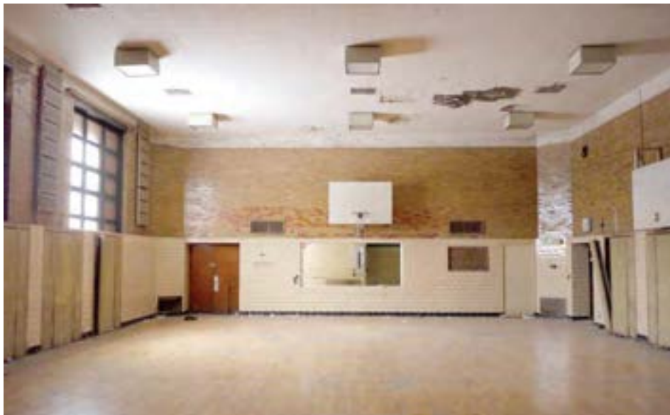
The gym was constructed in 1925 as part of the original school, though it has been updated since. It is in generally good condition.
