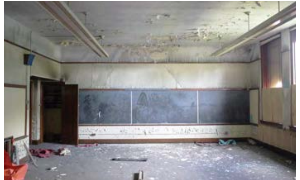
A typical classroom in the 1918 unit with finishes in good condition. Finish conditions vary a great deal in the original building, with some areas damaged by water, fire, and vandalism, and other areas in good condition.
