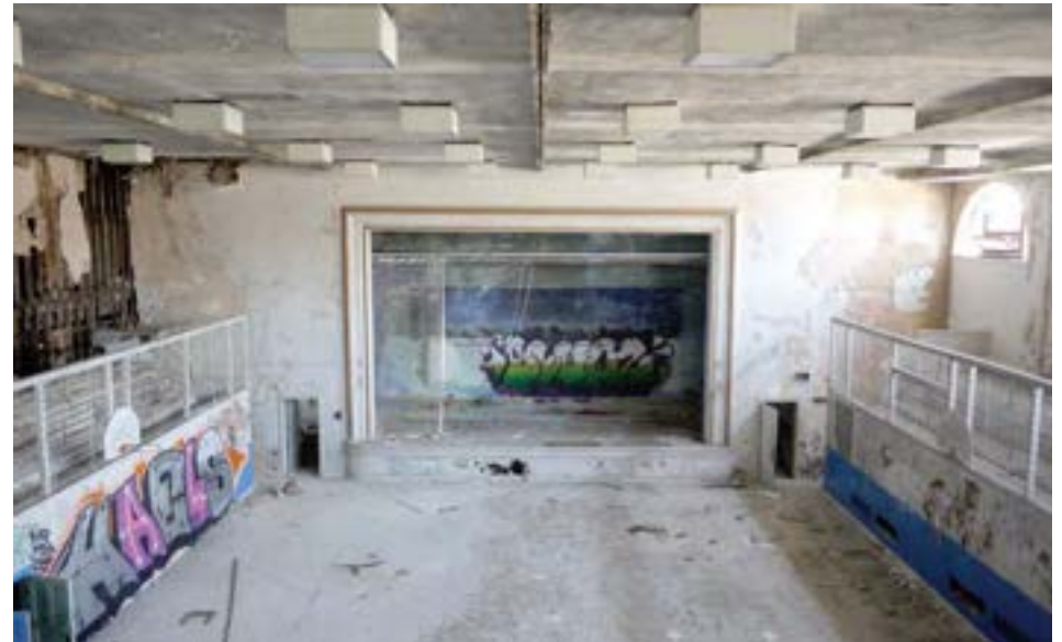
View of the gymnasium/auditorium and stage area from the second-floor projector room. Severe water damage to the wood-framed partition wall between the bleachers and main corridor is visible at the far left of the frame.
