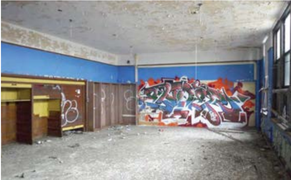
The second floor library is 8' longer than a typical classroom, and features roll-up wood cabinets. Woodwork and walls have been painted over and tagged, but are otherwise in good condition.
