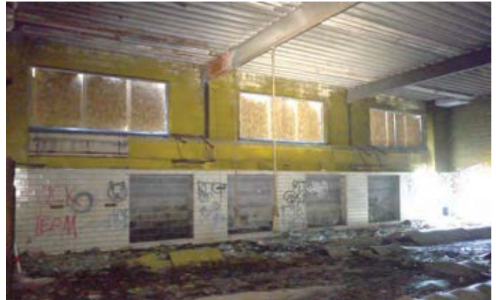
The modern gym/cafeteria is utilitarian steel frame and CMU construction. It has direct exterior access in two locations, but both are below grade and require a short flight of stairs.
