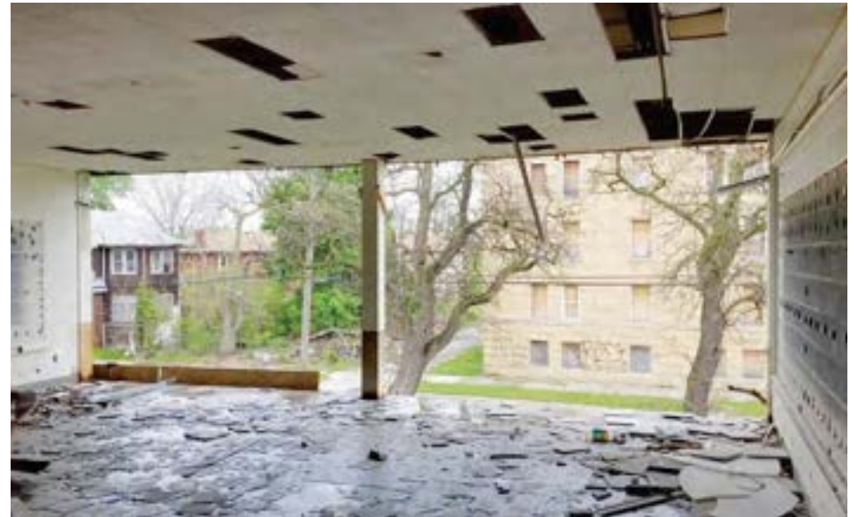
Inside a second-floor east classroom, looking toward Lawton St. The entire facade has been scrapped, revealing only the structure.
