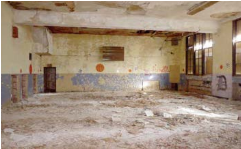
The brick gym is located in the center of the 1928 unit. The space features three large wood-framed windows that appear intact. The plaster ceiling has deteriorated and fallen, obscuring the condition of the floor itself.
