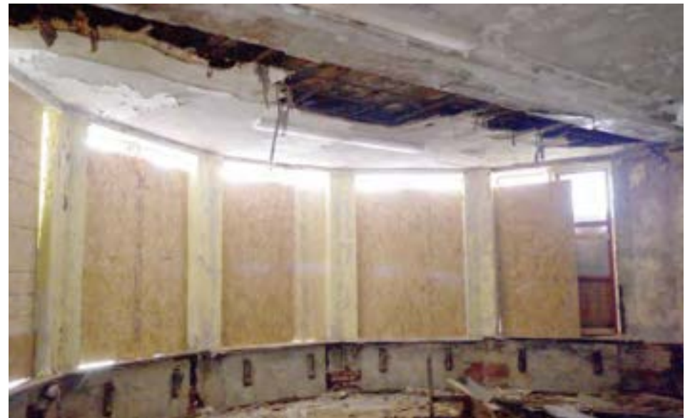
The kindergarten features a large bay window. The original wood benches and radiators have been scrapped, and water is entering from the roof where the bay window attaches to the main building.
