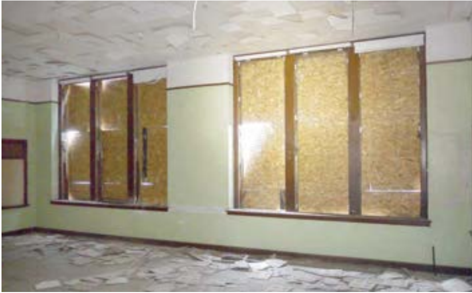
Typical classroom windows, showing original wood frames. The window assemblies were replaced with aluminum replacements, which have since been scrapped.
