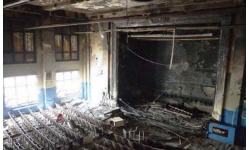
The 1918 auditorium is a grand space with a large balcony and 30' ceilings. The second floor corridor has large windows that overlook the auditorium, where this photo was shot. The stage area has significant fire damage.
