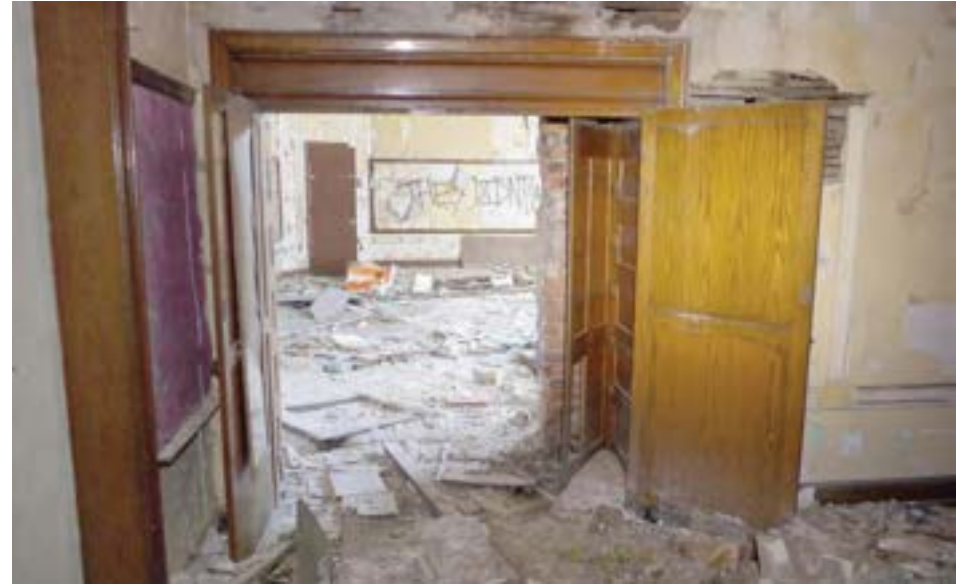
The passage between conjoined classrooms on the second floor reveals the thick walls; inside are brick shafts which travel from the basement through to the attic.
