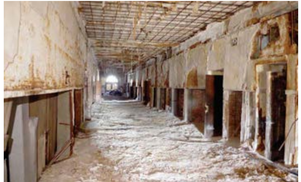
The interior of the building has suffered from extensive water infiltration and scuffing. This image shows the first floor east corridor, part of the first addition in 1928. The slab above is exposed and may require replacement.
