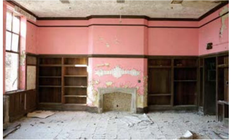
Classroom 101 is a small library space located on the first floor in the original 1925 north unit. It is one of the few rooms with intact original finishes, including built-in shelving, a stone fireplace, and decorative plasterwork. Wood frame windows are intact, but need repair.
