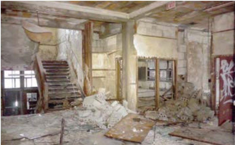
Gypsum block walls on the first floor have collapsed due to water infiltration, revealing the concrete frame. This photo shows the large cross-shaped landing between two facing stairs.
