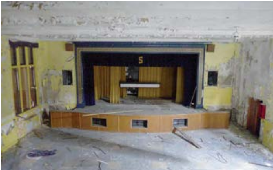
The auditorium and stage viewed from the small projection box. The auditorium has a flat floor and no fixed seating. The auditorium itself is not particularly large, but the generous stage give it a grand feel.
