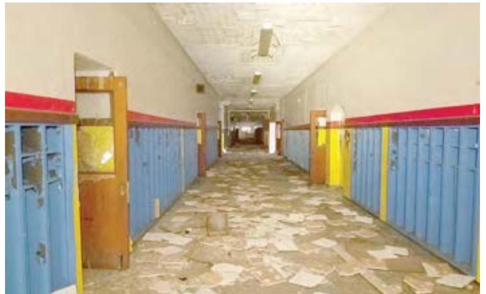
The long main corridor is 14' wide and has 11-12' high ceilings. The interior finishes are mostly intact, though the locker doors have been removed by scappers.
