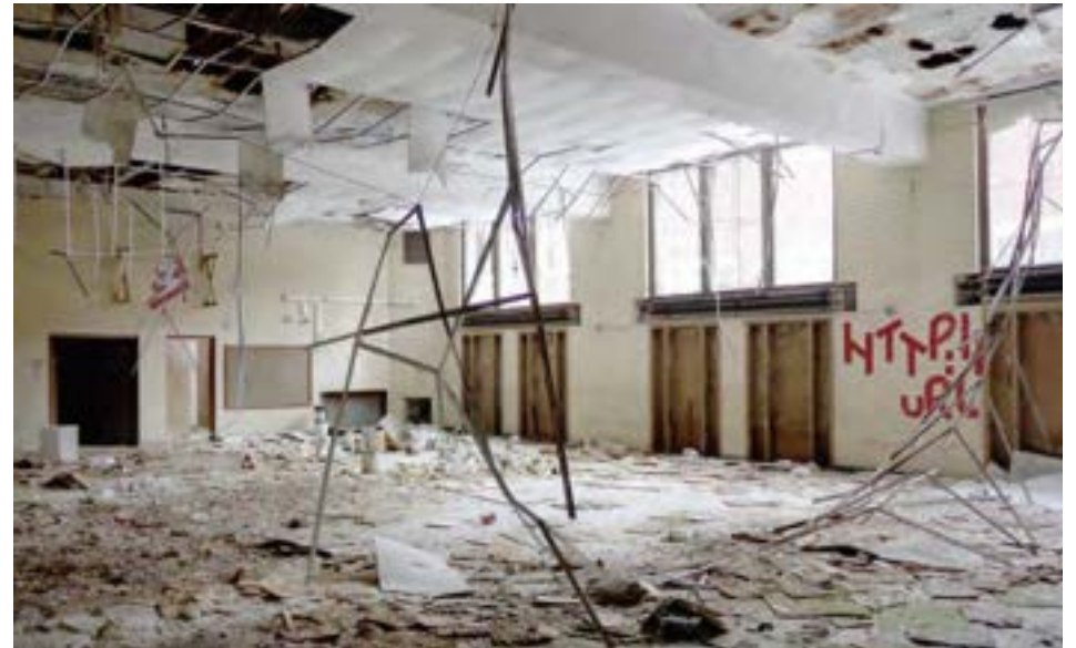
Water damage above the gym has caused the ceiling to collapse. There are three classrooms above this gym.
