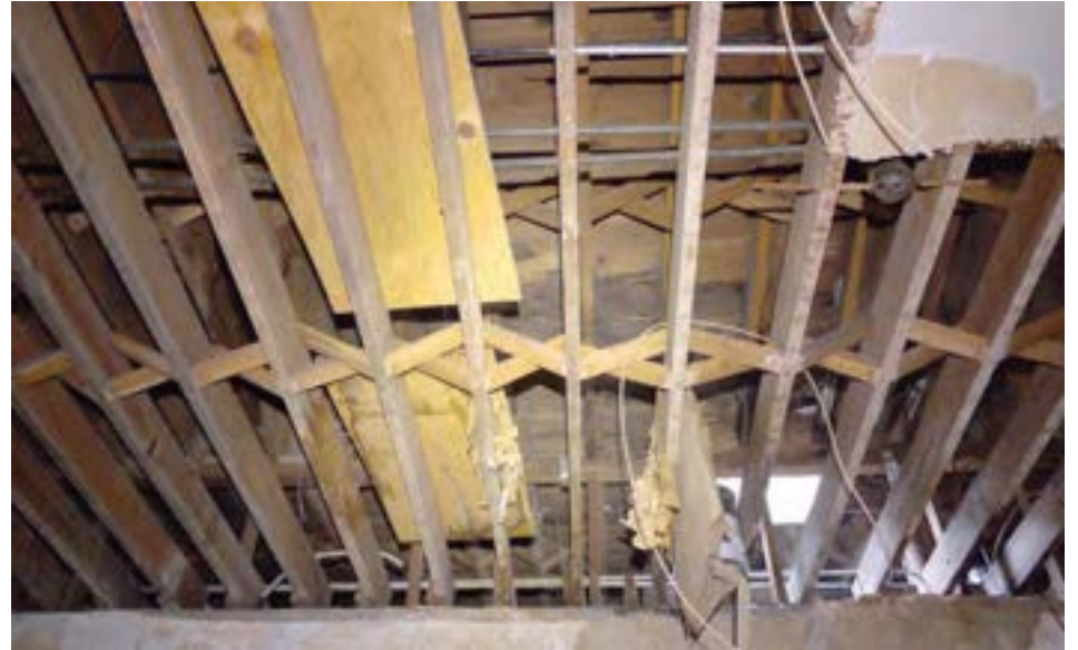
Hanneman has a wood-framed roof sitting on load-bearing brick exterior walls with an internal concrete frame. The roof is water damaged and requires replacement.
