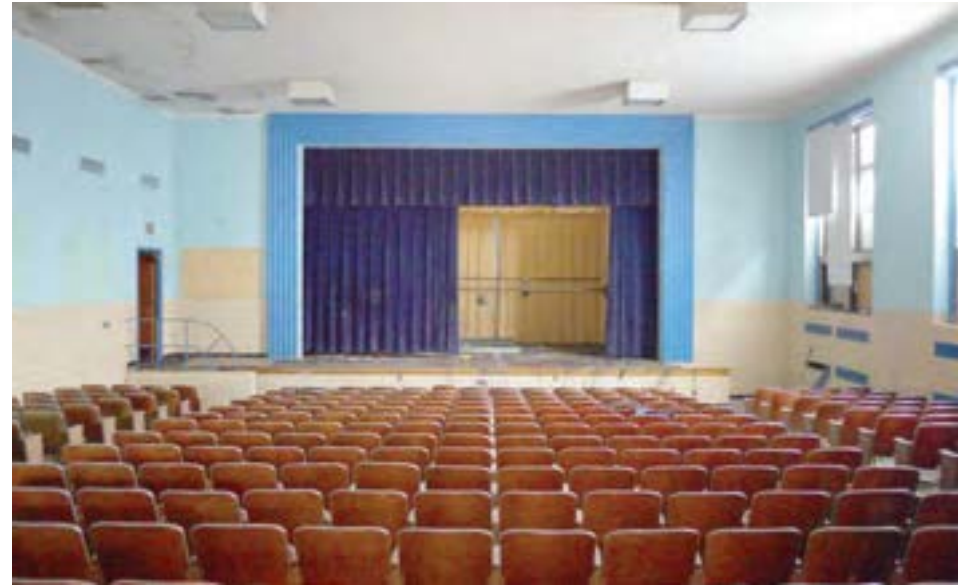
The school auditorium is a large, utilitarian box. The auditorium is accessed through a vestibule that can be closed off from the rest of the school. Conditions are generally good, with seating, windows, and finishes largely intact.
