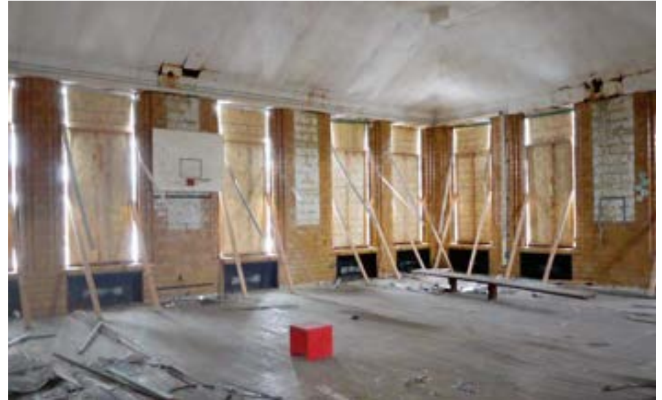
The play room/gymnasium anchors the southeast corner. It is surrounded by tall windows and was brightly lit even with its windows covered in plywood. This image highlights the extensive use of rounded glazed block throughout the building.
