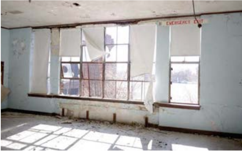
This second-floor classroom in the original 1925 unit features steel-frame windows instead of wood. Although the frames are present, the windows need repair.
