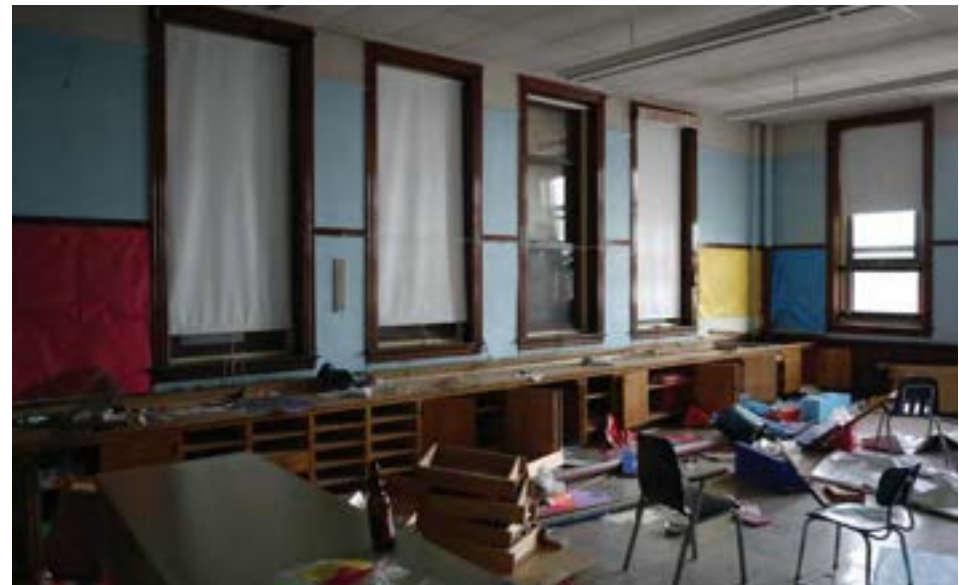
Typical corner classroom with windows on two elevations. Original wood frame windows have been replaced with modern aluminum assemblies. Plaster and wood finishes are in generally good condition throughout.
