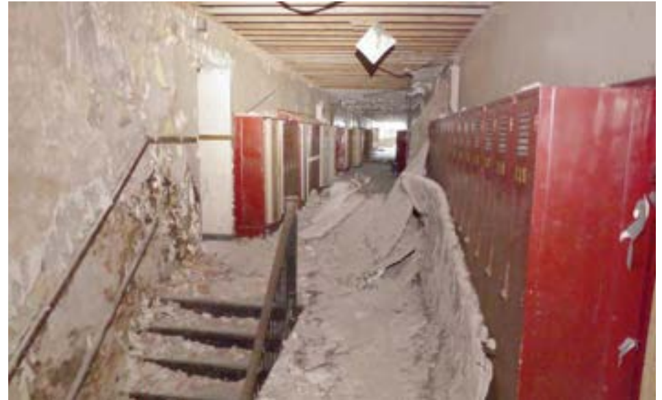
Corridors in the original south unit are 10' wide wall to wall, but feel narrower due to locker banks added later. Water infiltration in the south unit has caused the second floor's plaster ceiling to collapse and has caused widespread water damage in classrooms on both floors.
