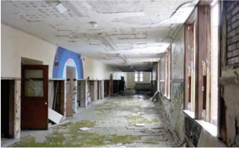
Water damage on the second floor has contributed to structural deterioration of the floor slab. The corridor floor slabs may need to be replaced.
