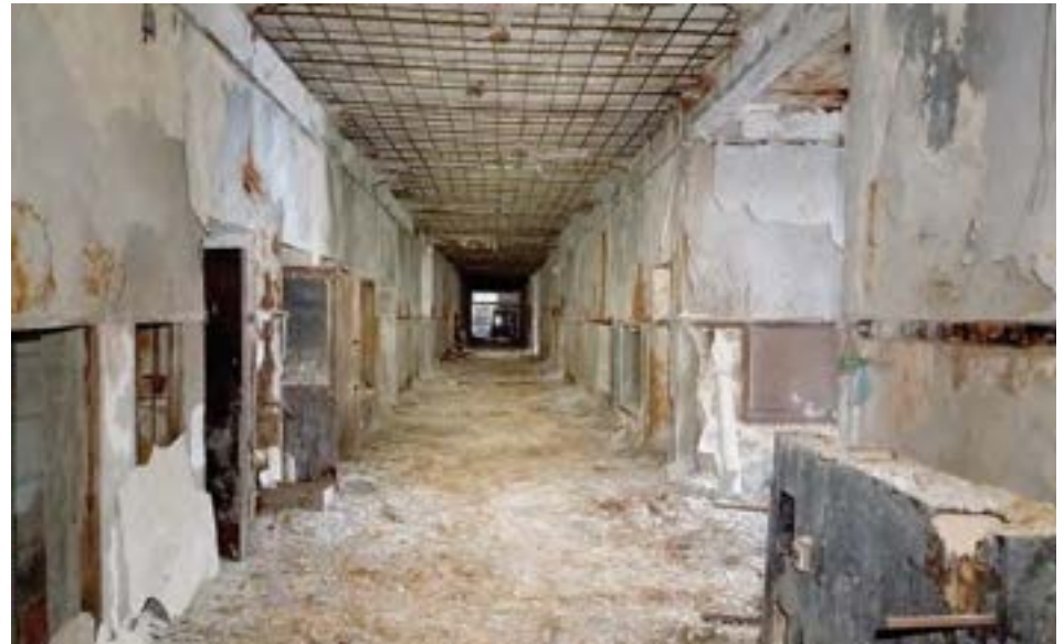
The interior has suffered from a great deal of water infiltration on both floors. The first floor main corridor shown above has had major deterioration of its plaster finishes; gypsum block non-bearing walls are also vulnerable to water.
