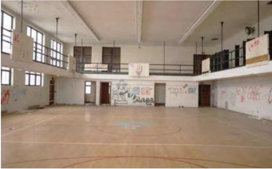
The "girls gym" is brightly lit thanks to large windows on two elevations. There is a suspended track or seating area around a full-size basketball court.
