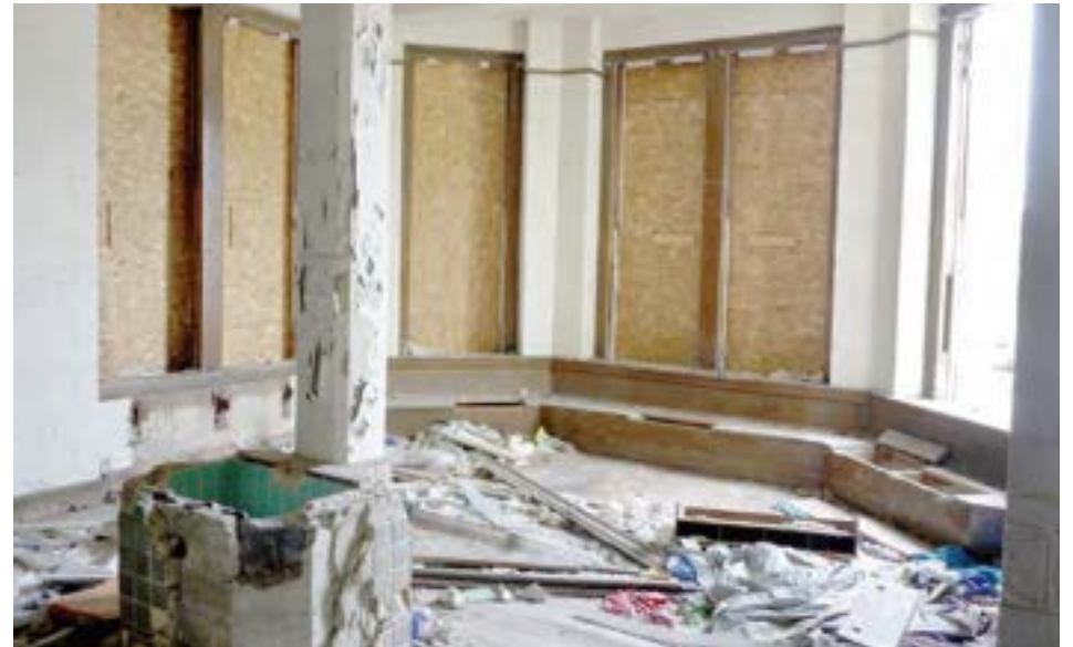
The kindergarten features a large bay window with bench seating commonly found in historic kindergartens. The basin in the center of the room (lower left corner of photo) is an unusual feature; many of the decorative animal tiles (possibly Flint Faience) have been chipped away.
