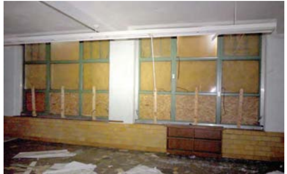
Typical classroom windows are modern aluminum-frame replacements. The wood shelf visible in the bottom right of the image is filling in the opening where there was once a door leading to the exterior terrace.
