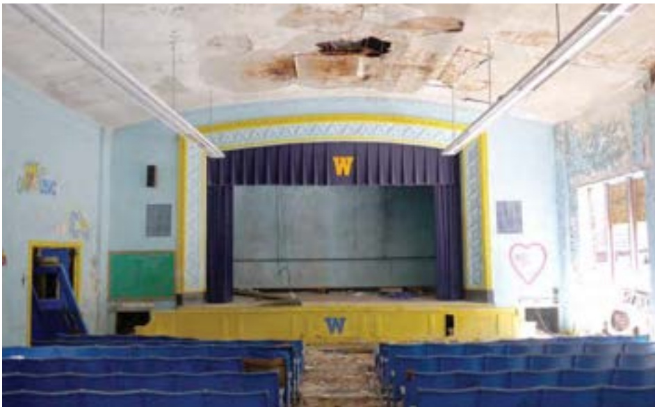
The auditorium has a plaster barrel-vault ceiling and low windows looking into the central lightwell. Water infiltration has damaged the ceiling and wood floors. Seating is still intact.
