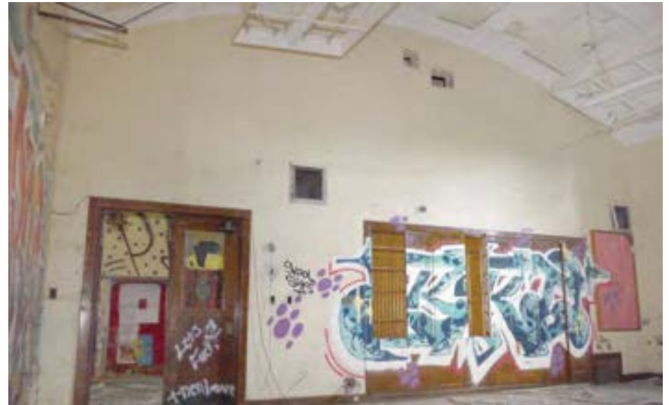
A small barrel-vaulted auditorium is on the second floor above the kindergarten. The stage has been closed off with drywall.
