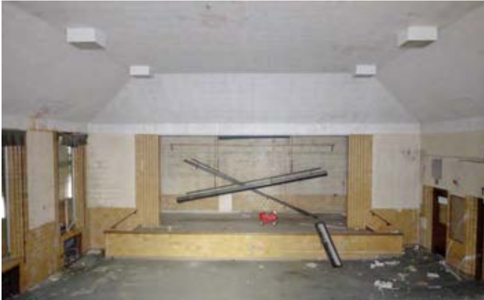
The school's corners are anchored by four large spaces with similar dimensions. The auditorium is distinguished from the other three spaces by its extended stage, a mezzanine projector room, and a dedicated street entrance with vestibule. It also has fewer windows than the other corner rooms.
