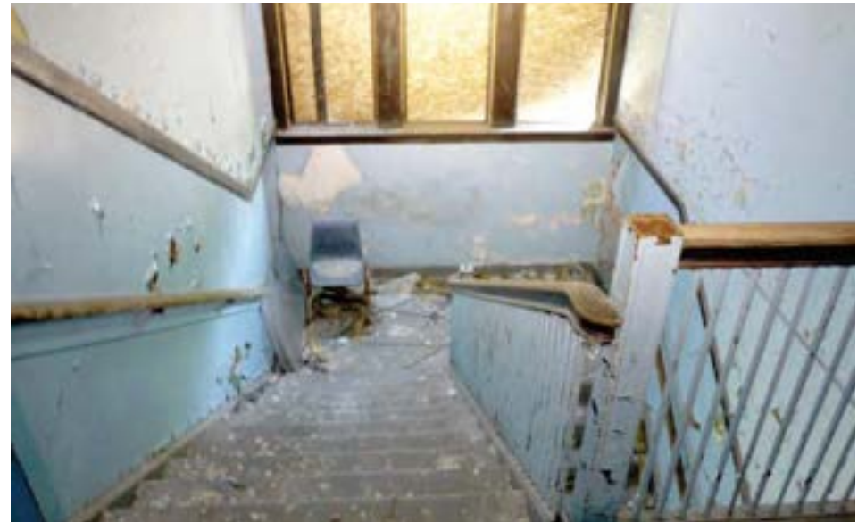
Stairwells in the original unit are tall and narrow; with flights of stairs at every entrance and a split-level first floor, this building is not ADA accessible.
