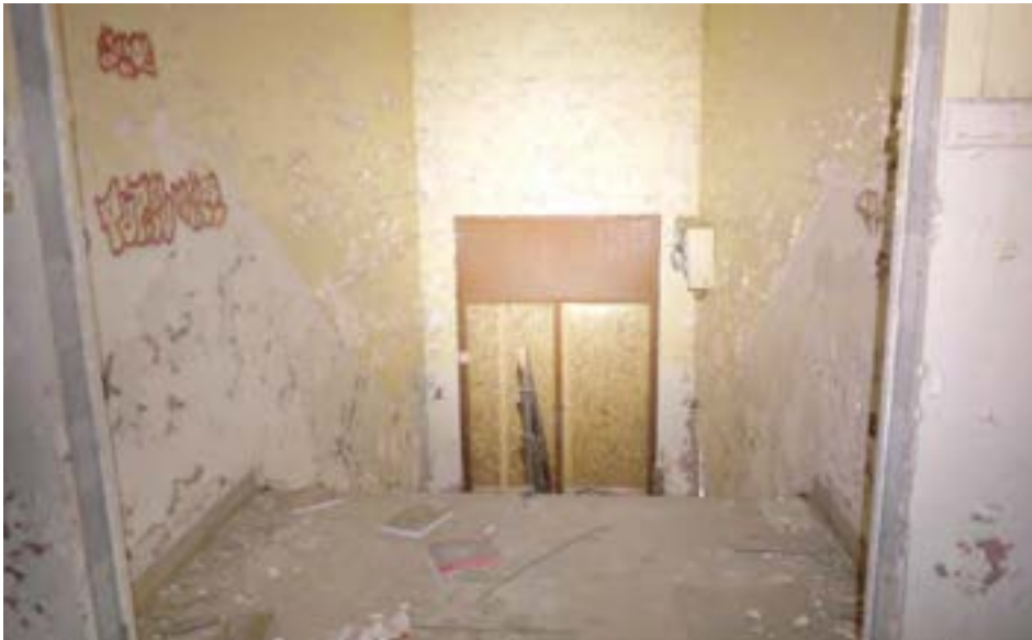
The original front entrance of the 1905 school, viewed from the first floor. The original school building is built on a raised basement, so all entrances have flights of stairs and are not accessible.
