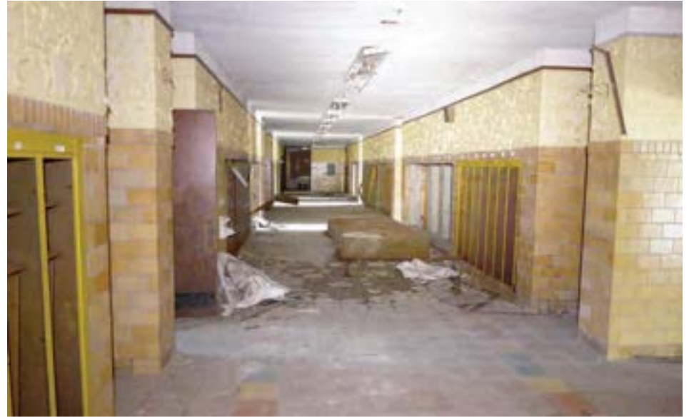
The second floor corridor. Lockers have been partially scrapped, but other finishes are in relatively good condition.
