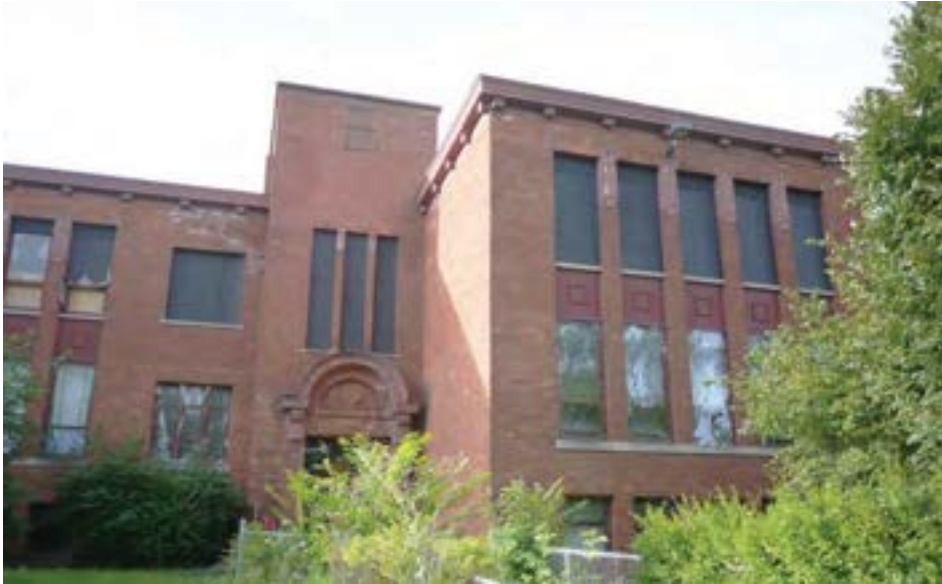
North (front) elevation of the original 1918 building. This view shows the west entrance, one of two main entrances. According to original plans, there was a raised "terrace" in the setback area at left, though this has been removed.
