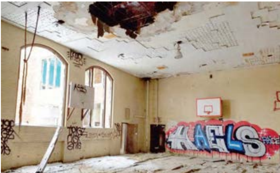
The gym is a mass-masonry brick box with tall arched windows. The wood roof deck has deteriorated, resulting in water damage to the ceiling and floors.
