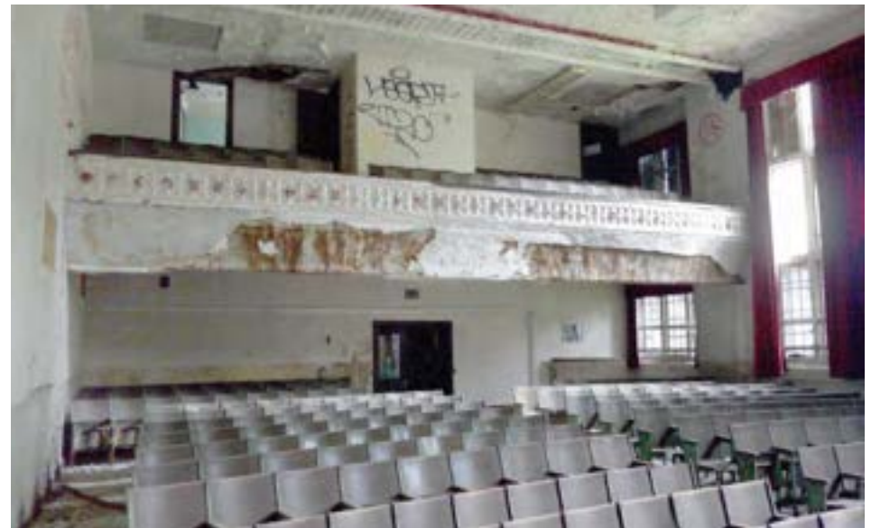
The auditorium has been damaged by the elements, but features a balcony, tall windows, and ornate decorative plasterwork.
