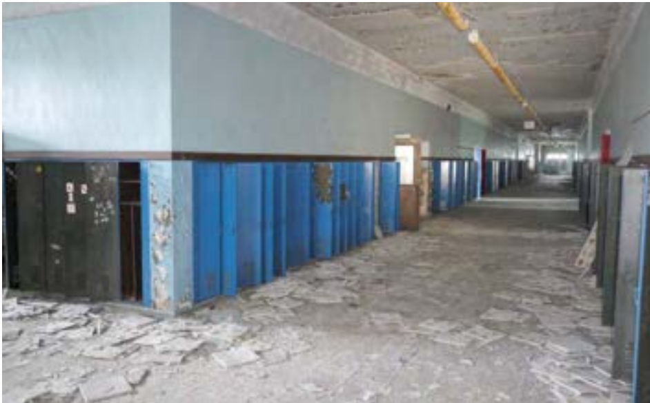
The spacious second-story main corridor is 14' wide. The plaster finishes and lockers are still in relatively good condition.
