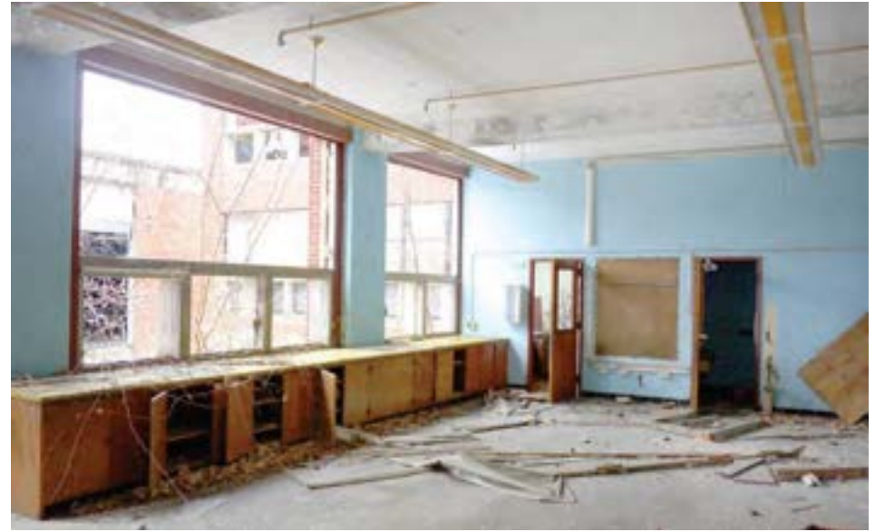
Classrooms in the 1951 addition featured large modern-style windows which formerly held glass block with operable steel-frame lites below. The original materials appear to have been replaced with aluminum frame windows, but those are largely missing.
