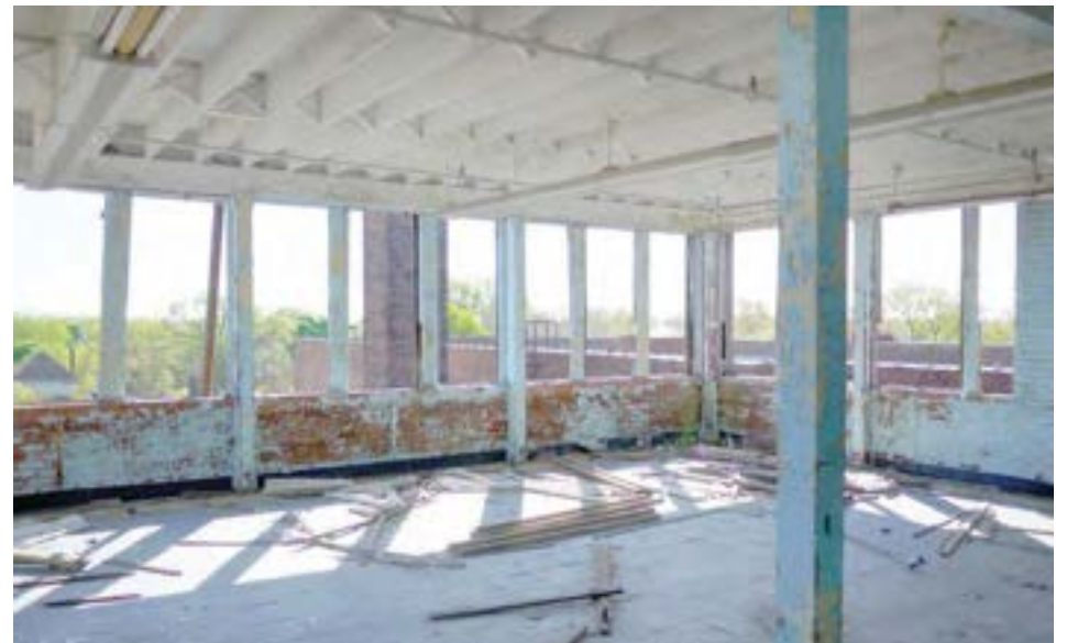
A small cafeteria occupies the center of a timber-framed penthouse added to the roof of the original school building. The penthouse has continuous windows around most of the perimeter and views across the neighborhood.
