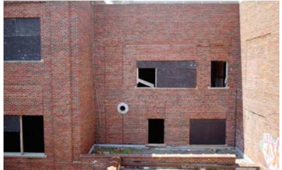
The central courtyard viewed from a restroom. Differences in brickwork show the original location and size of windows. The courtyard allows light and fresh air, but is not accessible. There is also no landscaping or greenery, since the courtyard "ground" is actually the roof of the basement boiler rooms.
