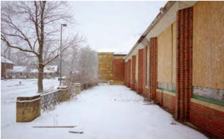
Oakman has exterior terraces on the south, east, and west sides. Classrooms around the outside of the building once had access to these terraces, but the doors are now gone. The brick infill where a door once stood is visible beneath the second window from the right (bottom right corner of photo)
