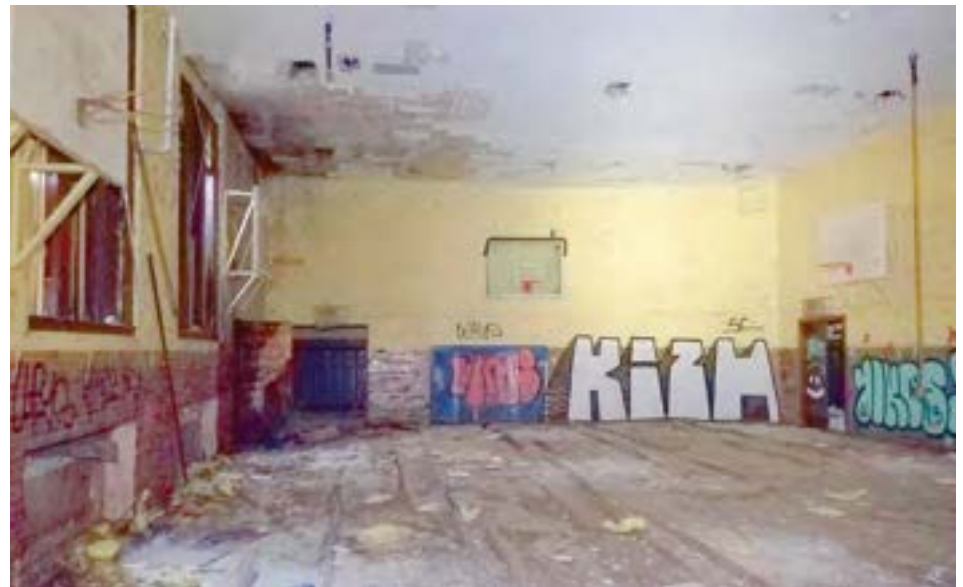
The gym is a simple 40x60' brick box with 17' ceilings and large east-facing windows.
