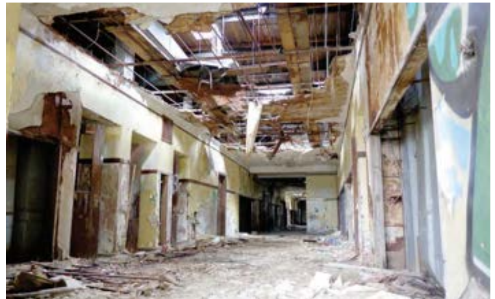
The second-floor main corridor. The school's main hallways are a generous 13 feet wide. A deteriorated roof has led to widespread water damage throughout the second floor.
