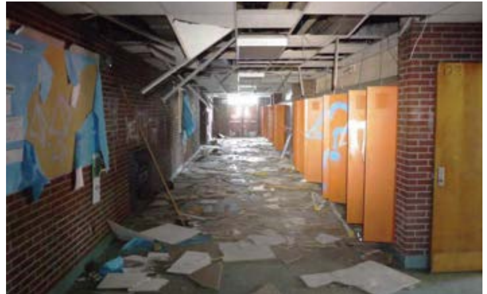
A classroom hallway in the 1963 addition. This area exhibited localized water damage and vandalism, but was in otherwise good condition.
