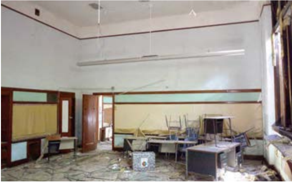
First floor classrooms in the 1923 (south) wing have 16-foot-tall ceilings, and high ceilings, giving the spaces a cavernous feel.
