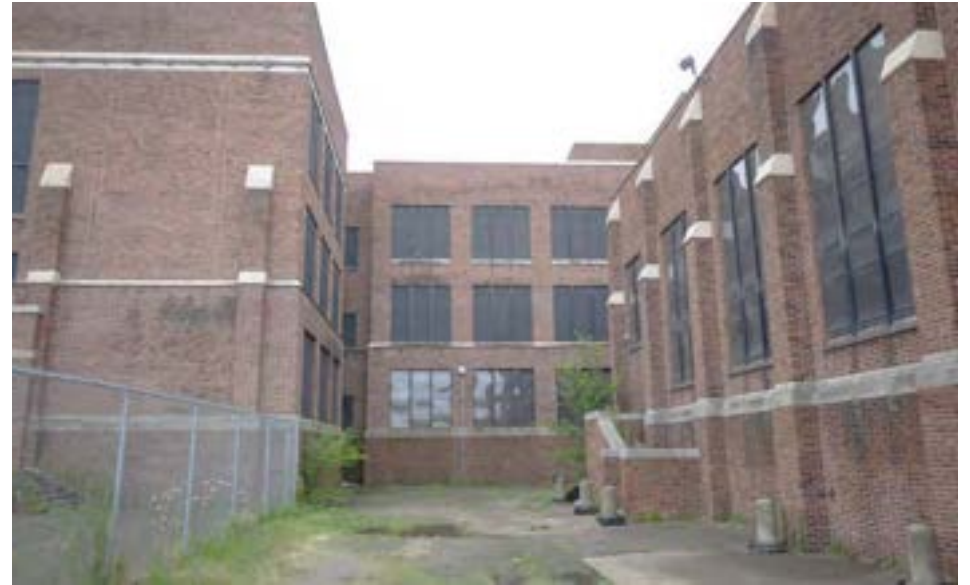
The east (rear) elevation is plain, with drab paved courtyards providing light, ventilation to classrooms and access to back-of-house operations.
