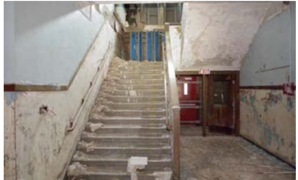
A rain storm caused water to pour down stairs at the north end of the building. The roof has been repaired, but water infiltration continues to be a widespread issue and a threat to the building.
