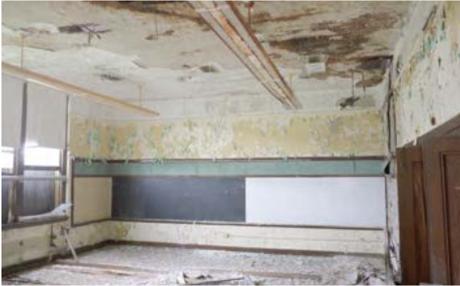
Many classroom finishes are still intact, including many wood-framed double-hung windows. Intact historic windows are a rarity in vacant school properties.
