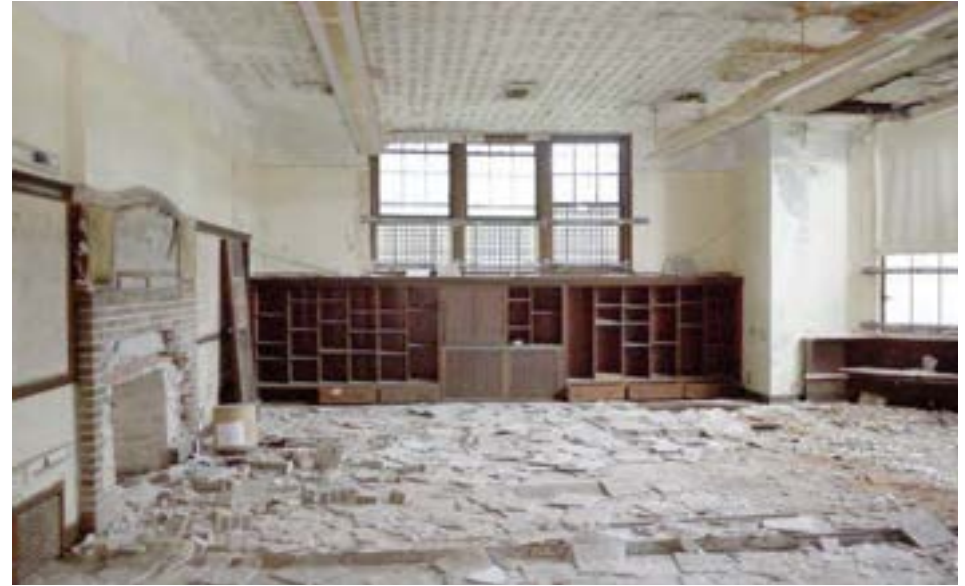
The kindergarten is spacious and once featured beautiful details; however, vandalism and water damage have taken a toll on the woodwork and tiled fireplace.
