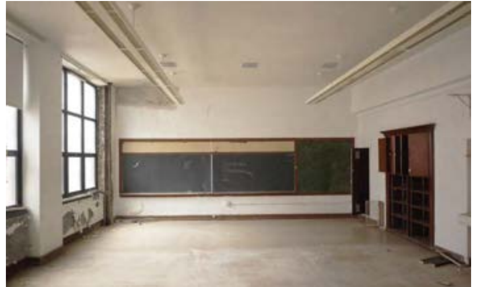
A typical classroom with finishes in good condition. Classrooms are small and squarish, with simple plaster finishes. Windows are aluminum replacements in serviceable condition.
