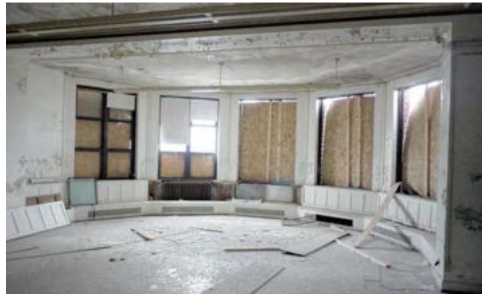
The kindergarten in the original north unit features a large east-facing bay window/play area with intact bench seating.
