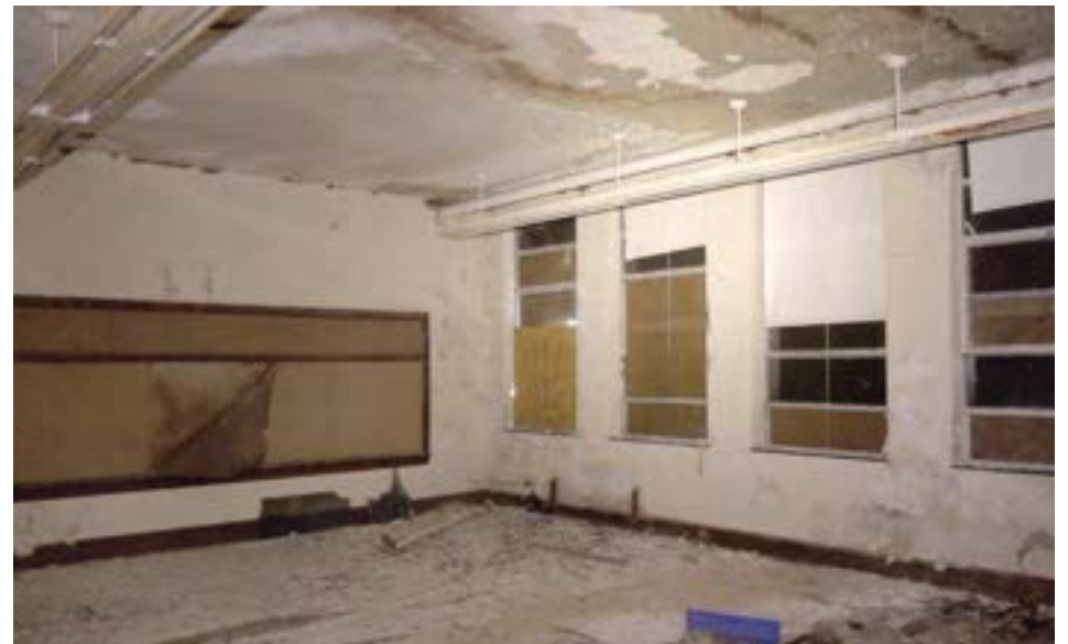
Operable steel windows are generally intact throughout the 1920s classroom wing. These likely date to the 1951 update of the building. Water damage is causing the plaster ceiling to sag.
