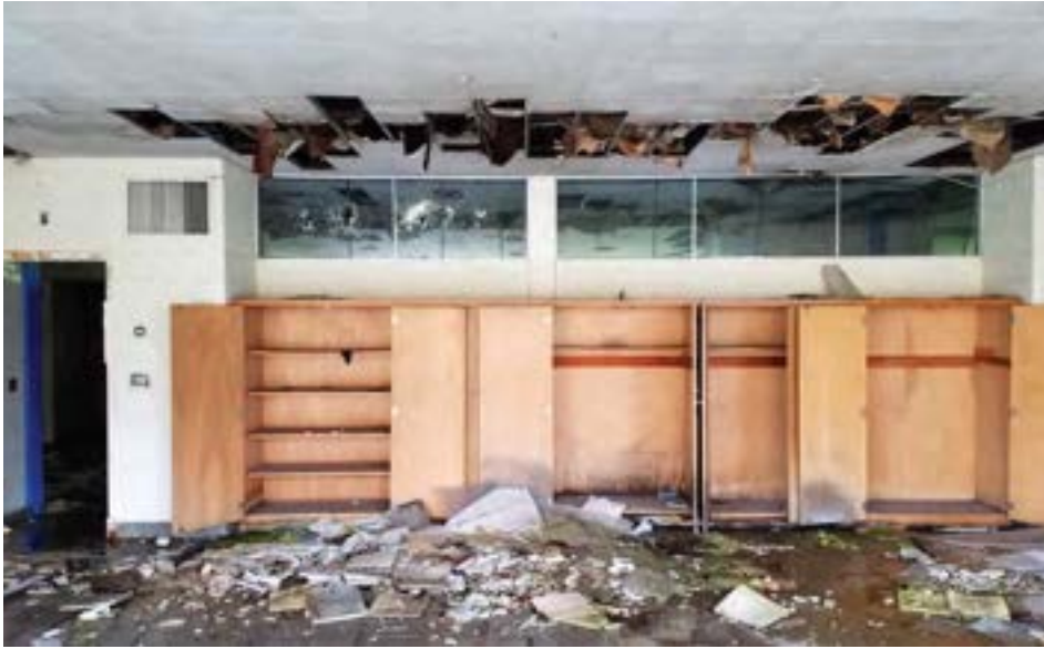
A typical classroom in the original 1961 unit, showing a storage alcove with simple wood cabinetry. Clerestory windows along the corridor wall allowed natural light into the narrow, double-loaded corridors.
