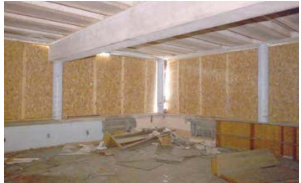
The kindergarten, located at the northeast corner of the building, features continuous glazing on two sides, designed to flood the space with natural light. The school's concrete post and beam structure is clearly visible.
