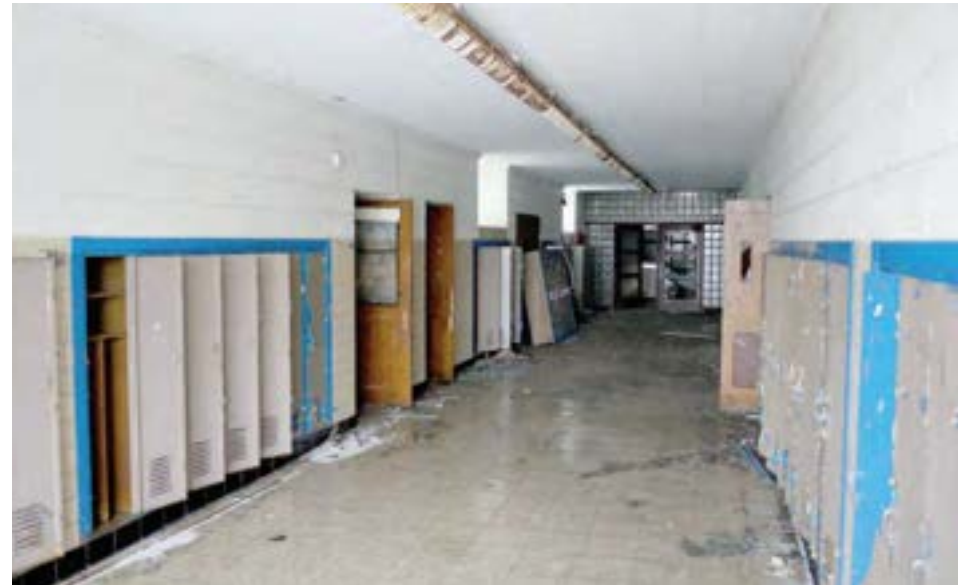
A corridor in the 1951 wing, with painted CMU, glass block, and built-in lockers.
