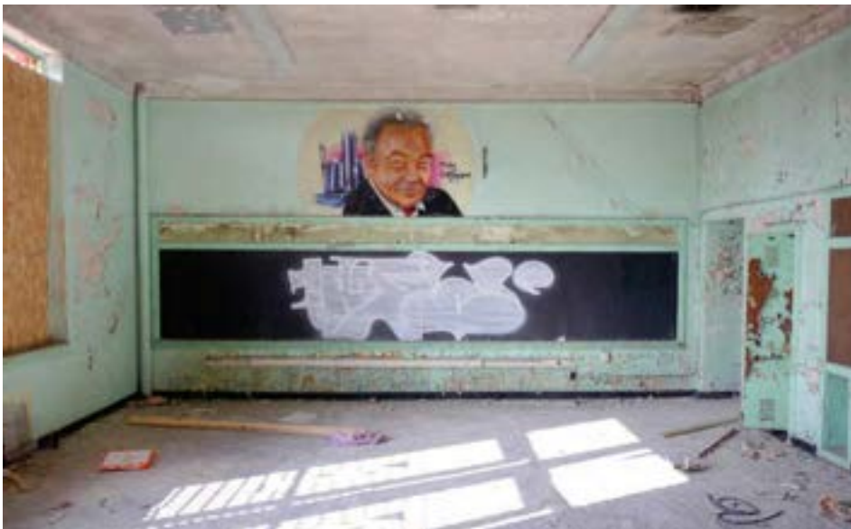
A typical classroom showing finishes in relatively good condition (and a smiling Coleman Young). Windows have been scrapped throughout much of the building.
