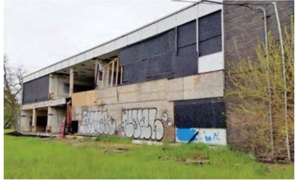
The 2-story east elevation of the original 1961 unit. This 2-story double-loaded bar houses about half of the school's standard classrooms. The facade originally featured a curtain wall with bands of glass and steel panels (see top right corner), but the system has been stripped away.
