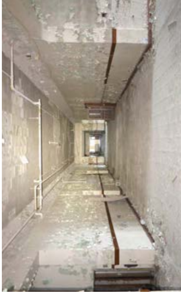
The main corridors in the original 1912 unit are extremely large, at 17' across and 13' high.
