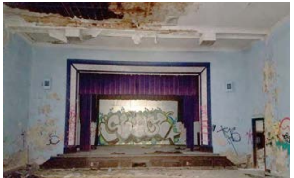
A view of the auditorium. A large section of the ceiling had collapsed due to water infiltration.
