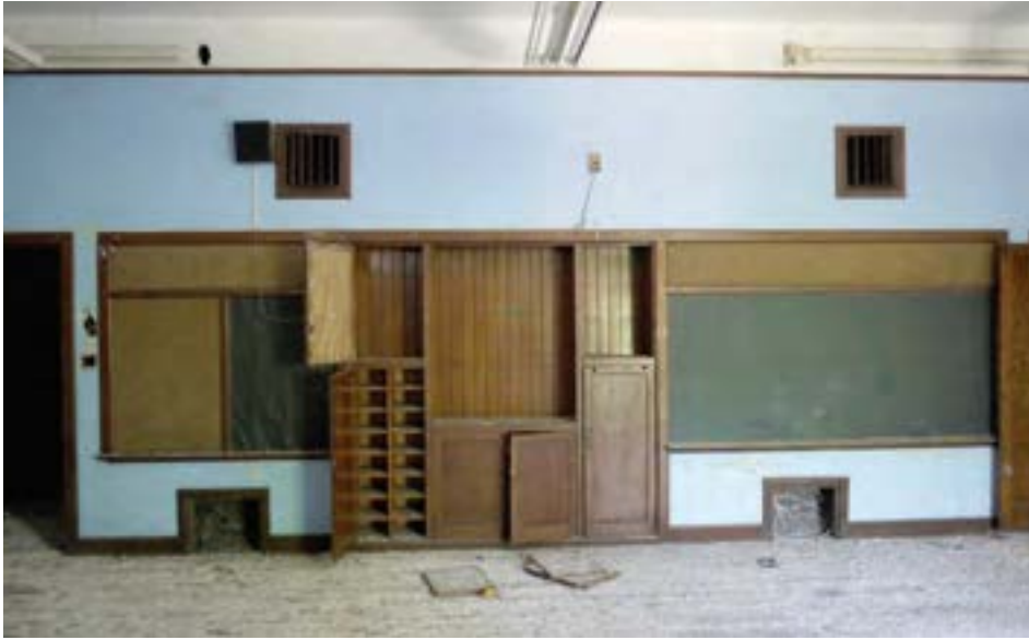
A typical classroom featuring built-in furniture and finishes in excellent condition. Although the school is open to trespass from the street, there is relatively little damage from vandalism, scrapping, and the elements.
