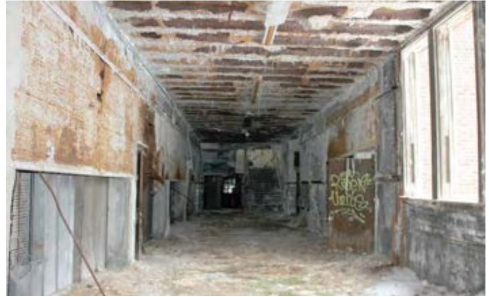
The first floor corridors are heavily water damaged and scrapped, with no original finishes intact.
