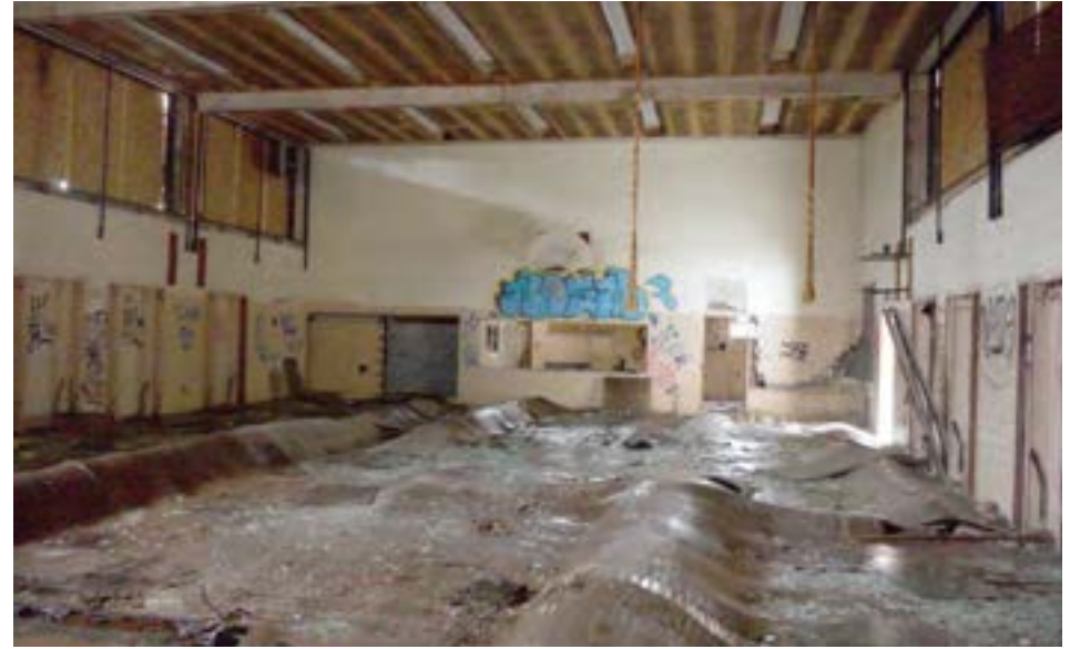
The combination gym and cafeteria is a 40x60' box that features large clerestory windows and 20' ceilings.
