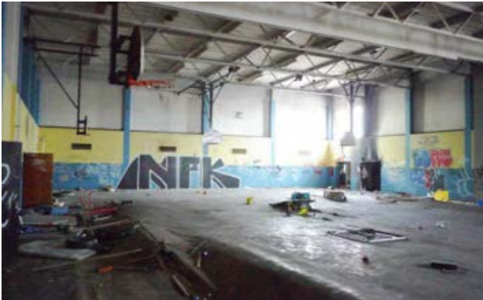
The 1963 gymnasium is a large steel-framed structure measuring approximately 70x100' with 27' ceilings. There are multiple auxiliary spaces attached, including locker rooms, gym offices, and storage areas. The gym complex is accessible from the street on the south end.
