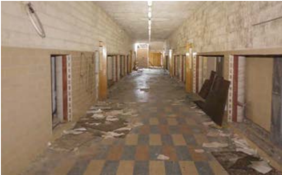
The main corridor on the first floor with lockers removed, but otherwise in good condition. Corridors are 12' wide and double-loaded.
