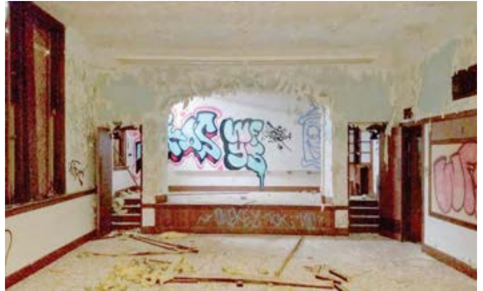
The 1930 addition included a classroom-sized mini-auditorium on the second floor, complete with a small raised stage.
