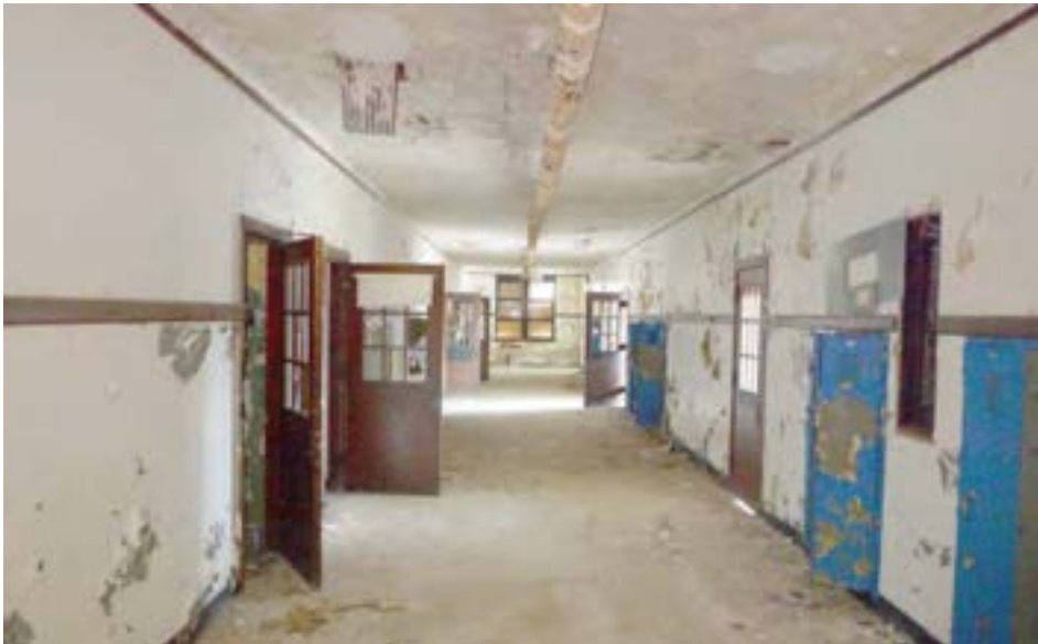
A corridor in the original 1925 wing, with plaster finishes and built-in lockers.
