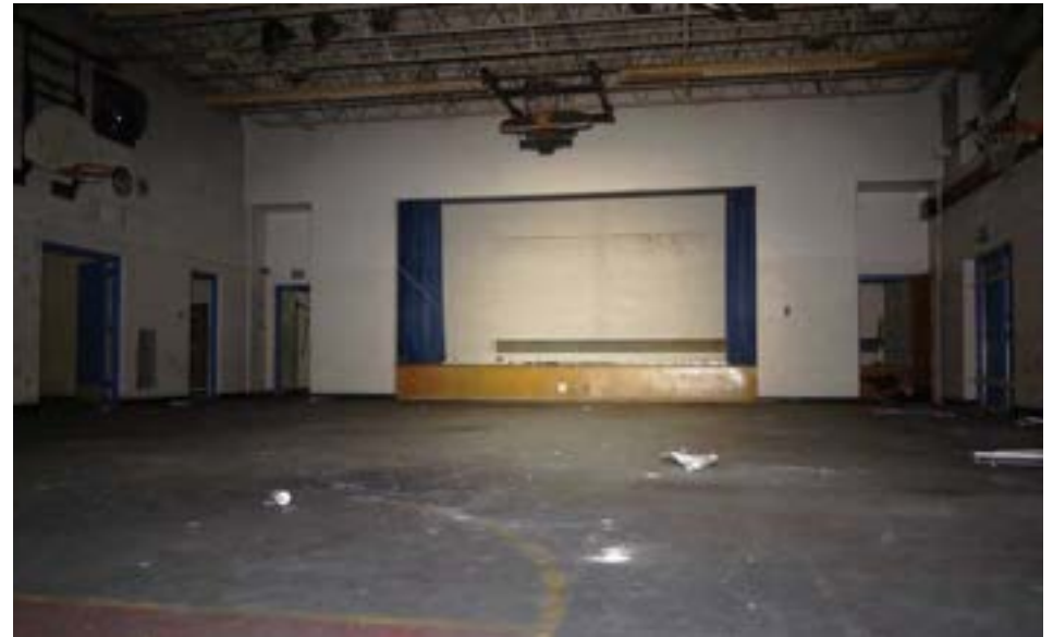
The large multipurpose room functions as a gym, auditorium, and cafeteria. The eastern wall has a row of small high windows to provide natural light, though these were boarded up during the visit.
