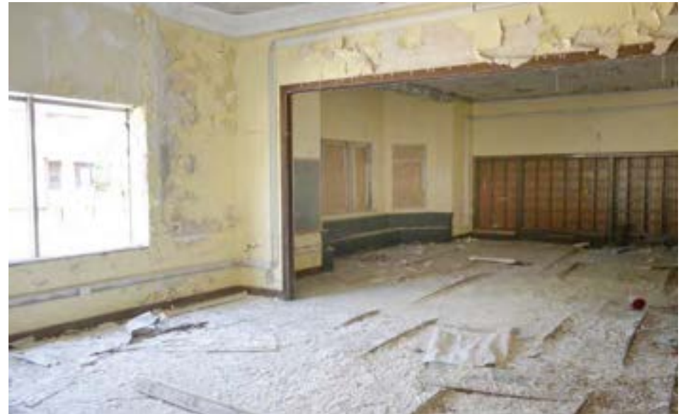
The kindergarten is a 2-room open-plan space featuring a shallow bay window and built-in wood shelving. The opposite end of the space (not visible above) features a plastered fireplace.
