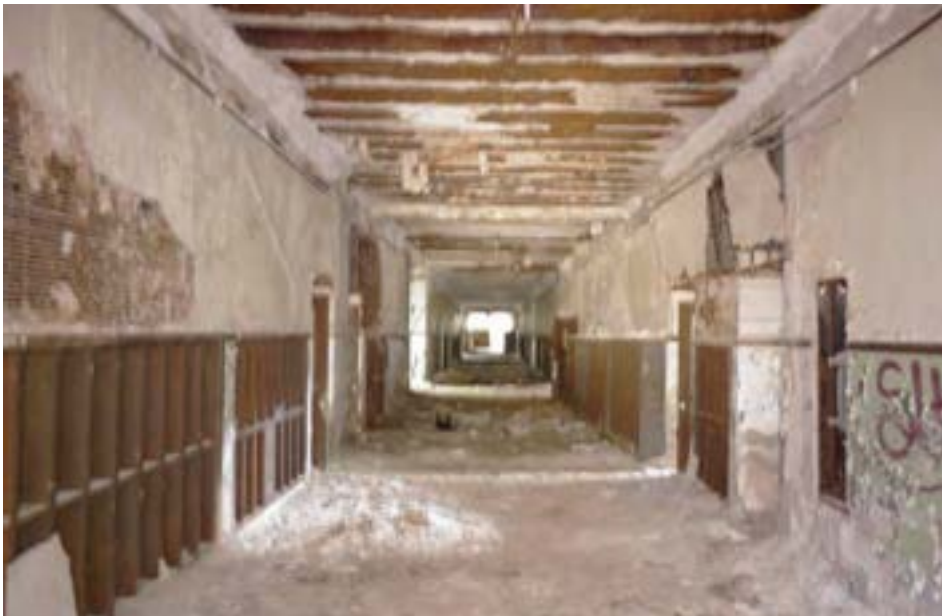
The first floor main corridor is heavily water damaged, causing plaster finishes to melt off the walls and ceiling.
