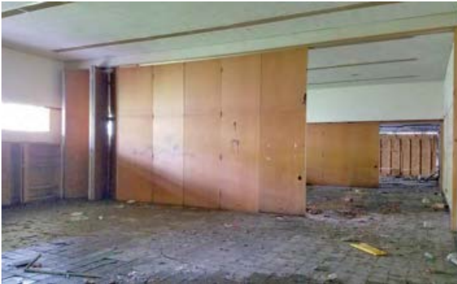
The multipurpose cafeterium is a unique space that can be reconfigured using two sets of wood folding panels. When both panels are open, the space extends seamlessly into the main entrance foyer; the main doors (boarded) are visible at the far end. Clerestory windows allow light from the courtyard.
