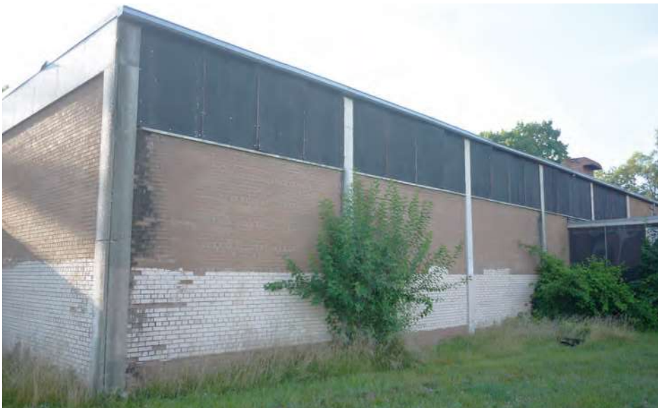
Gym exterior viewed from the northwest. Glass block clerestory has been boarded over but is intact. Some masonry distress is visible at the lefthand corner, likely due to water infiltration from roofing membrane deterioration around perimeter of gym.
