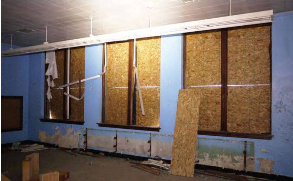
Window configuration and finishes in typical 1925 classroom. Original wood frame windows and their metal replacements are gone; radiators have also been scrapped.
