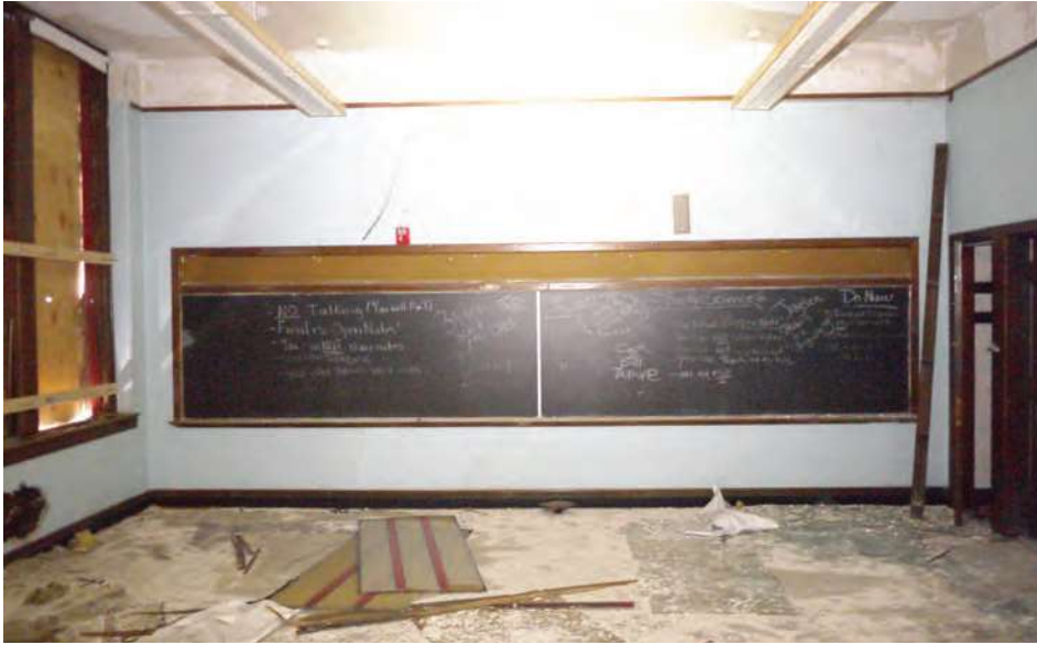
A typical classroom in the original unit, with plaster and wood finishes in relatively good condition. Metal replacement windows have been scrapped.
