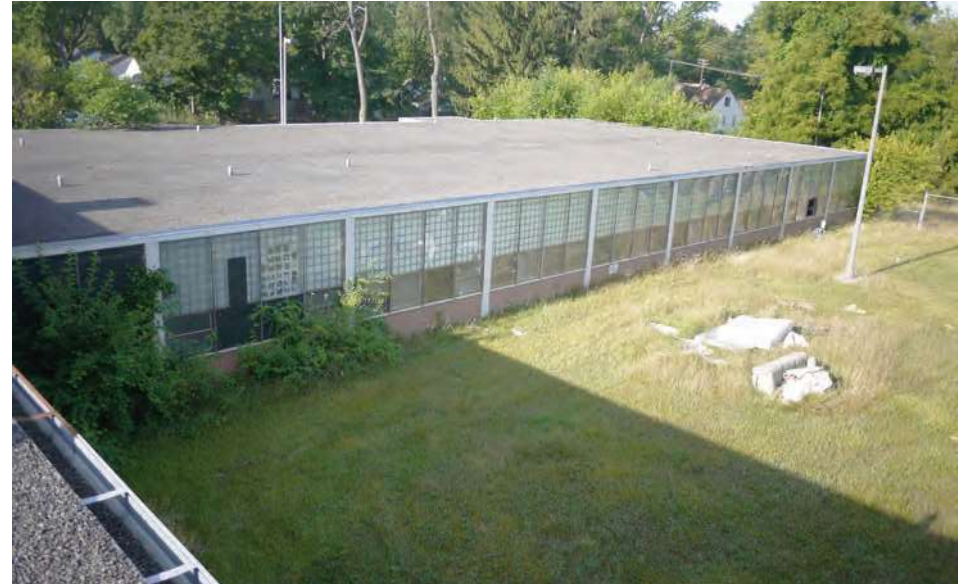
North elevation viewed from gymnasium roof. Original window scheme is clearly visible here. Windows are mostly intact and in repairable condition, though some glass panes have been replaced by plexiglass.
