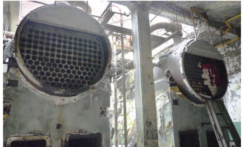
Two massive boilers sit in the pit-like 1930 boiler room. The boiler room is built partly above grade and has an open roof.
