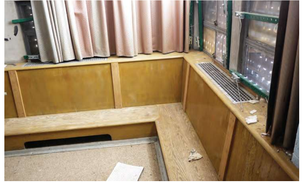
The original wood bench in the kindergarten’s bay window is intact and in good condition.
