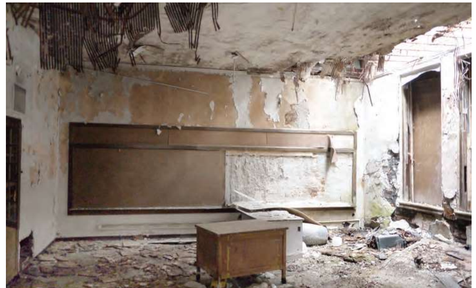
An original 1925 classroom with water damage and partly missing roof. The school building has extensive damage from water infiltration, as well as scrapping and minor fires.
