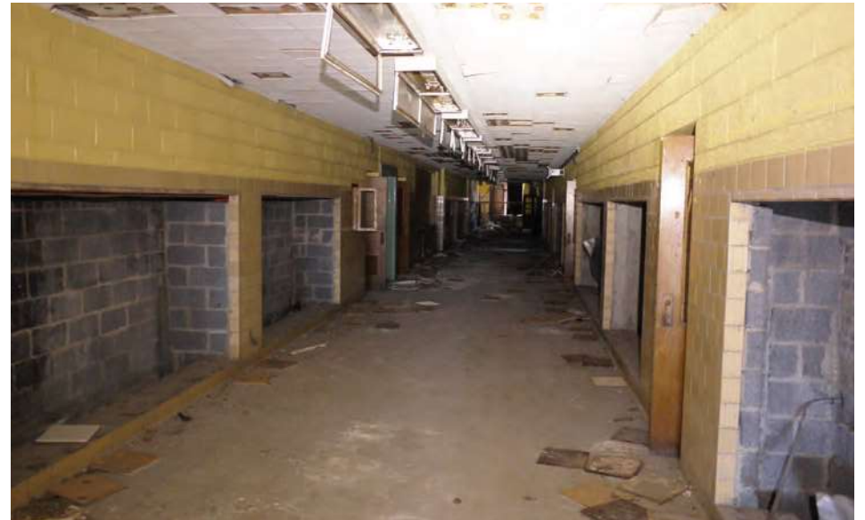
Typical corridor in 1959 addition. Lockers and ductwork have been scrapped, but otherwise the corridor is clean and in serviceable condition.
