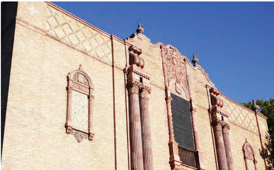
Decorative tile and terra cotta elements on the southeast corner of the original school building.
