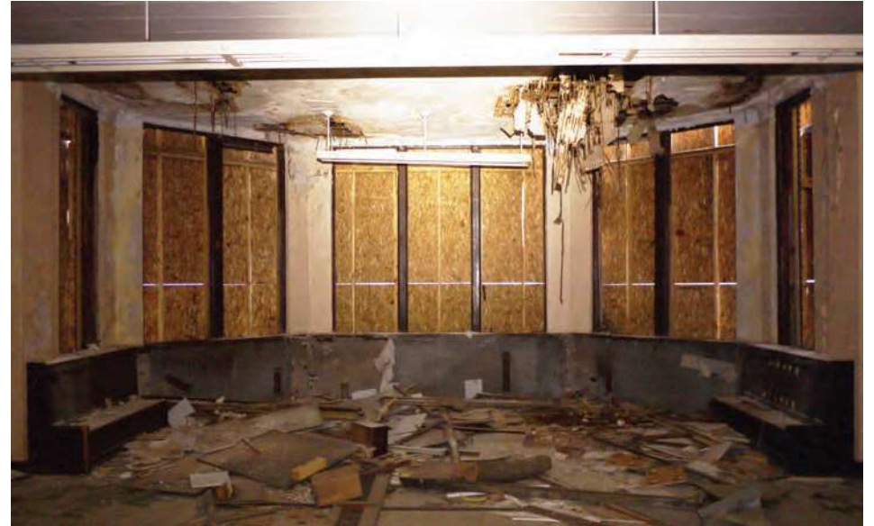
Kindergarten bay window in original 1925 unit. Windows, original wood benches, and radiators have been removed. Water infiltration at the protruding roof has caused plaster failure.
