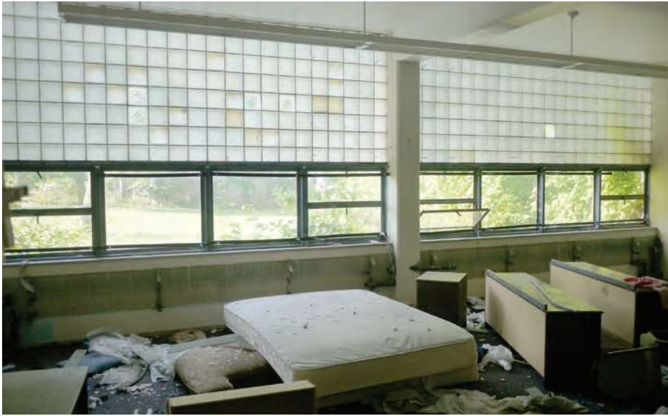
Classrooms feature large windows with glass block bands over steel frame operable lites. Most of the windows are in repairable condition.
