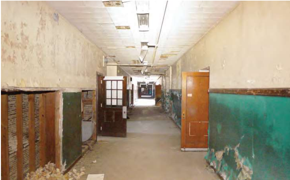
The long, west corridor, part of the original 1925 building. Lockers have been scrapped, but the plaster finishes are in relatively good condition.
