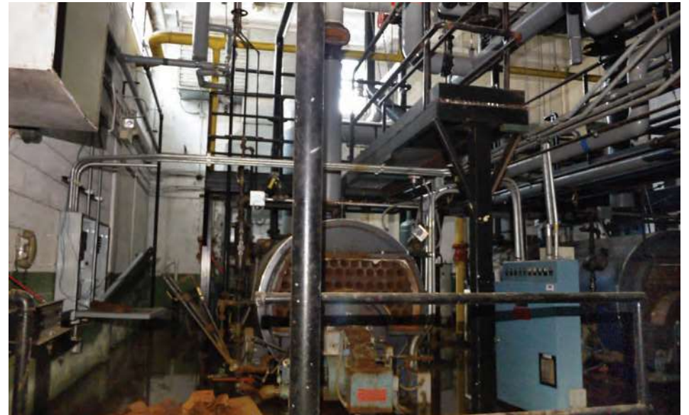
The school features an attached boiler room accessible from the main hallway. The space is a naturally-lit sunken cube, measuring almost 30 feet in all directions.
