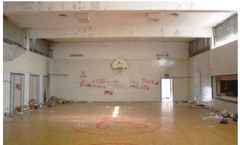
The combination gym/cafeteria is in mostly good condition, though water infiltration and distress is noted at the ends of the roof beams and ceiling perimeter, where roof membrane has deteriorated. The kitchen and serving window are visible to the right.
