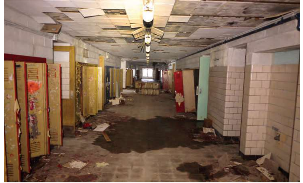
The main (north) corridor in the 1955 unit is 12' wide, but has only 8' ceilings—lower than at other historic schools. Water infiltration was observed throughout all corridors.
