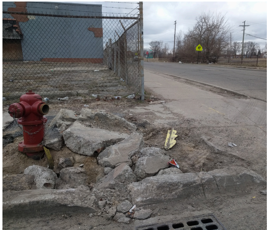
The intersection of Saint Aubin and Brewster Streets at Kap's Wholesale is too tight for large trucks, resulting in sidewalk damage. Photo: BuroHappold Engineering
