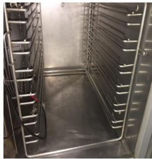
Interior of Blast Chiller
