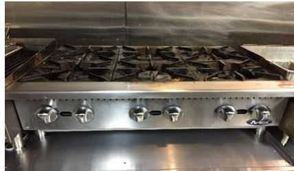
Equipment Elevated 4" Above Counter
