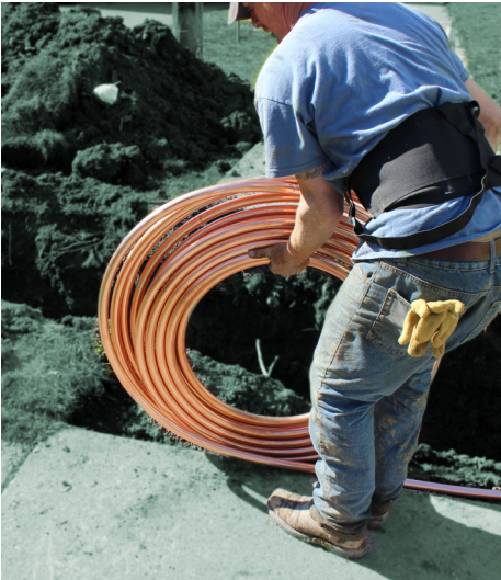
In 2018, DWSD started a Lead Service Line Replacement Program as part of its water main replacement projects.
