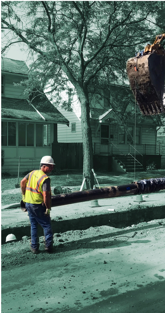
DWSD replaced the water main on Robson Street north of Grand River Avenue.
