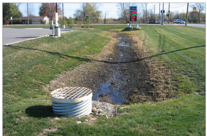
Detention basin with outlet riser in the forefront of the photo
