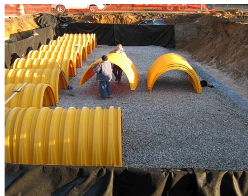
Subsurface Detention Storage
