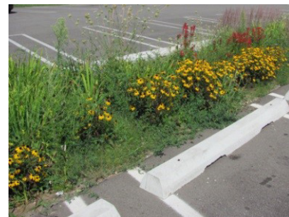
Bioretention between Parking Lot Aisles
