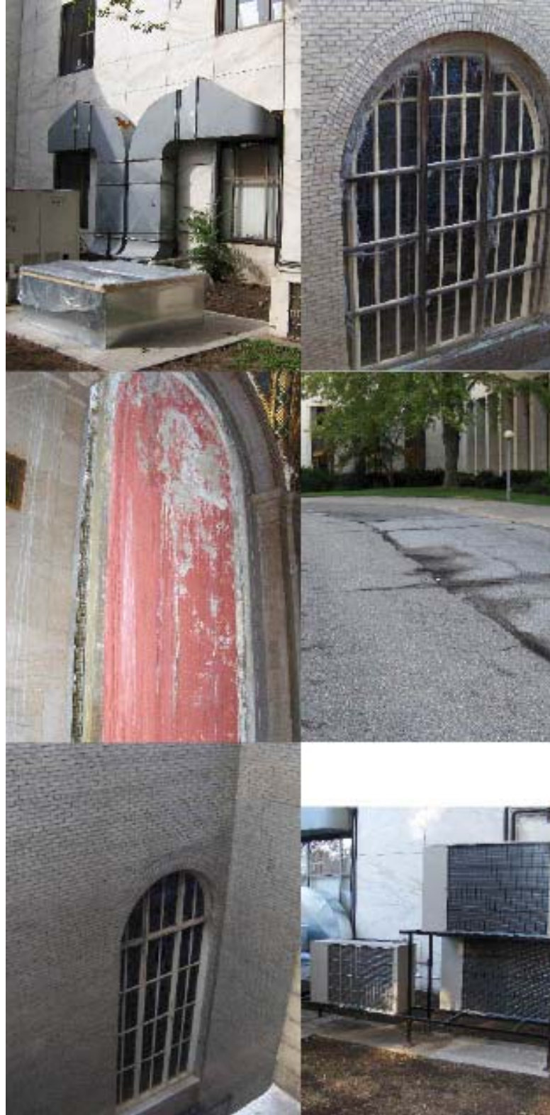
Structural Damage/Needs at the Main Library
