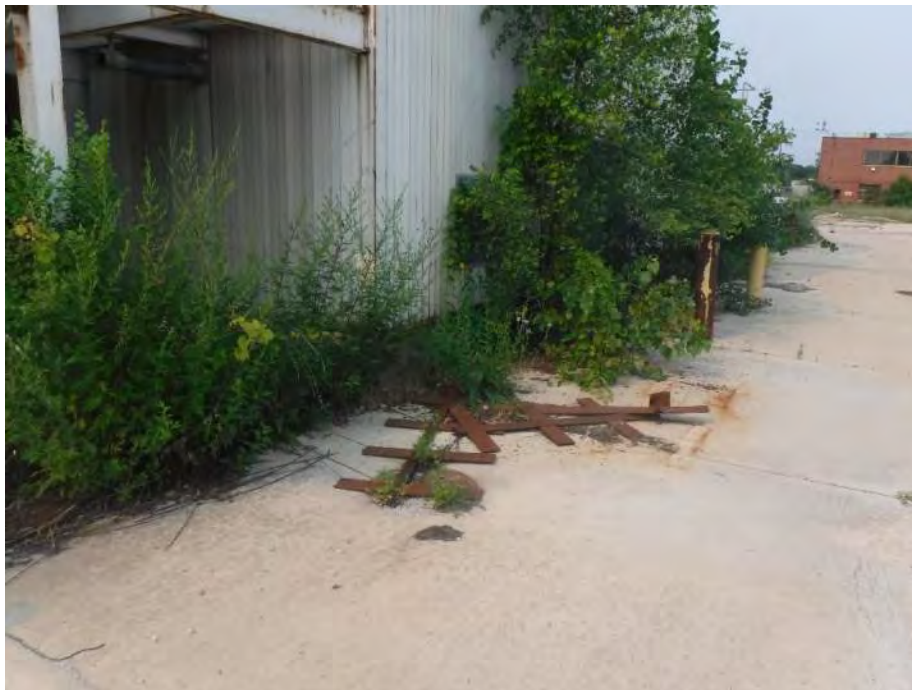
Photo 40: Looking southwest at the northern portion of the Gas House portion of the Main Building. Gasoline odors were noted in the storm sewer catch basin in the bottom central portion of the photo, beneath the scrap steel.
