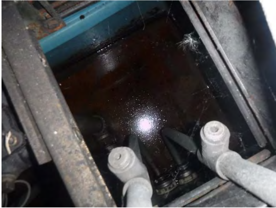
Photo 23: Looking southwest (and downward) beneath the gasoline dispenser in the southern portion of the gas house. Unknown fluids were present within the dispenser sump at this location.
