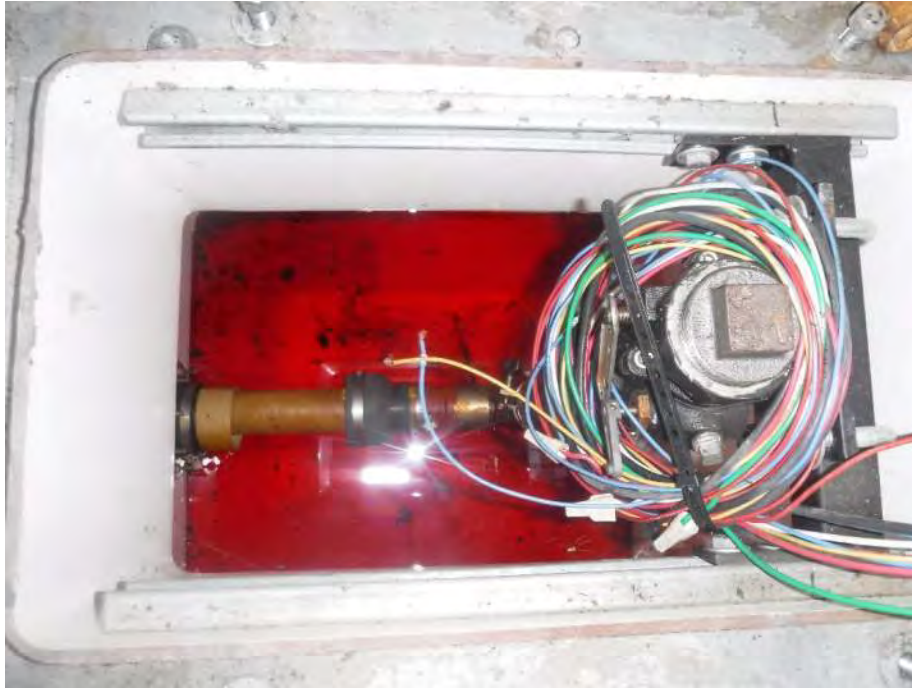
Photo 19: Looking south (and downward) beneath one of the five removed diesel fuel dispensers. Apparent dyed diesel fuel was observed in the dispenser sump at this location.
