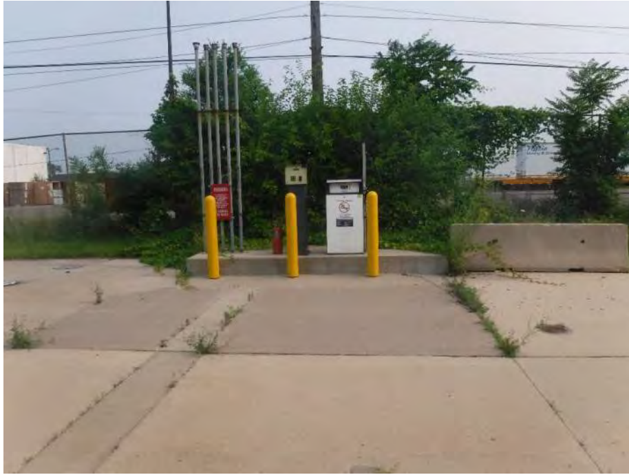
Photo 15: Looking north at a gasoline dispenser near the 12,000-gallon gasoline underground storage tank (UST) located north of the Main Building. A 10,000 to 12,000-gallon gasoline UST is located in this area. Historical records are conflicting whether this tank is actually 10,000 or 12,000-gallon capacity.
