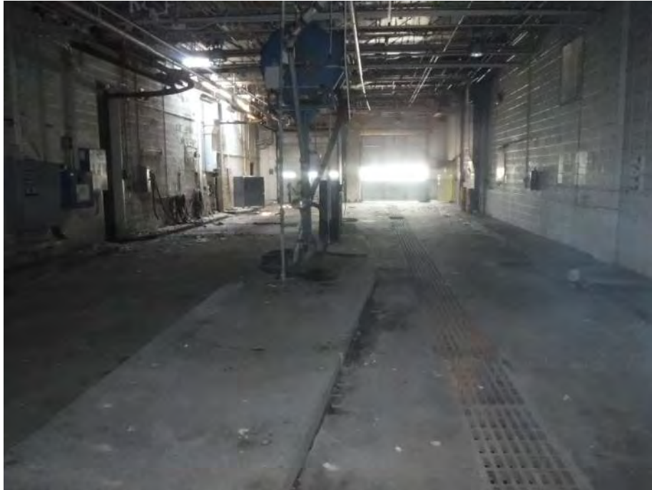
Photo 21: Looking west at the southern portion of the gas house which contained the gasoline fueling area. A hydraulic lift was also present within this area (at grade in left bay).
