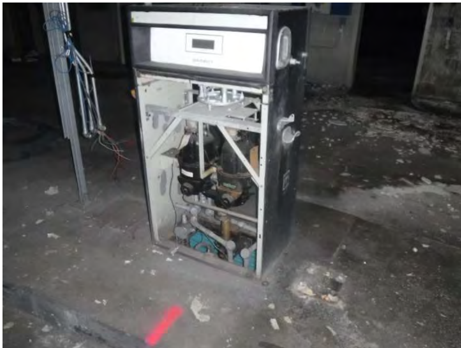
Photo 22: Looking southeast at a gasoline dispenser in the southern portion of the gas house.
