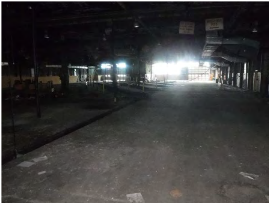
Photo 24: Looking east at open trenches in the maintenance area of the Main Building. Grating which formerly covered the trenches had been removed in several areas.
