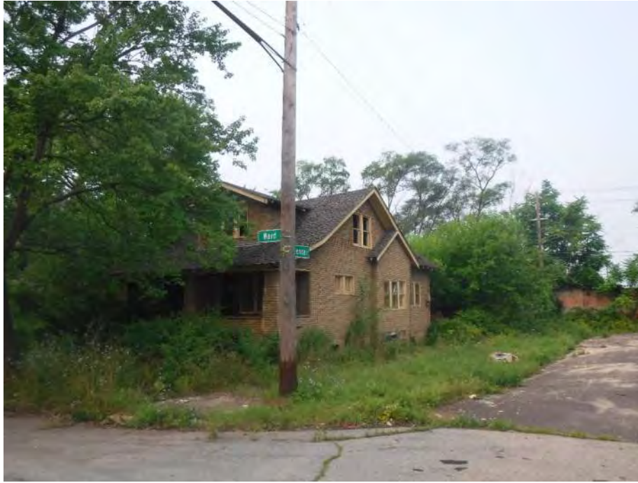
Photo 9: Looking southwest at a vacant dwelling located at 14045 Ward Avenue in the eastern portion of the Subject Property. The west end of Kendall Street where it meets the bus terminal property is seen at right.
