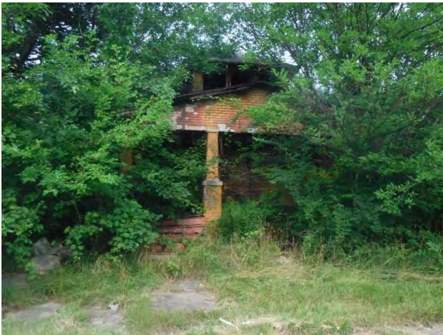
Photo 12: Looking west at an abandoned residential dwelling located at 14151 Ward Avenue in the eastern portion of the Subject Property. Fire damage was evident within the structure and it appeared unsafe to enter.
