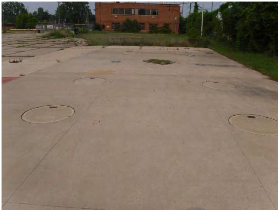
Photo 16: Looking west at the access covers above the diesel underground storage tanks (USTs). Four 25,000-gallon diesel USTs installed in 2001 are located in this area.
