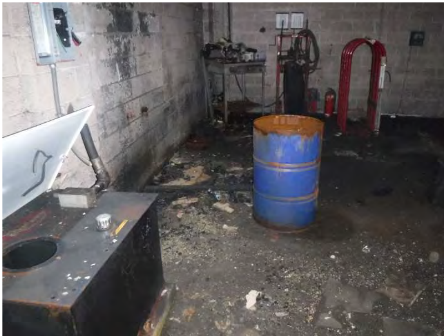
Photo 28: Looking northeast at a hydraulic fluid reservoir (far left) and deteriorated 55-gallon steel drum located between the maintenance area and gas house in the northern portion of the Main Building. The roof was deteriorated in this area which allowed water to infiltrate.
