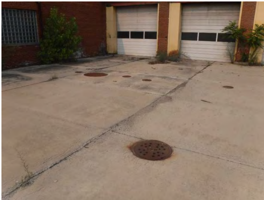
Photo 34: Looking southwest at an in-ground oil water separator to the east of the bus wash portion of the gas house, which is located in the northern portion of the Main Building.
