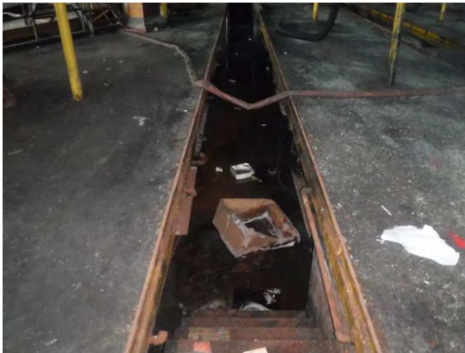
Photo 30: Looking northeast at a trench within the maintenance area of the Main Building, which was formerly used to access the underside of buses during maintenance such as oil changes. Oily water was observed within this and several other trenches in the vicinity.
