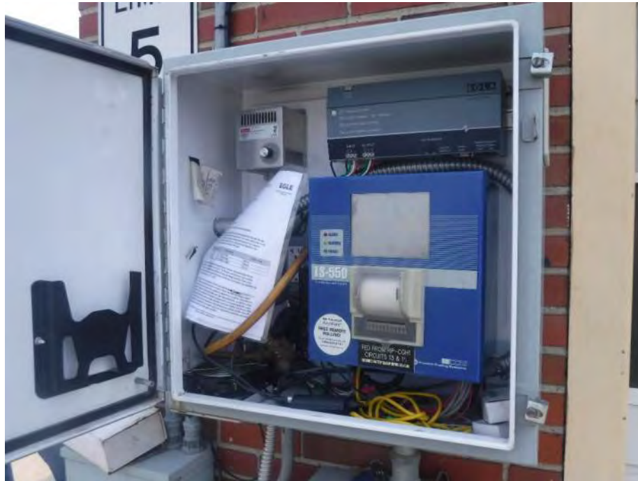
Photo 17: Looking northeast at the automatic tank gauge which serves the nearby underground storage tanks. Clean Fuel Solutions personnel were present onsite during the site reconnaissance and indicated the diesel USTs are constructed of steel with no cathodic protection system.
