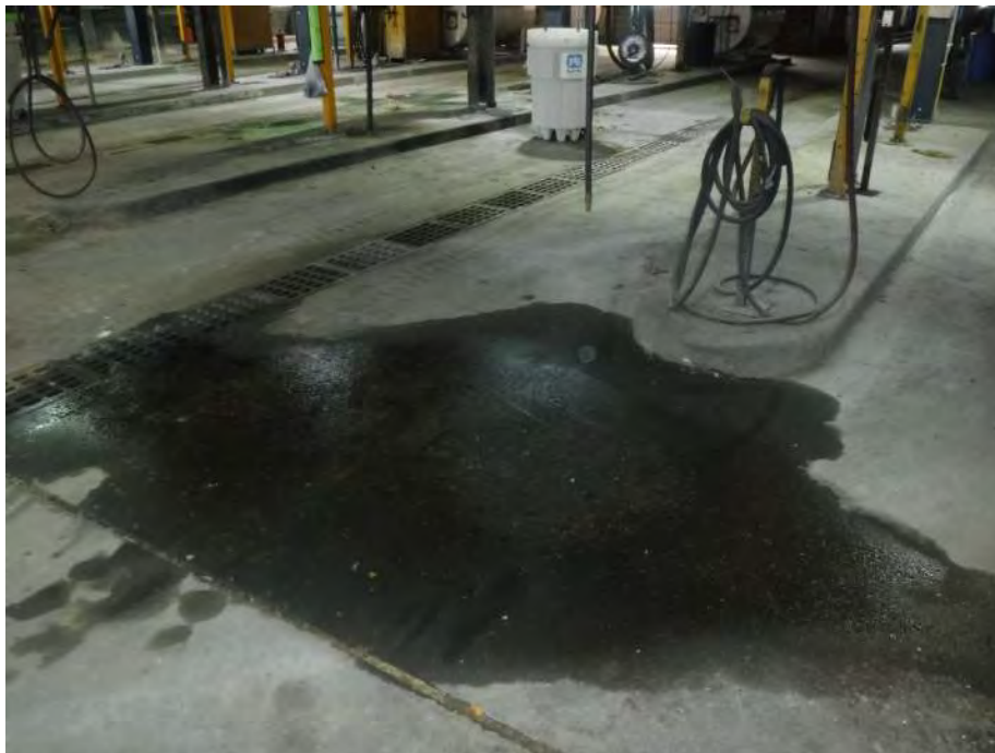
Photo 20: Looking northeast at an oil stain in the southwest portion of the gas house. The oil had migrated into a nearby crack in the concrete as well as trenches in the area.
