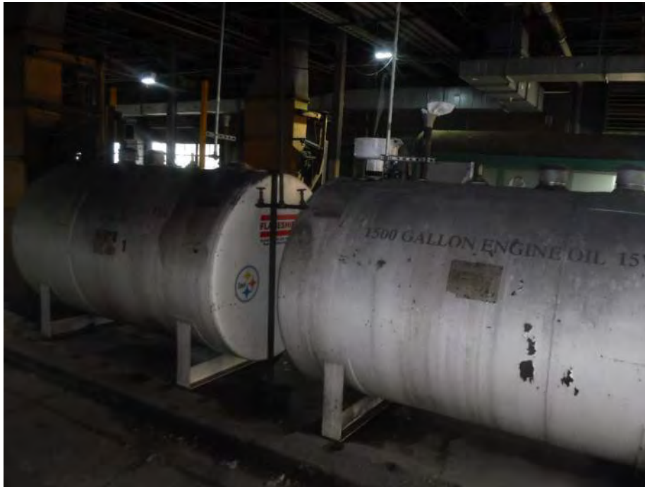
Photo 32: Looking southeast at engine oil aboveground storage tanks located in the gas house portion of the main Building. De minimus staining of the surrounding concrete floor was observed in this area.
