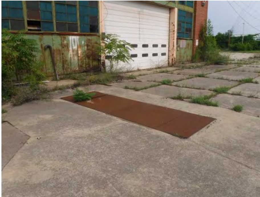
Photo 35: Looking northwest at an in-ground oil water separator located east of the maintenance area portion of the Main Building. The metal cover was welded in-place which prohibited further assessment.
